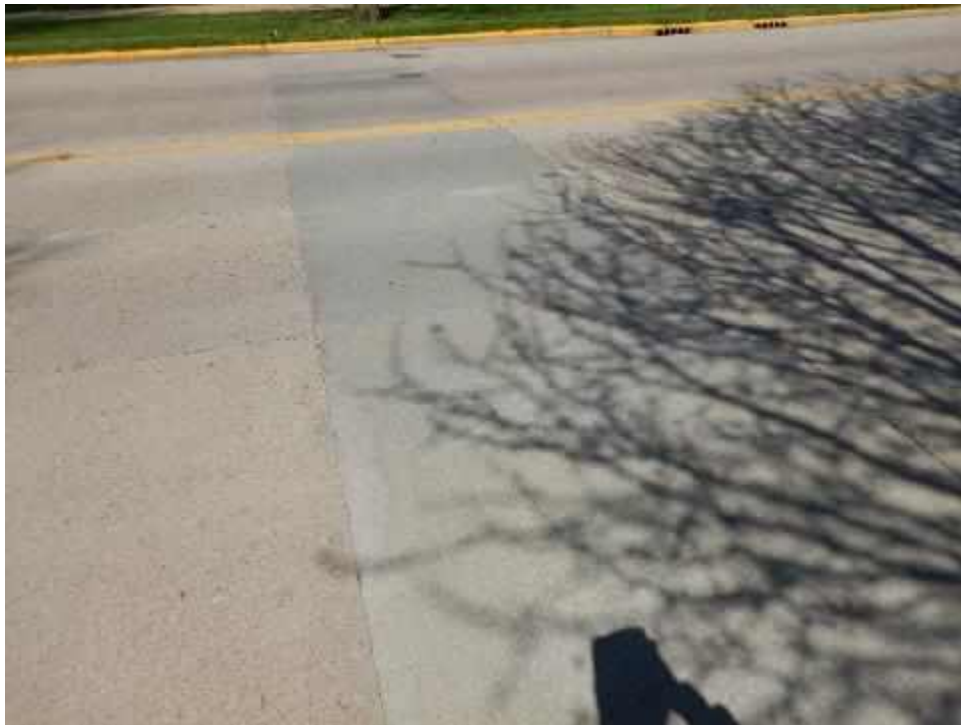
LNCLNAV-US19-Large Patching-(Sample Unit No. 01)
