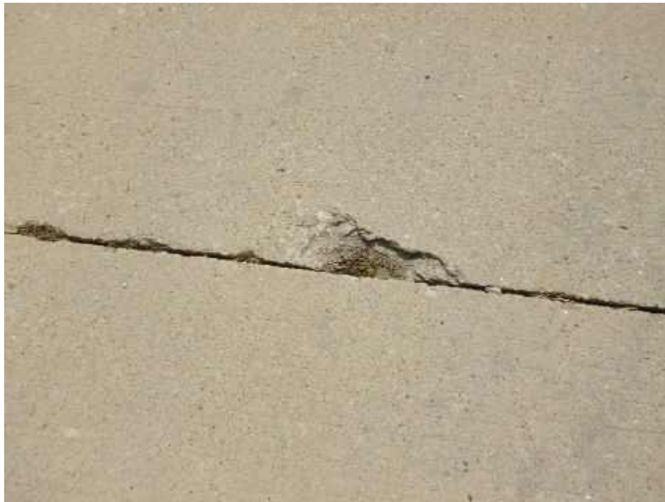
VRGNADR-US14BE-Joint Spalling-(Sample Unit No. 01)
