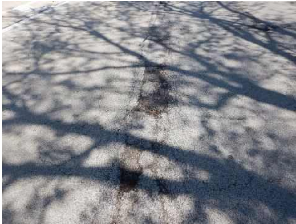
LNCLNAV-US17B-Joint Reflection Cracking-(Sample Unit No - 72)
