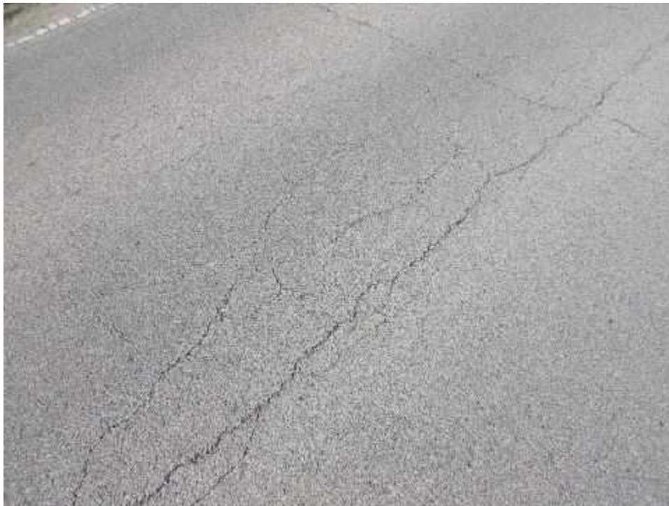
STMARR-UW12-Alligator Cracking-(Sample Unit No. 01)
