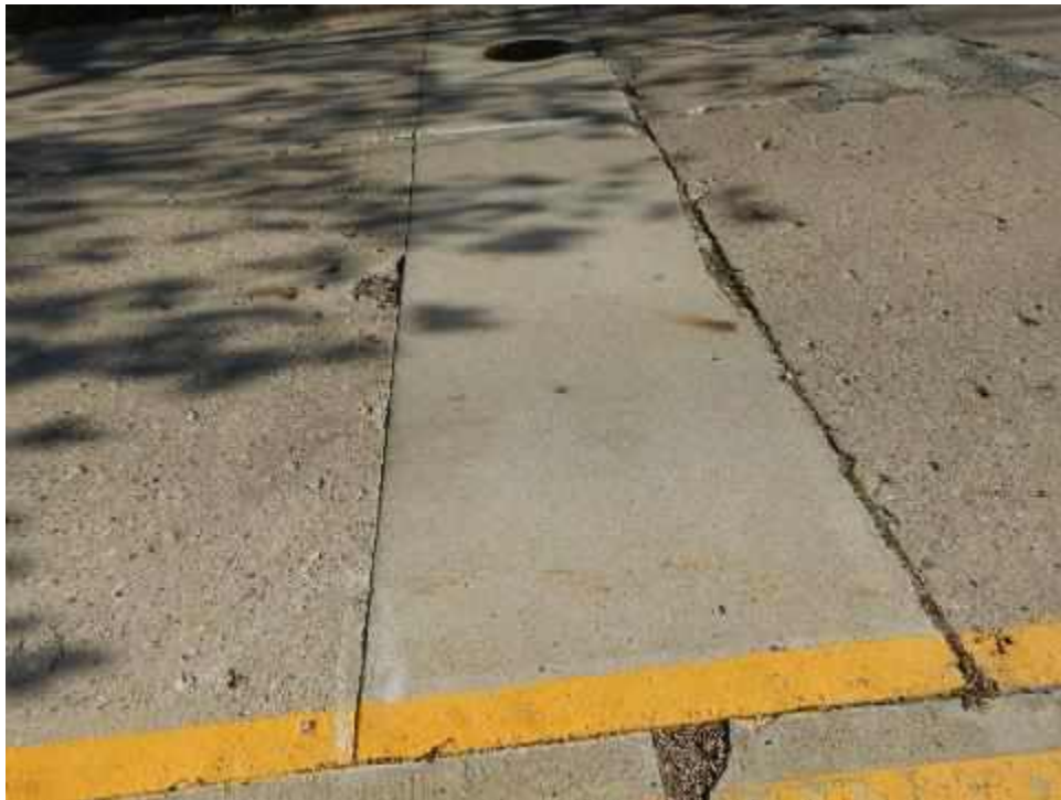
STMARR-E00B-Large Patching-(Sample Unit No. 01)
