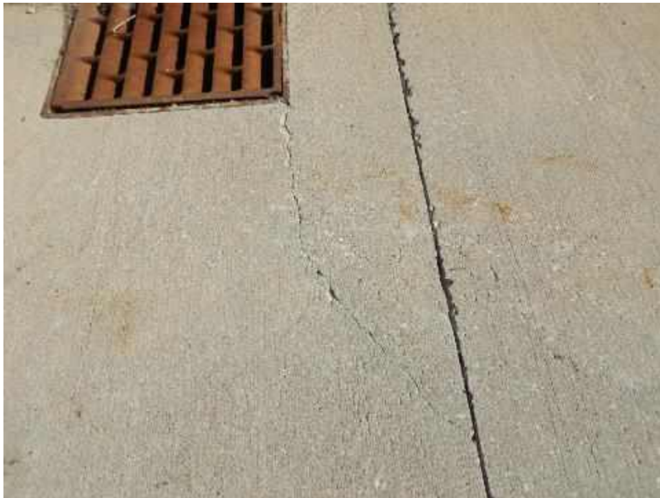
GERTYD-E00C-LTD Cracking-(Sample Unit No. 01)
