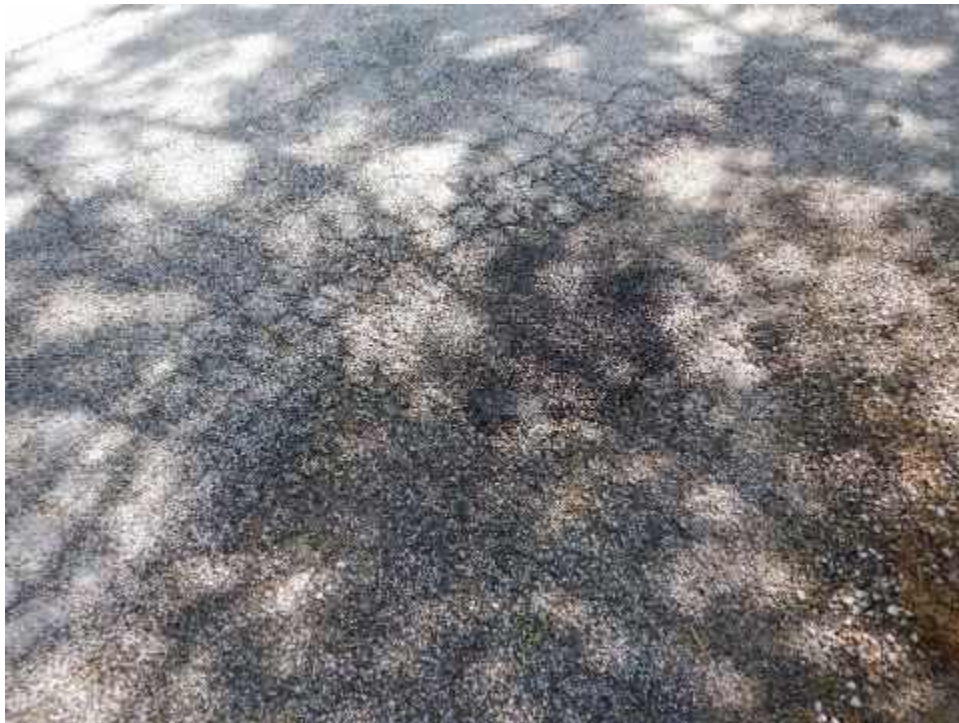
HAZELWDD-E00A-Alligator Cracking-(Sample Unit No. 01)
