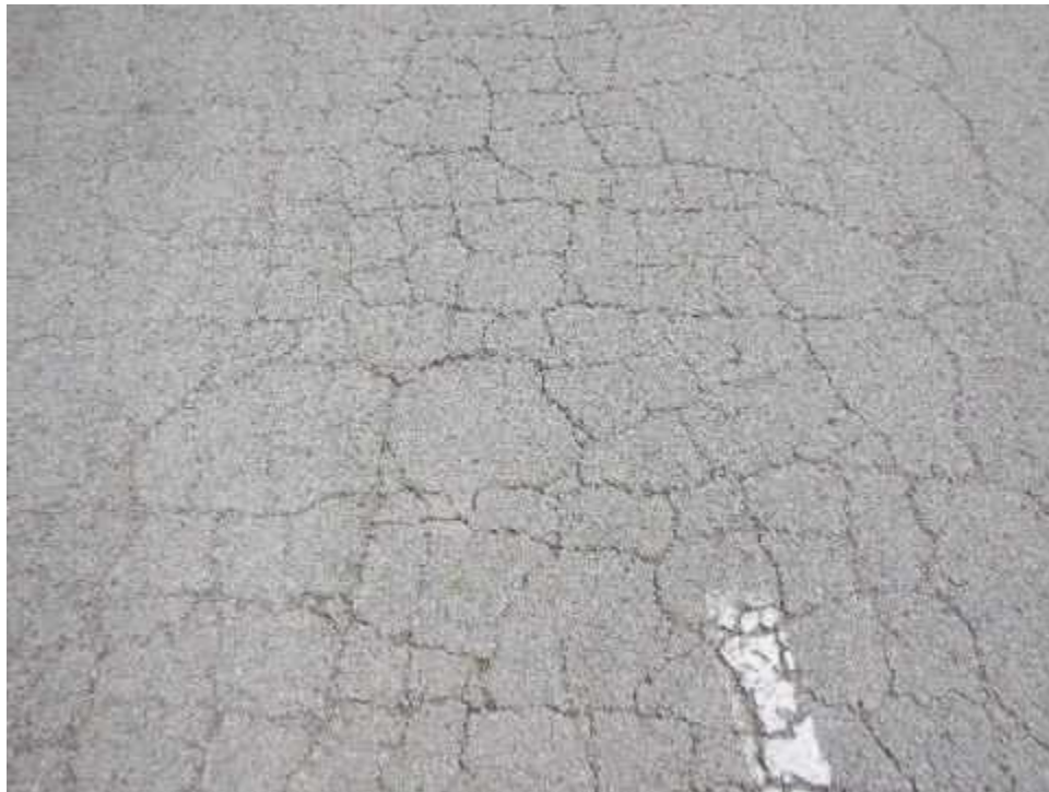
COLAGCT-UW09AN-Alligator Cracking-(Sample Unit No. 01)
