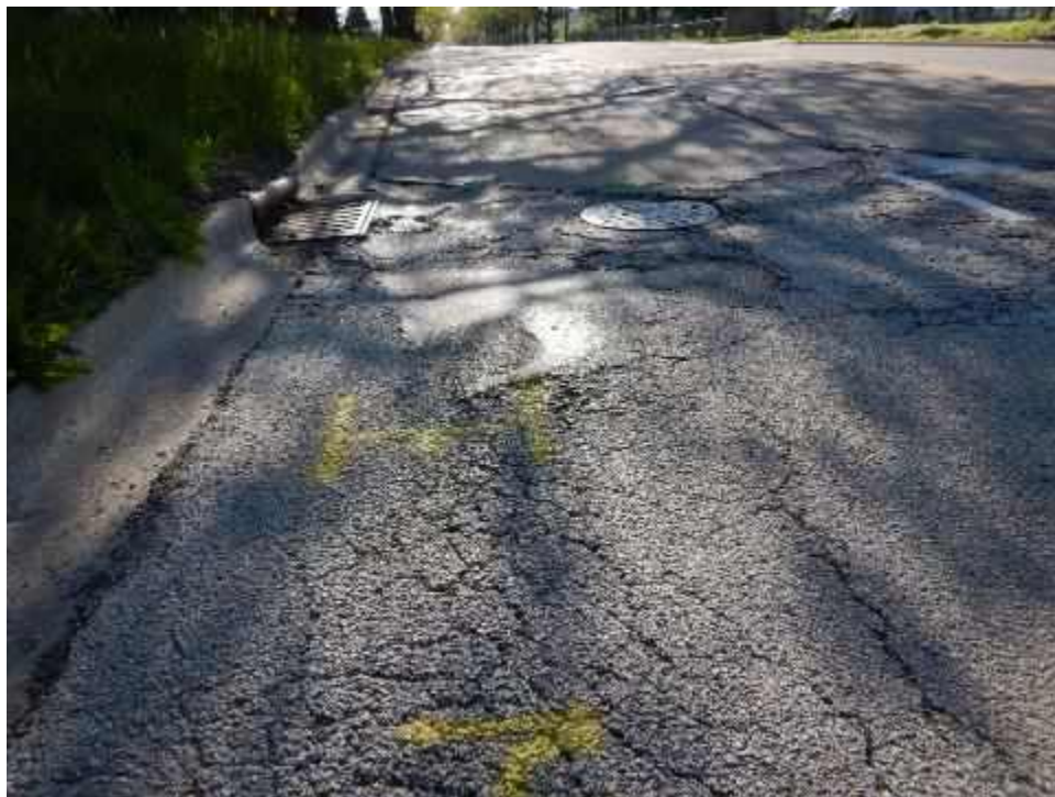
STMARR-E00A-Patching-(Sample Unit No. 01)
