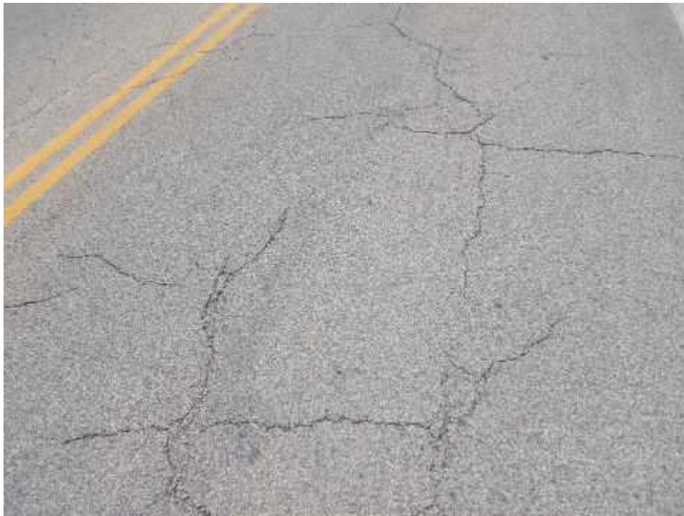
GREGYD-UW11-Block Cracking-(Sample Unit No. 01)
