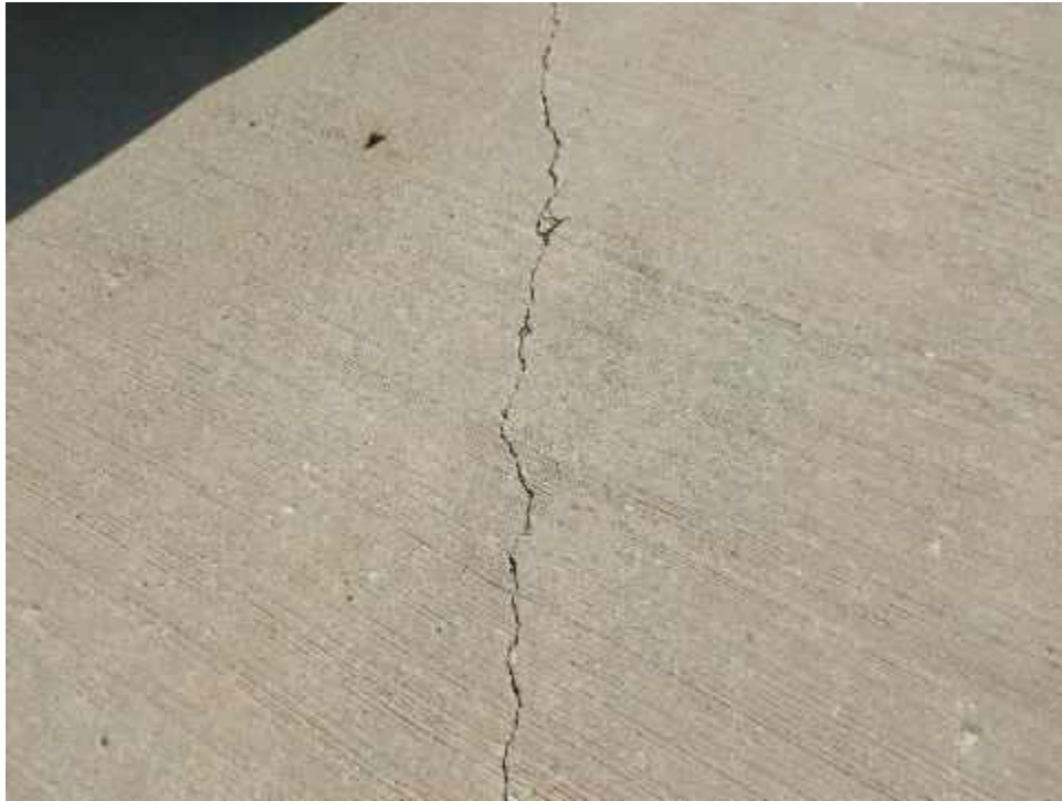
HAZELWDD-E01B-LTD Cracking-(Sample Unit No. 01)
