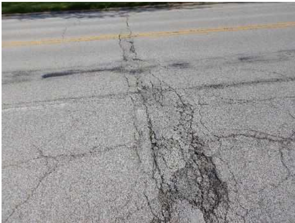
STMARR-E01-Joint Reflection Cracking-(Sample Unit No - 71)
