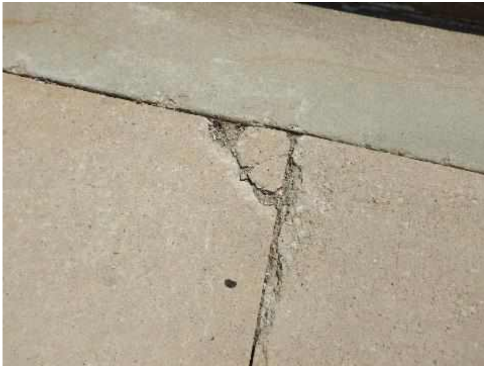
ARMRYA-E05-Corner Spalling-(Sample Unit No. 01)
