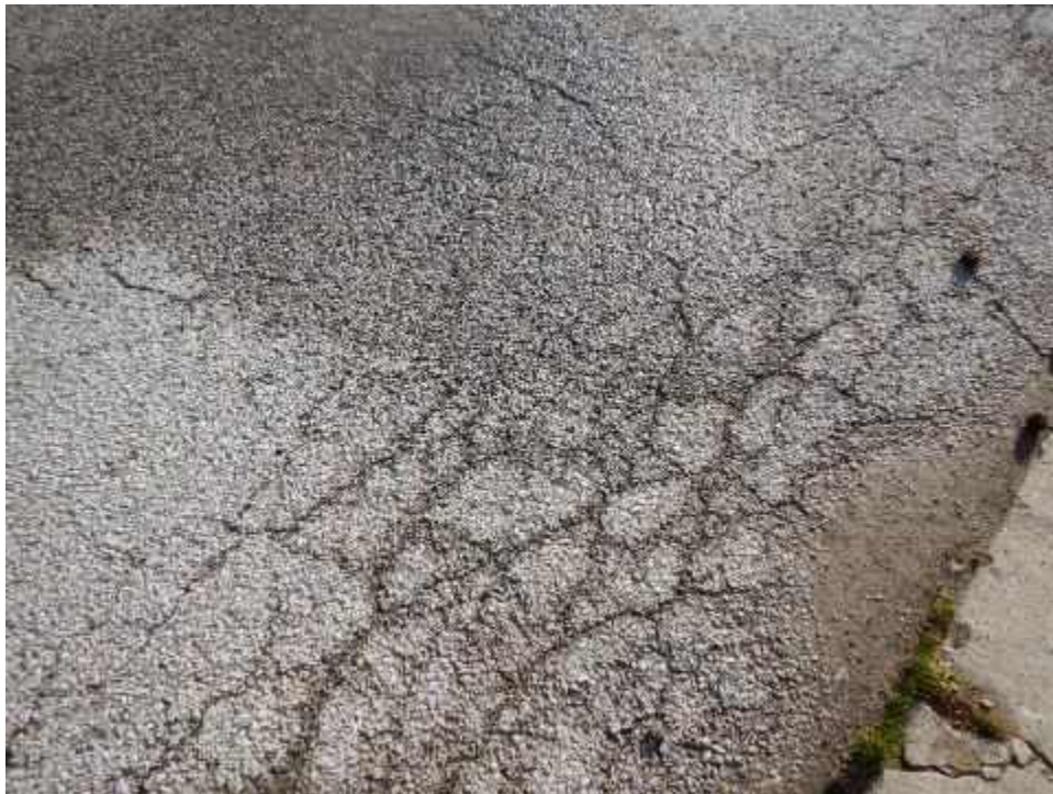
BAILEYD-E00-Alligator Cracking-(Sample Unit No. 01)
