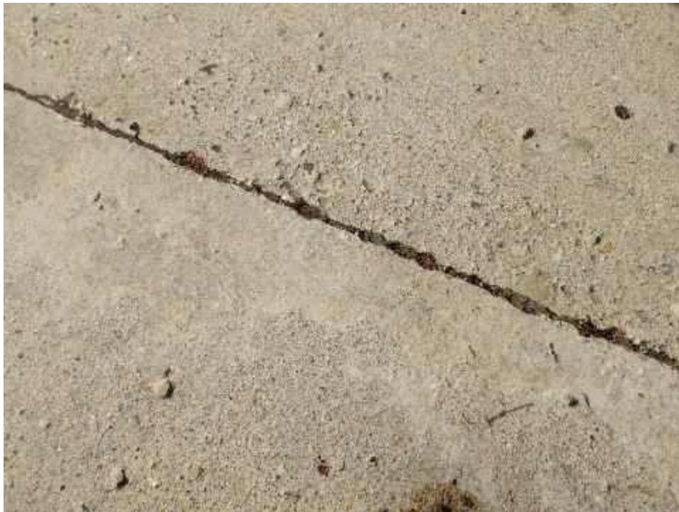
GERTYD-E00B-Joint Seal Damage
