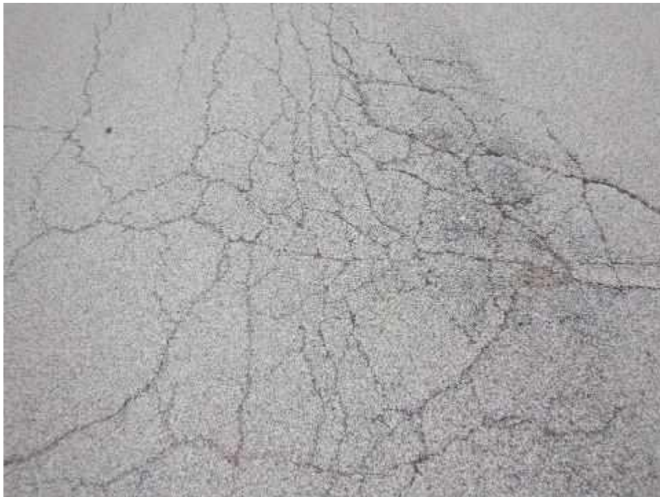
LORADOTD-UW12-Alligator Cracking-(Sample Unit No. 01)
