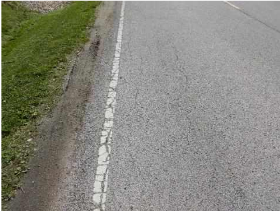
STMARR-UW09A-Alligator Cracking-(Sample Unit No. 01)
