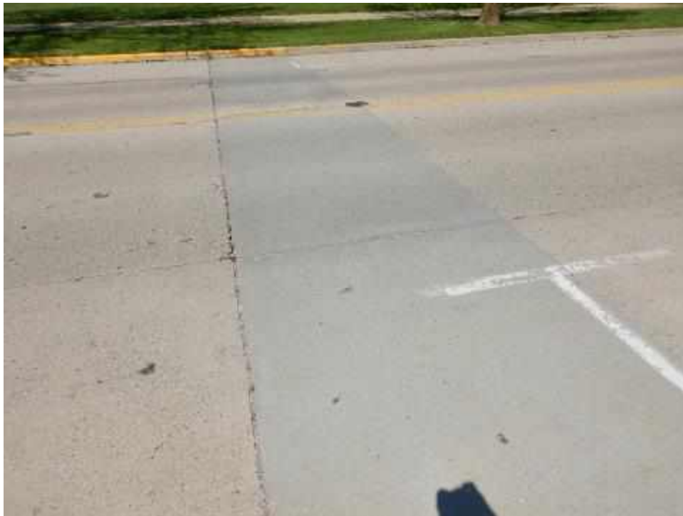
LNCLNAV-US17A-Large Patching-(Sample Unit No. 01)
