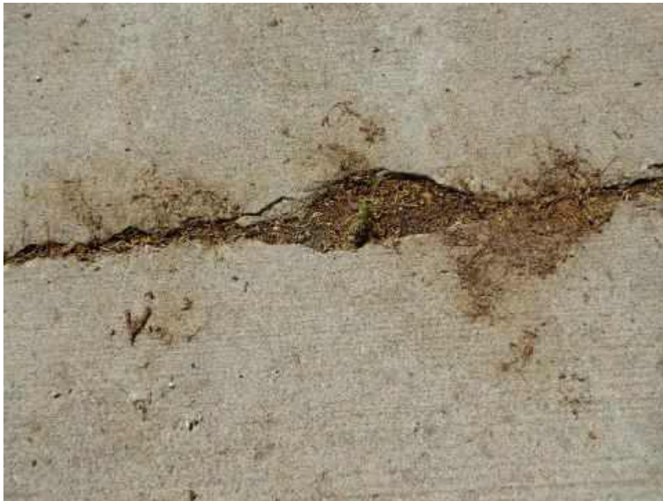
STADMD-E00D-Joint Spalling-(Sample Unit No. 02)
