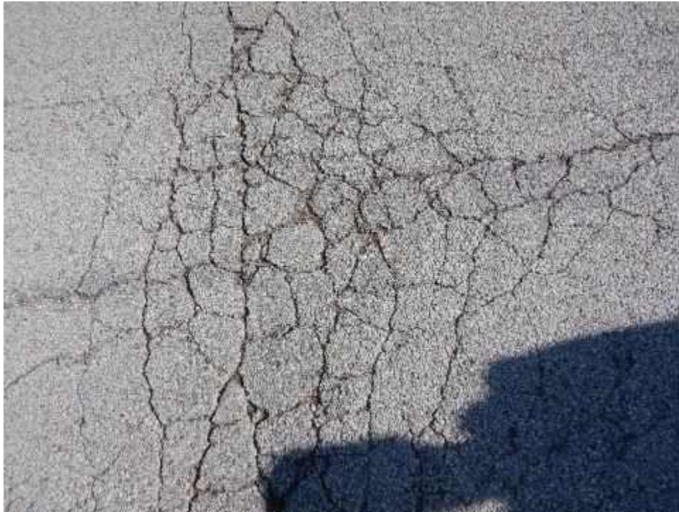
STMARR-E00D-Alligator Cracking-(Sample Unit No. 01)
