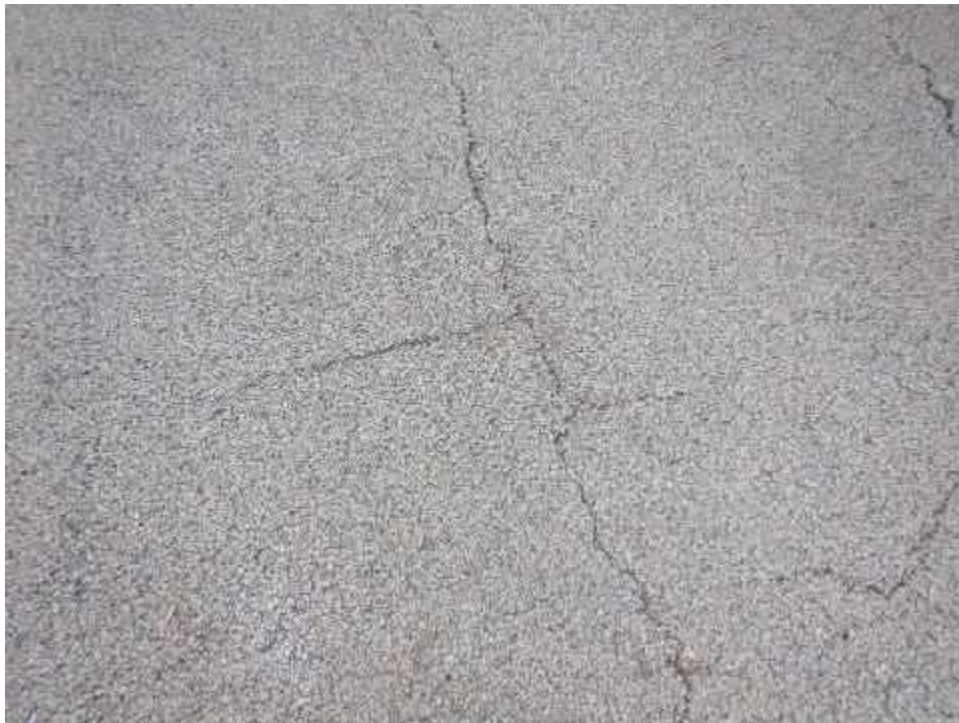
MAINS-UW11B-L&T Cracking-(Sample Unit No. 01)
