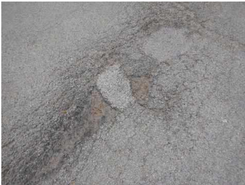
PENSYA-UW09B-Alligator Cracking-(Sample Unit No. 01)
