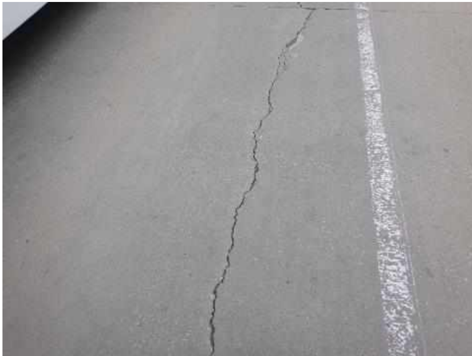
GREGYD-UW12B-LTD Cracking-(Sample Unit No. 01)
