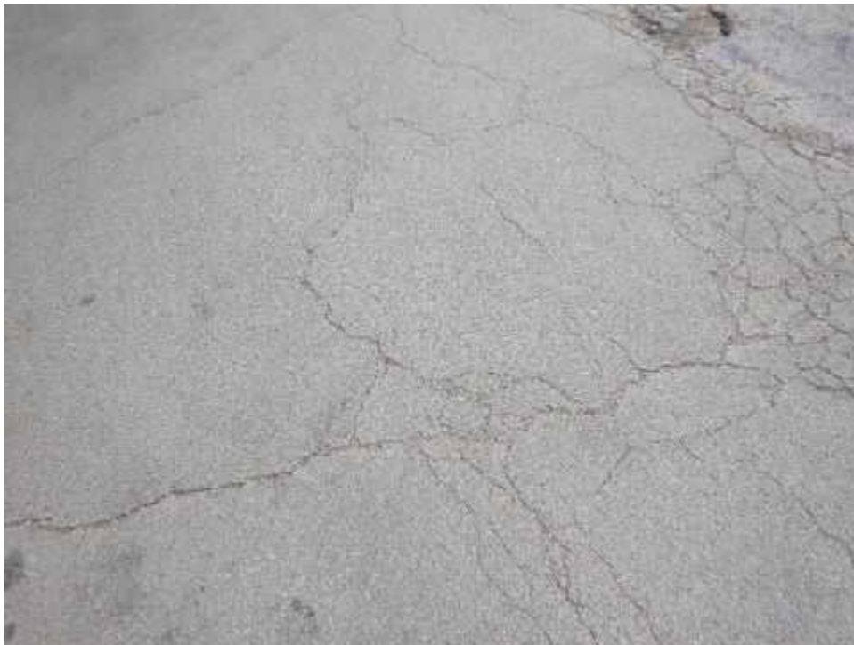
PENSYA-UW11A-Block Cracking-(Sample Unit No. 01)
