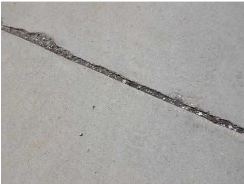
OAKS-S10C-Joint Seal Damage-(Sample Unit No. 01)
