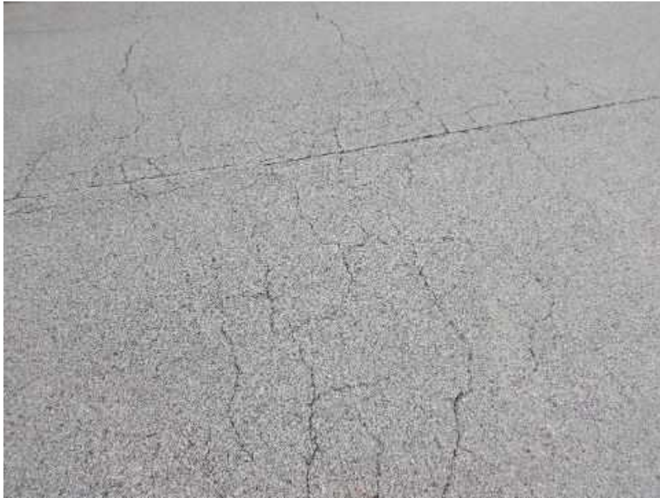
HAZELWDD-E00B-Alligator Cracking-(Sample Unit No. 01)
