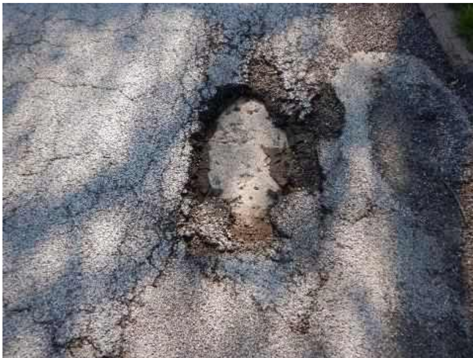
STMARR-E00C-Pothole-(Sample Unit No. 01)
