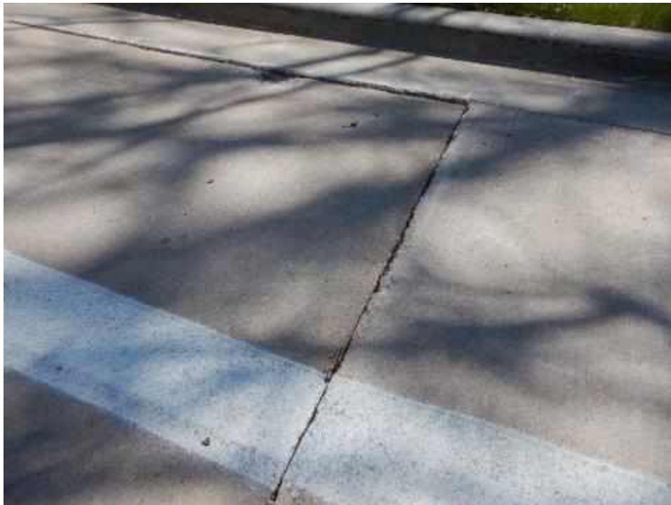
ARMRYA-E05-Faulting-(Sample Unit No. 01)
