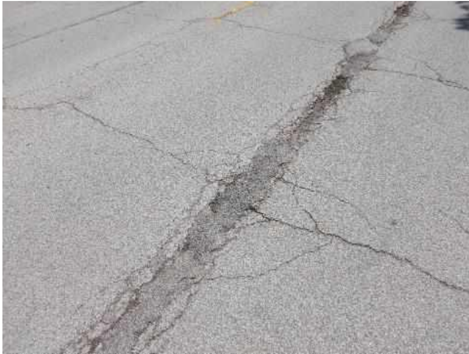
SIXTHS-S14-Joint Reflection Cracking-(Sample Unit No. 01)
