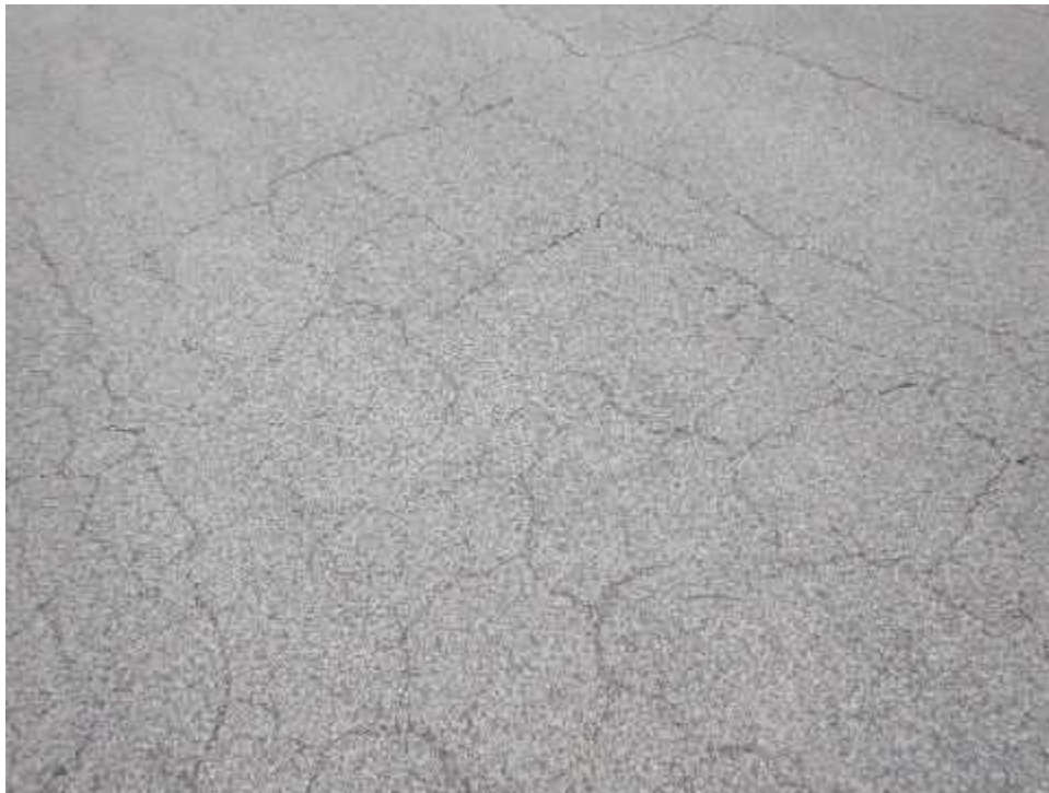
PENSYA-UW12B-Block Cracking-(Sample Unit No. 01)
