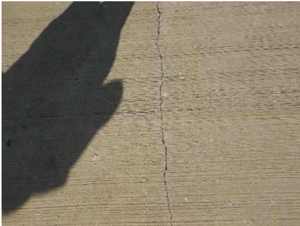
HAZELWDD-E01A-LTD Cracking-(Sample Unit No. 01)
