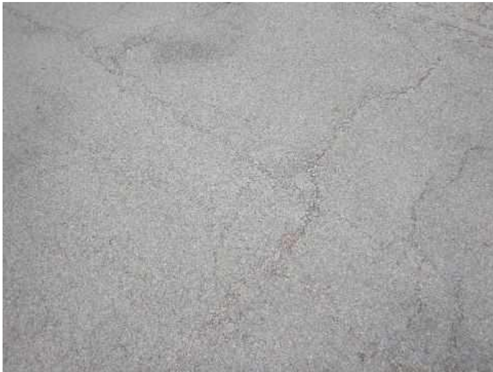
PENSYA-UW09B-Block Cracking-(Sample Unit No. 01)
