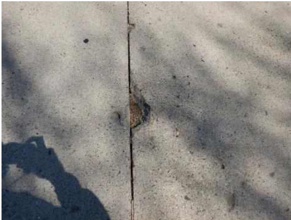
LNCLNAV-US19-Joint Spalling-(Sample Unit No. 01)
