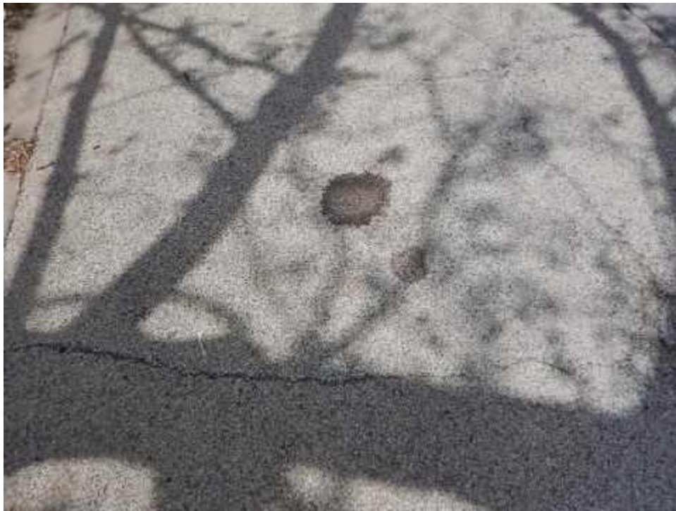
COLAGCT-UW09BS-Block Cracking-(Sample Unit No. 01)
