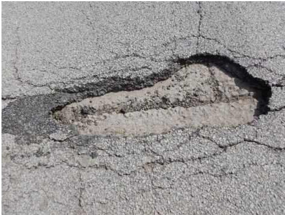
DORNRDR-US11AW-Pothole-(Sample Unit No. 01)
