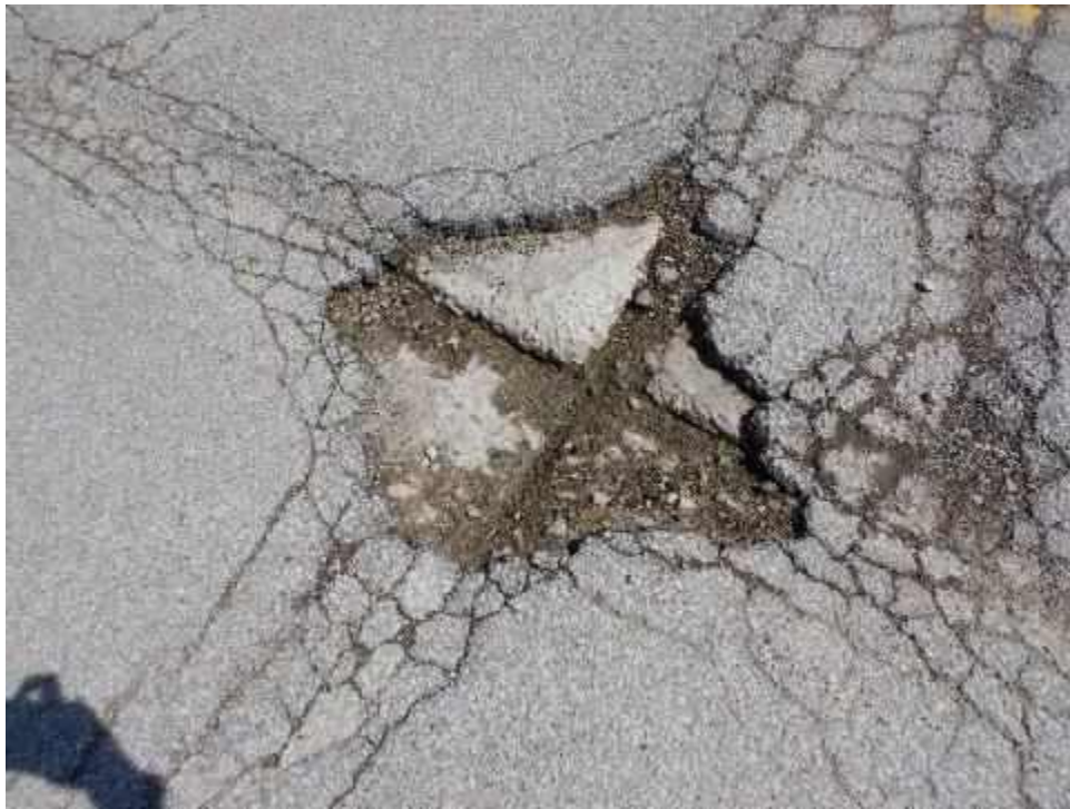
PEABYD-E01A-Pothole-(Sample Unit No. 01)
