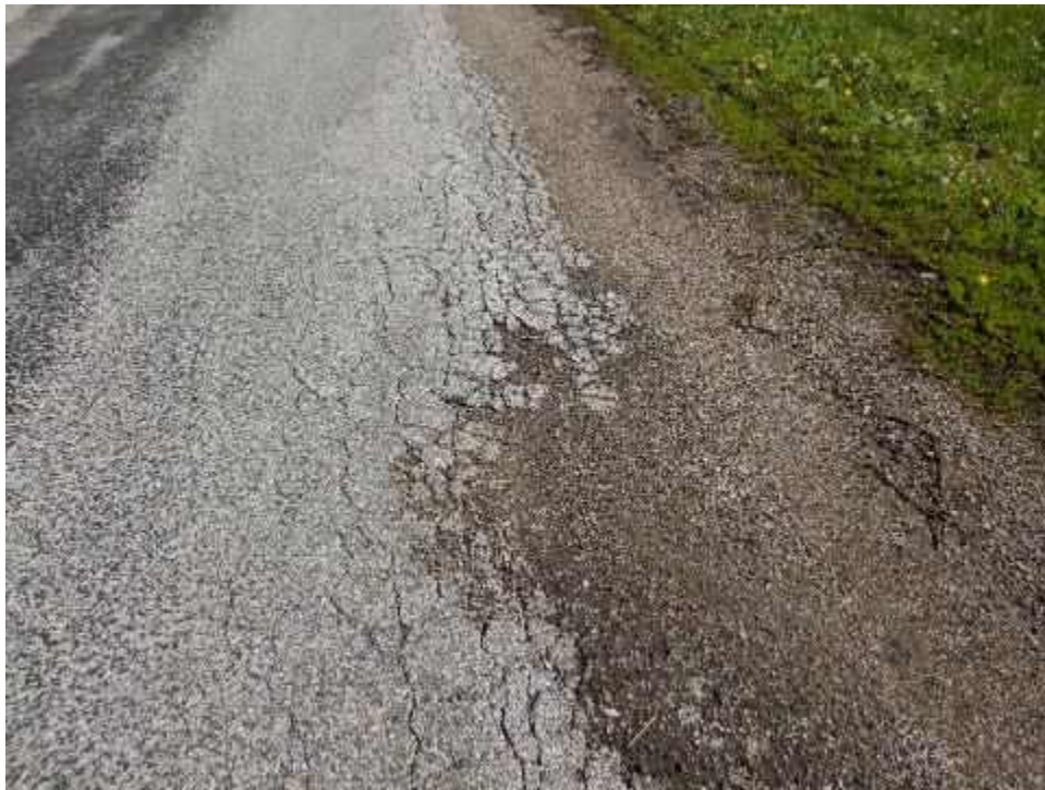
GRIFFITHD-S18-Alligator Cracking-(Sample Unit No. 01)
