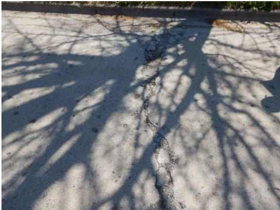
LNCLNAV-US19-Durability Cracking-(Sample Unit No. 01)
