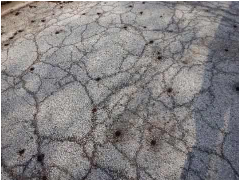
BAILEYD-E00-Alligator Cracking-(Sample Unit No. 02)
