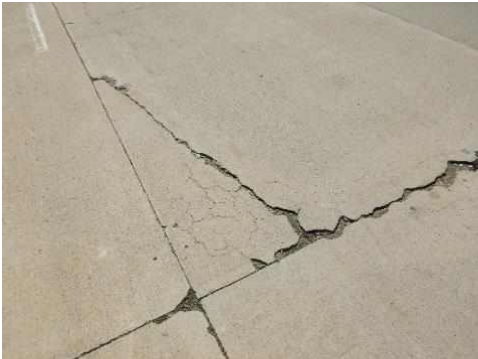
HAZELWDD-UW09-Durability Cracking-(Sample Unit No - 03)
