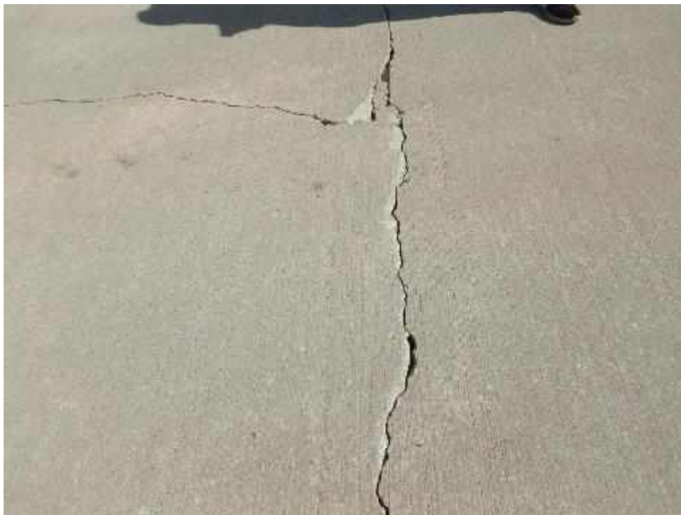
HAZELWDD-E01B-Shattered Slab-(Sample Unit No. 02)
