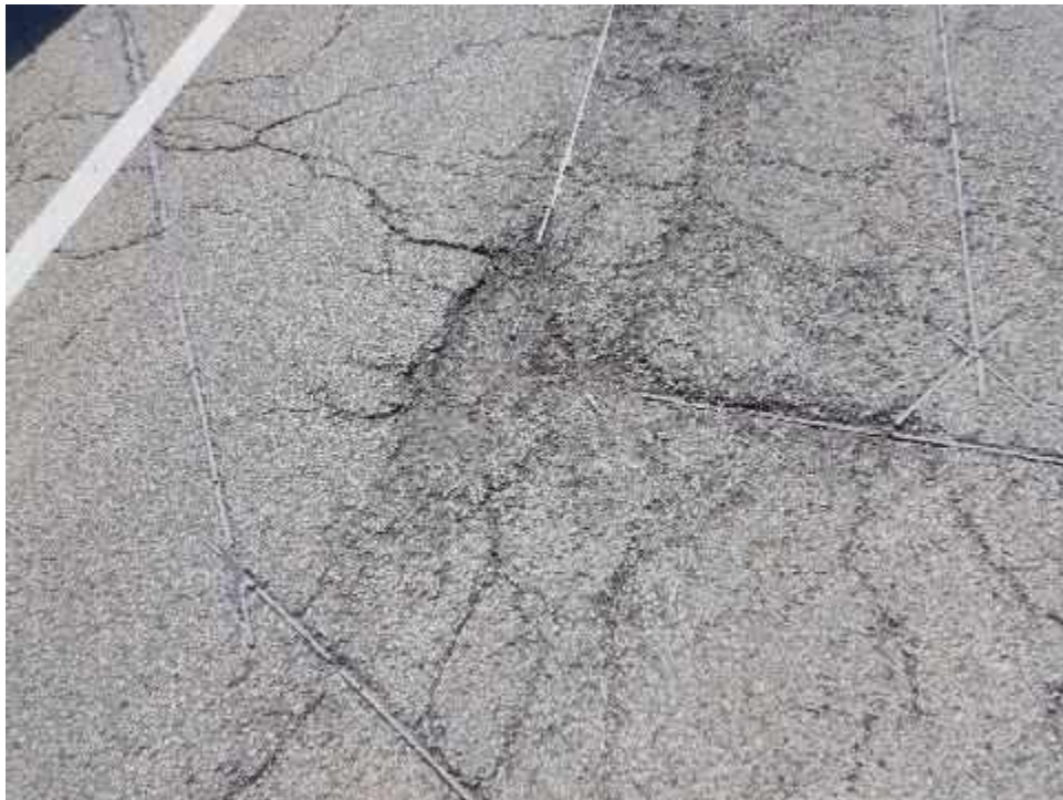
STADMD-E00A-Raveling-(Sample Unit No. 01)
