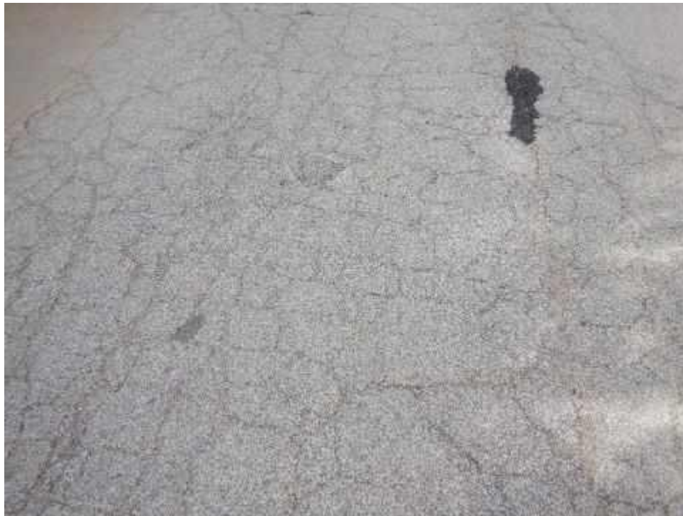
GRGRYST-US05-Alligator Cracking-(Sample Unit No. 01)
