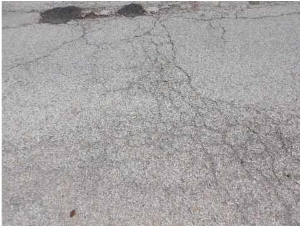
SIXTHS-S11-Alligator Cracking-(Sample Unit No. 01)
