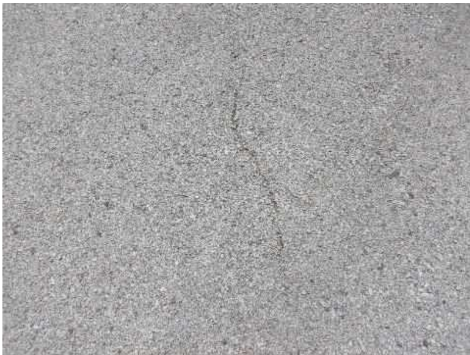
HAZELWDD-UW04-L&T Cracking-(Sample Unit No. 01)
