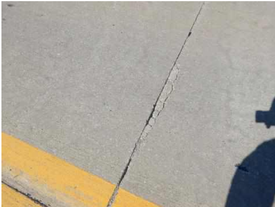
LNCLNAV-US23-Joint Spalling-(Sample Unit No. 01)
