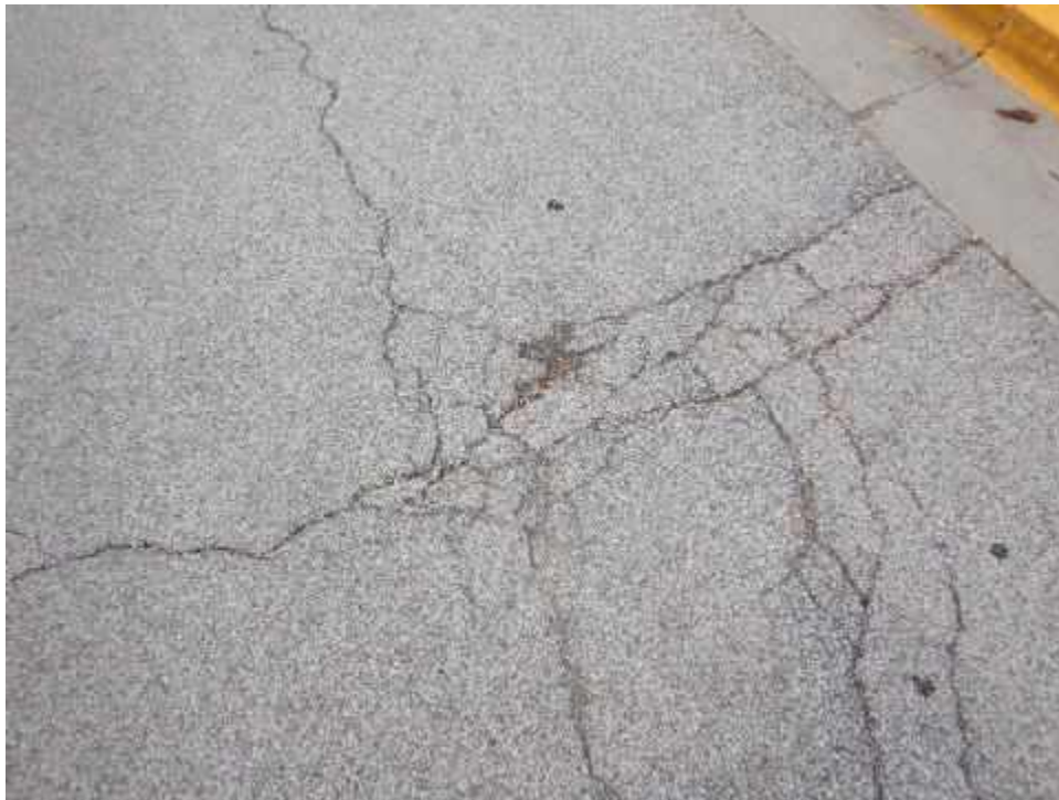
COLAGCT-UW09BN-Alligator Cracking-(Sample Unit No. 01)
