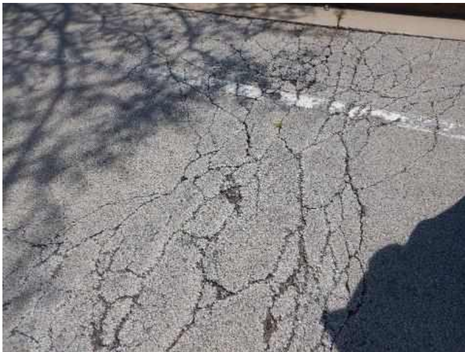
OAKS-S20B-Alligator Cracking-(Sample Unit No. 01)
