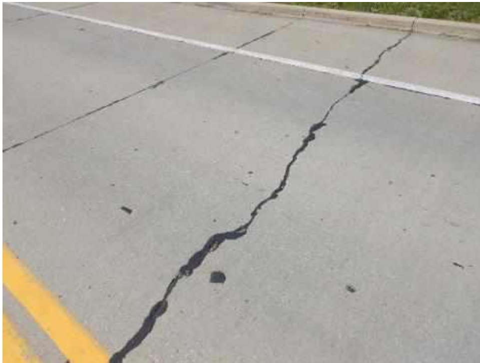
GREGYD-E02B-LTD Cracking-(Sample Unit No. 01)
