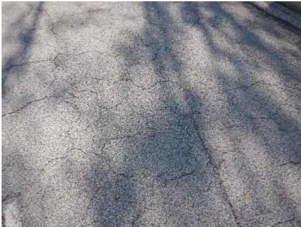
STMARR-E00D-Block Cracking-(Sample Unit No. 01)
