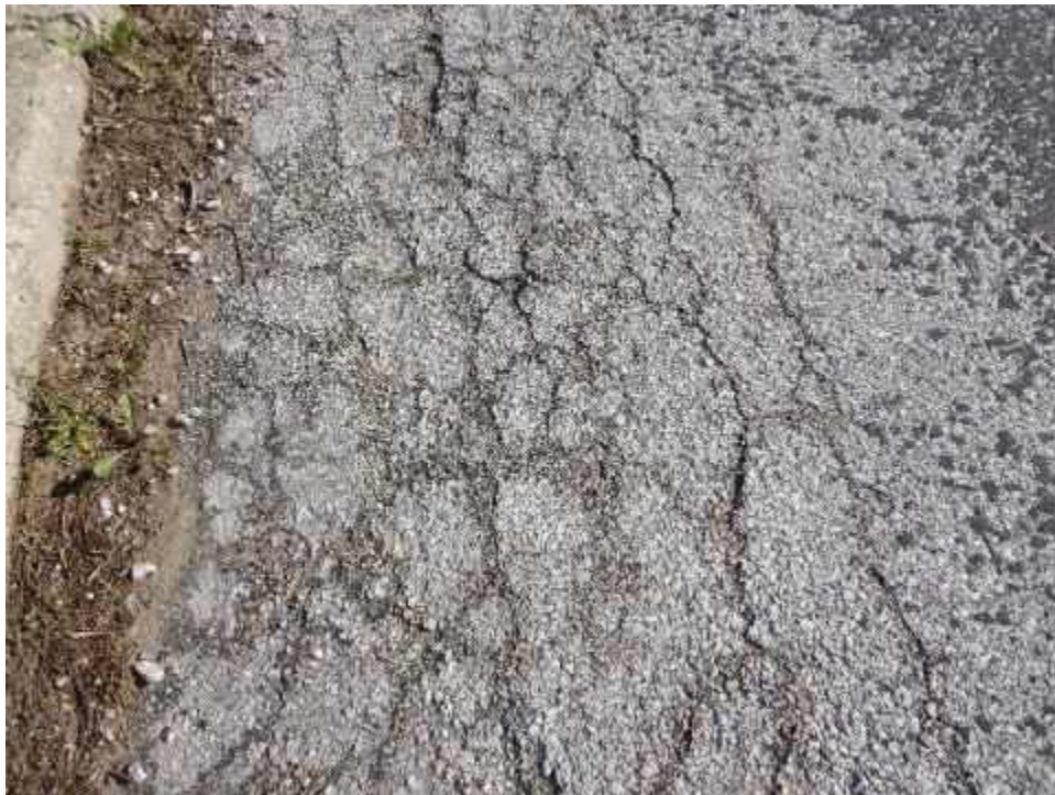
GRIFFITHD-S20-Alligator Cracking-(Sample Unit No. 01)
