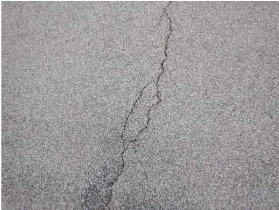
COLAGCT-UW09BN-L&T Cracking-(Sample Unit No. 01)
