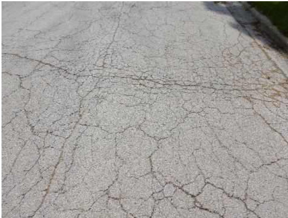
STOUGS-UW11-Alligator Cracking-(Sample Unit No. 01)
