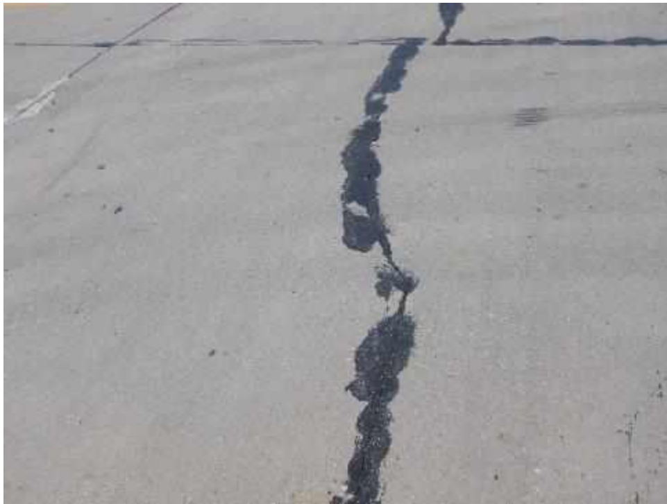
MRYLNDDR-US15-LTD Cracking-(Sample Unit No. 01)
