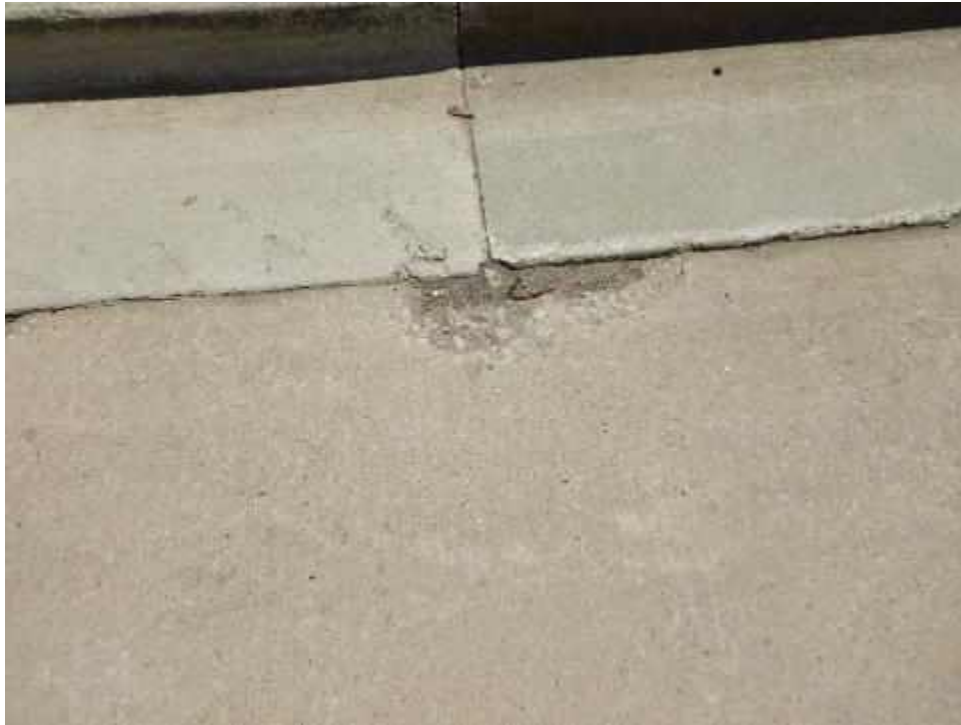
ARMRYA-E05-Joint Spalling-(Sample Unit No. 01)
