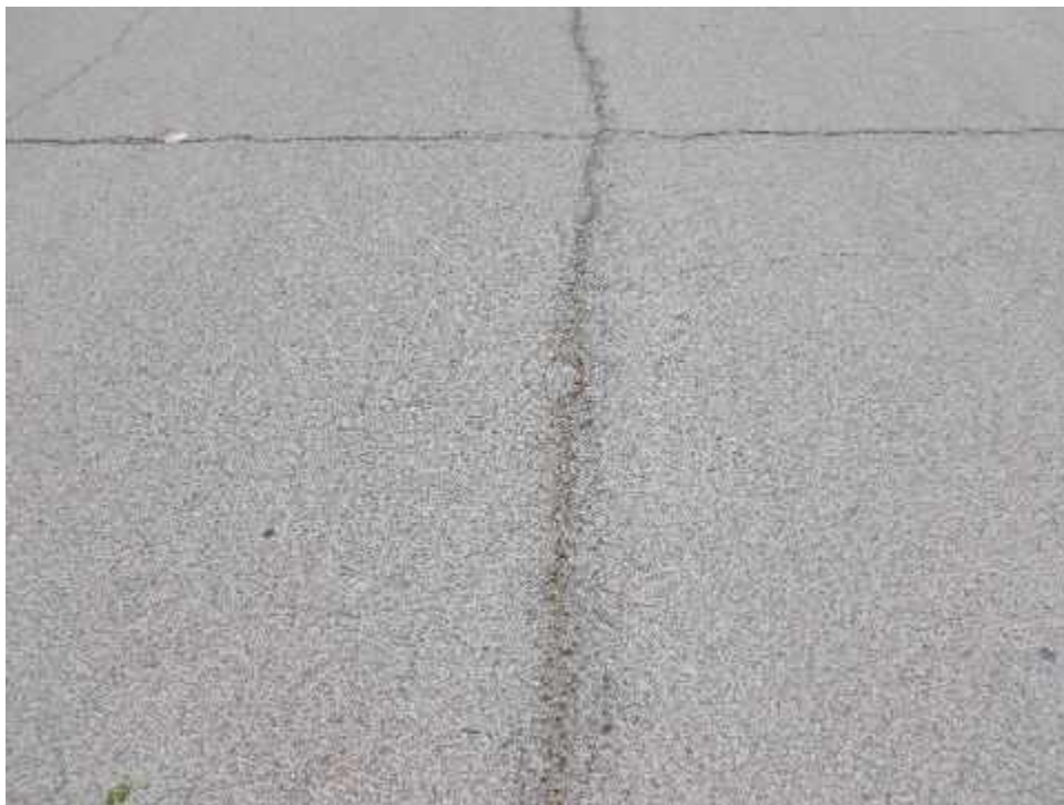
VRGNADR-US14A-L&T Cracking-(Sample Unit No. 01)
