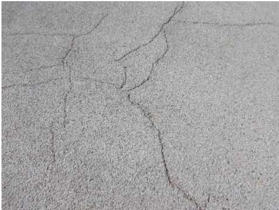
STMARR-E04B-L&T Cracking-(Sample Unit No. 01)
