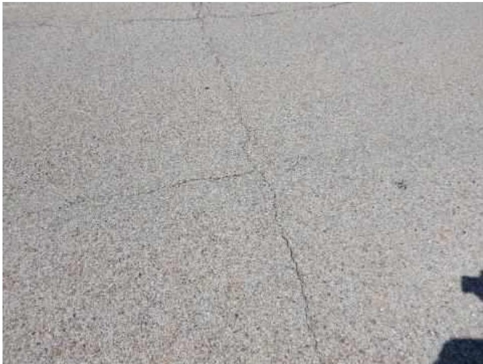
PEABYD-E01B-Joint Reflection Cracking-(Sample Unit No. 01)
