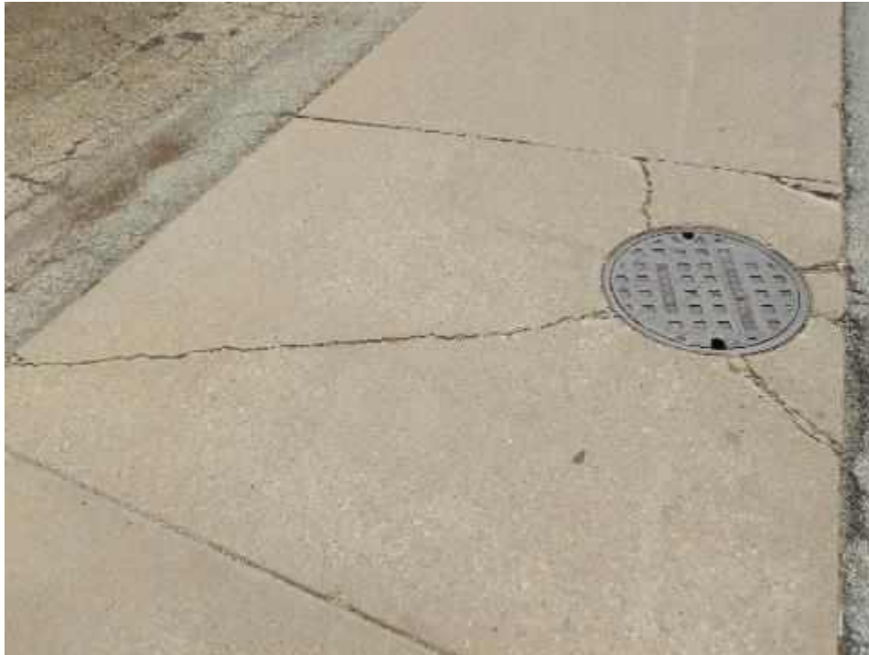
VRGNADR-US14BE-Shattered Slab-(Sample Unit No. 01)
