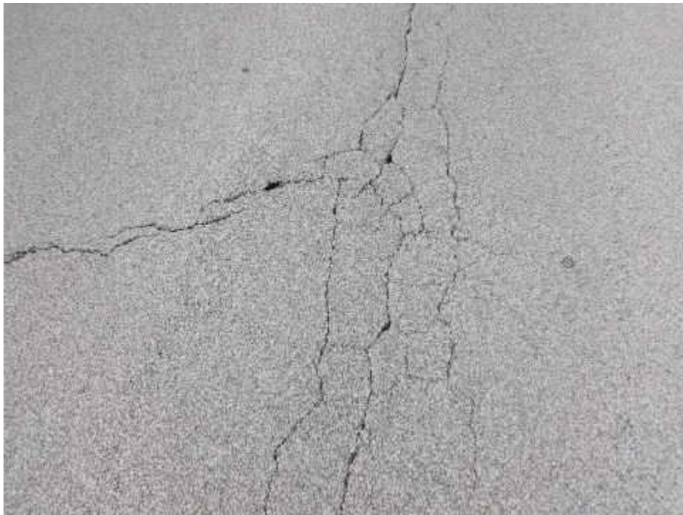
DORNRDR-US11AW-Alligator Cracking-(Sample Unit No. 01)
