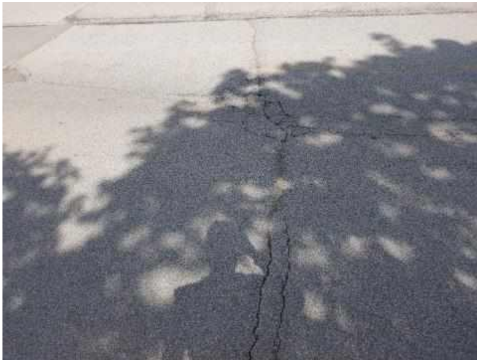
DORNRDR-US11BW-Joint Reflection Cracking-(Sample Unit No. 01)
