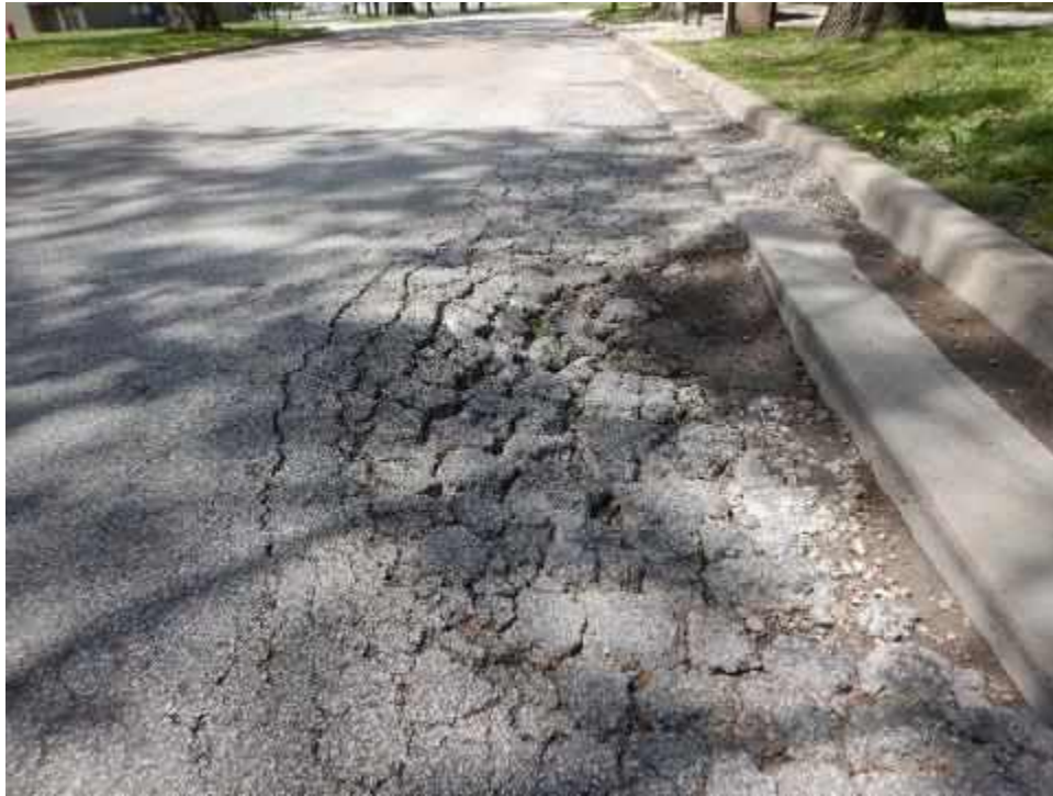
GHUFFDR-UW03-Alligator Cracking-(Sample Unit No. 01)
