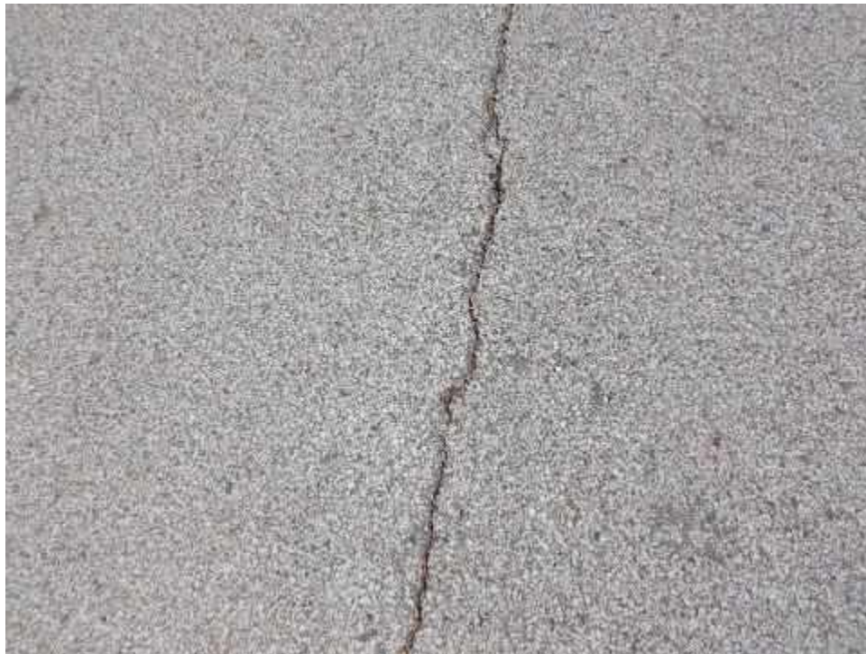
GHUFFDR-UW04AN-L&T Cracking-(Sample Unit No. 01)
