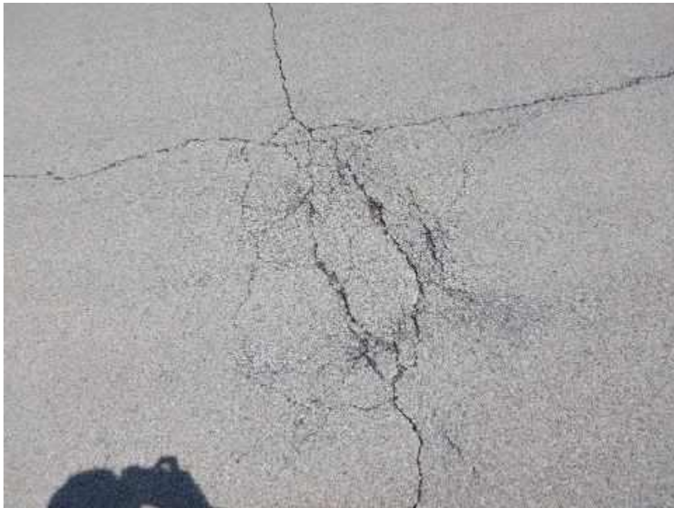
GHUFFDR-UW04BN-Alligator Cracking-(Sample Unit No. 01)
