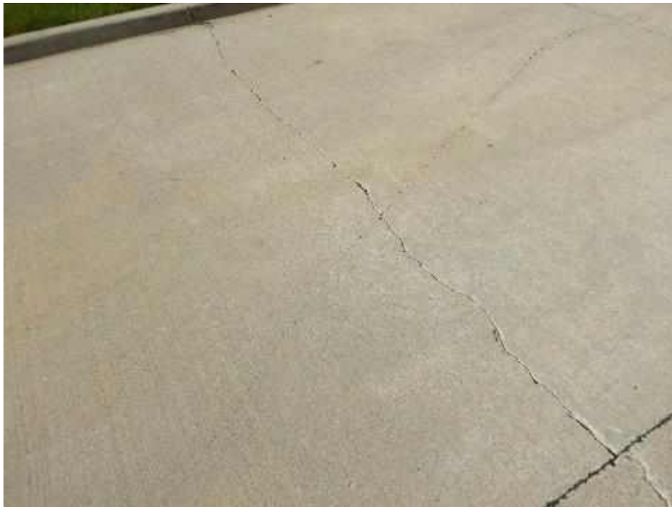
HAZELWDD-E01B-LTD Cracking-(Sample Unit No. 02)
