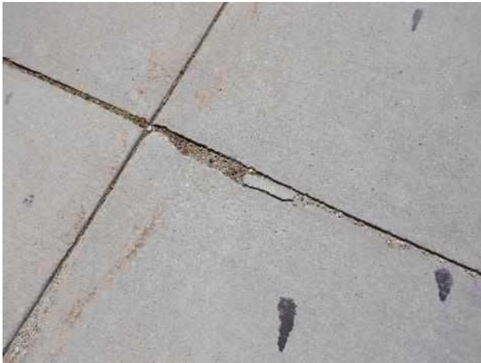
STADMD-E00C-Joint Spalling-(Sample Unit No. 071)
