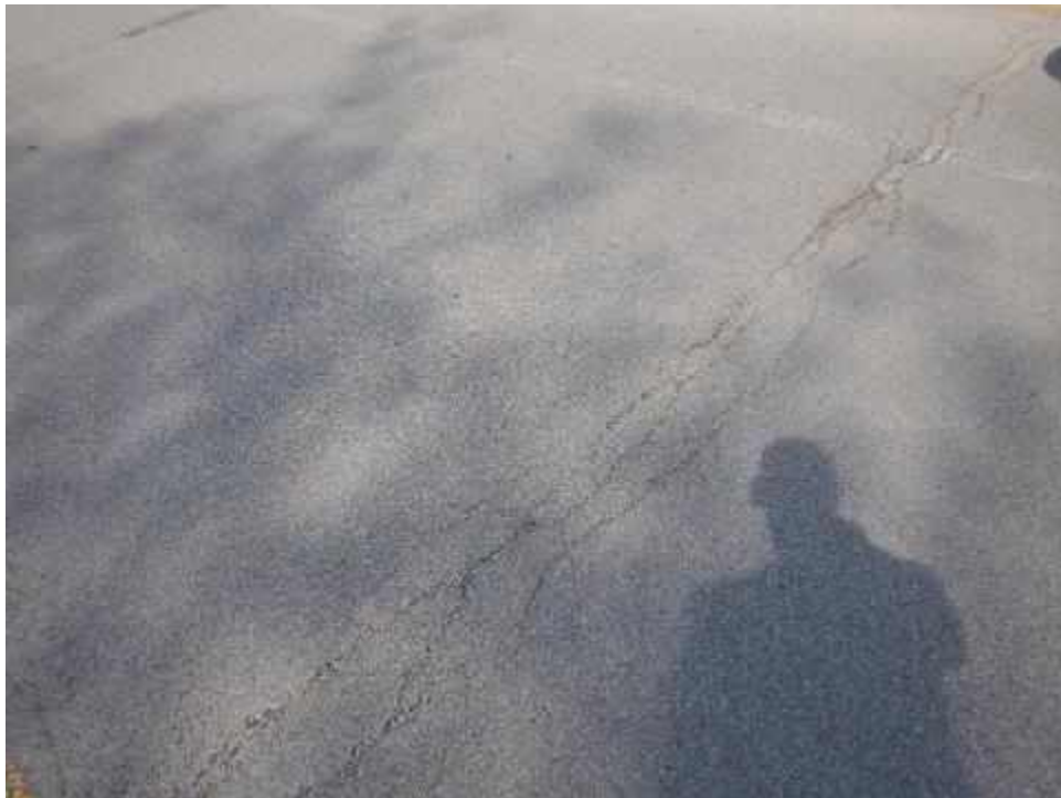
GOODWINA-US08-Joint Reflection Cracking-(Sample Unit No. 01)
