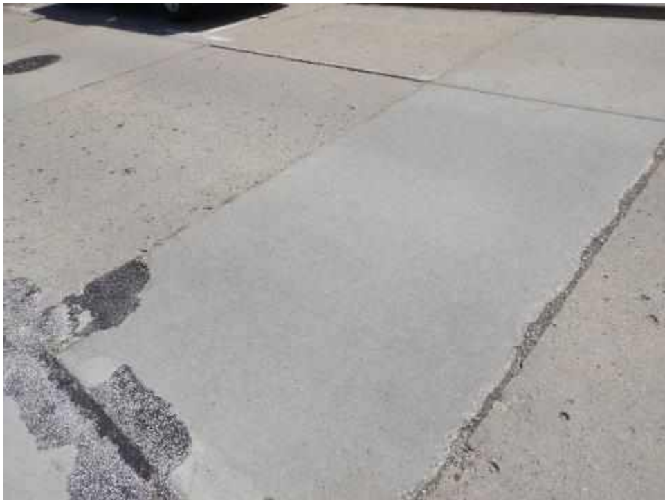
OAKS-S13-Large Patching-(Sample Unit No. 01)
