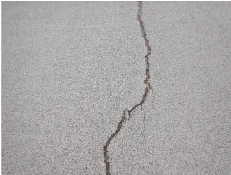
LORADOTD-UW12-L&T Cracking-(Sample Unit No. 01)
