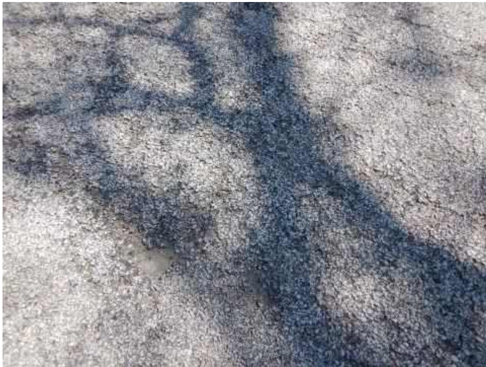
LNCLNAV-US17B-Raveling-(Sample Unit No. 01)
