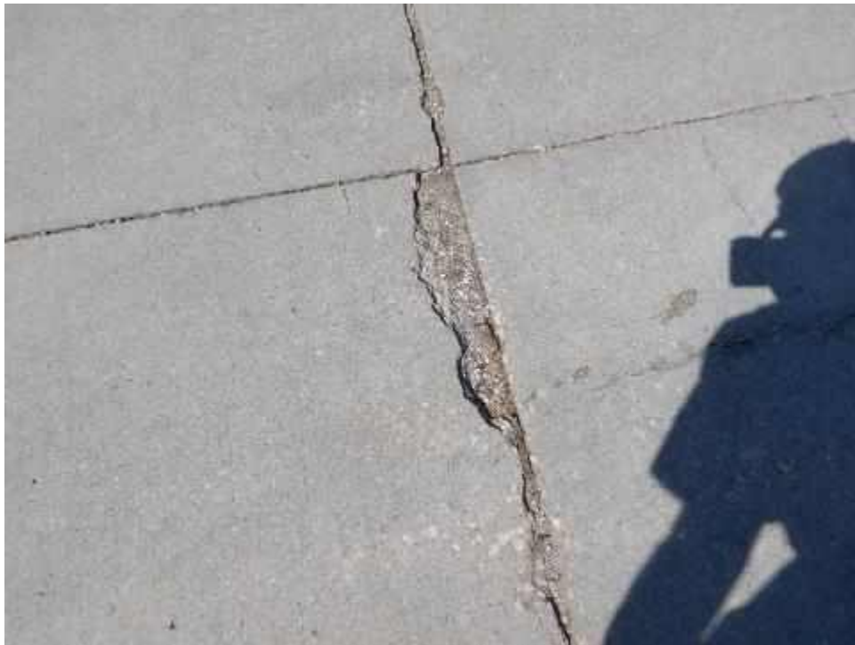
STADMD-E00D-Joint Spall-(Sample Unit No. 01)
