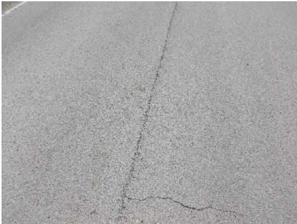
STMARR-UW09A-L&T Cracking-(Sample Unit No. 01)
