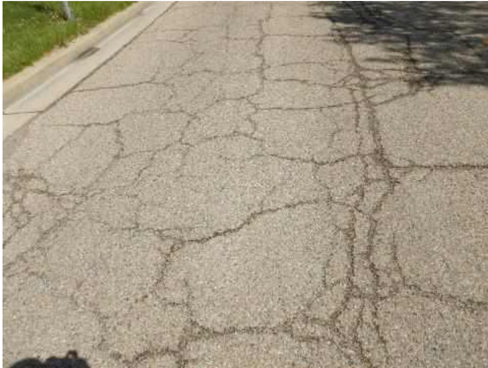
OAKS-S18A-Block Cracking-(Sample Unit No. 02)
