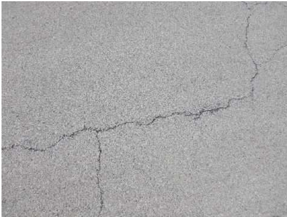
GHUFFDR-UW04BN-L&T Cracking-(Sample Unit No. 01)
