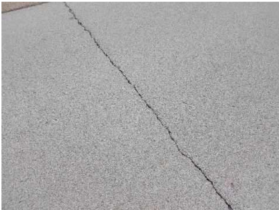
OAKS-S18B-L&T Cracking-(Sample Unit No. 05)
