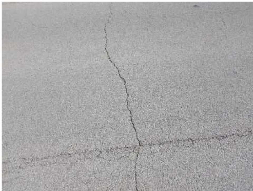
STMARR-E04A-L&T Cracking-(Sample Unit No. 01)
