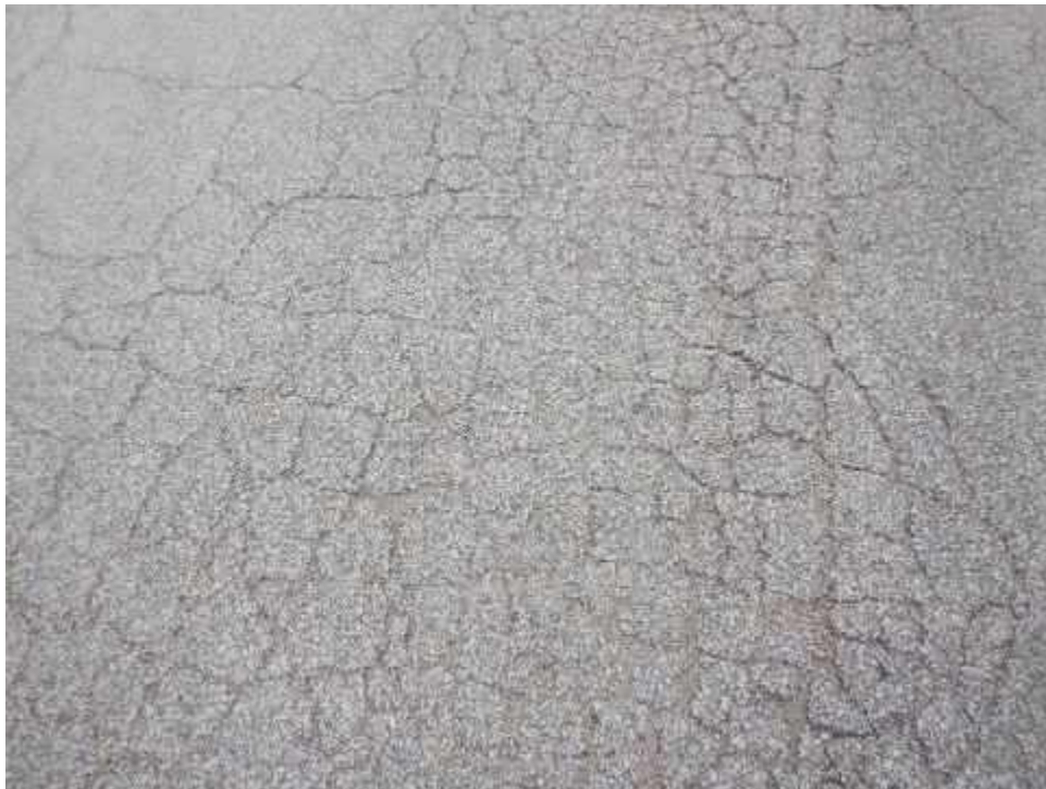
PENSYA-UW12B-Alligator Cracking-(Sample Unit No. 01)
