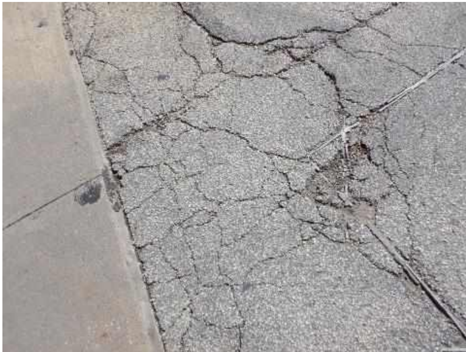
STADMD-E00A-Alligator Cracking-(Sample Unit No. 01)
