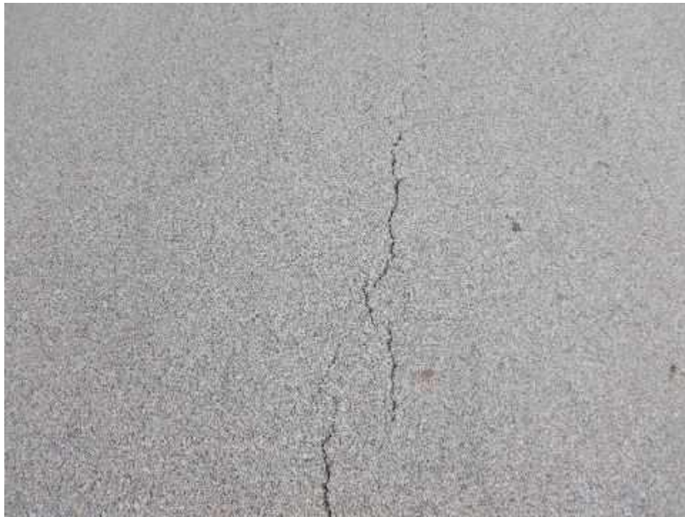
DORNRDR-US11AE-L&T Cracking-(Sample Unit No. 01)
