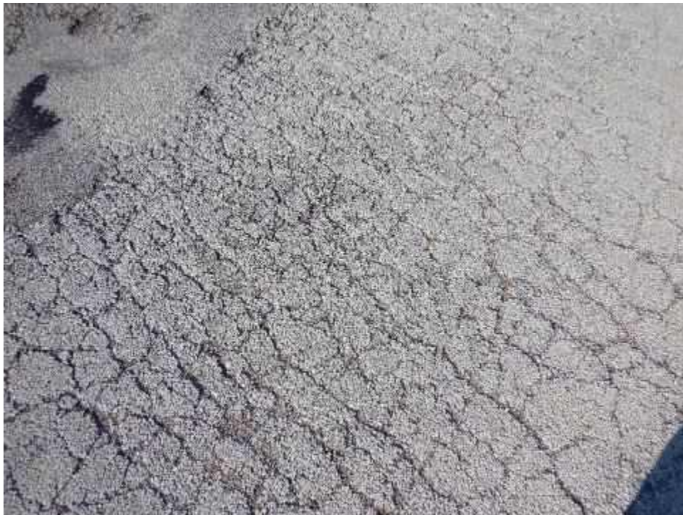
STMARR-E00A-Alligator Cracking-(Sample Unit No. 01)
