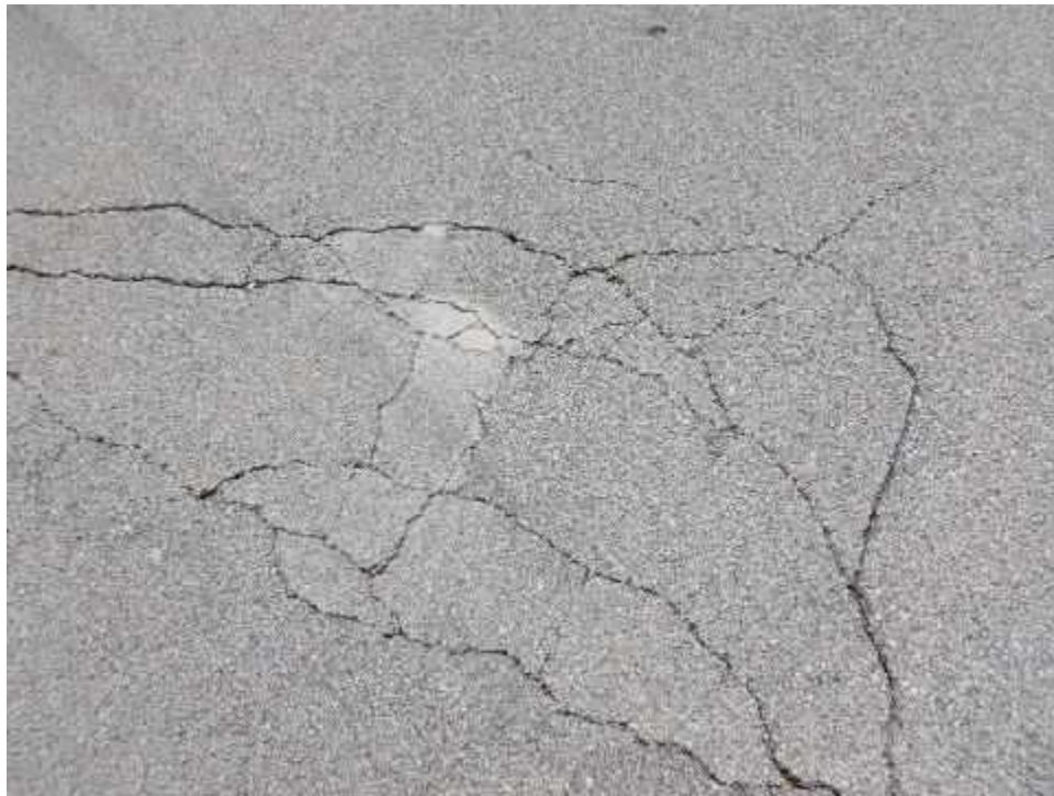
FIRSTS15-Alligator-Cracking-(Sample Unit No.01)
