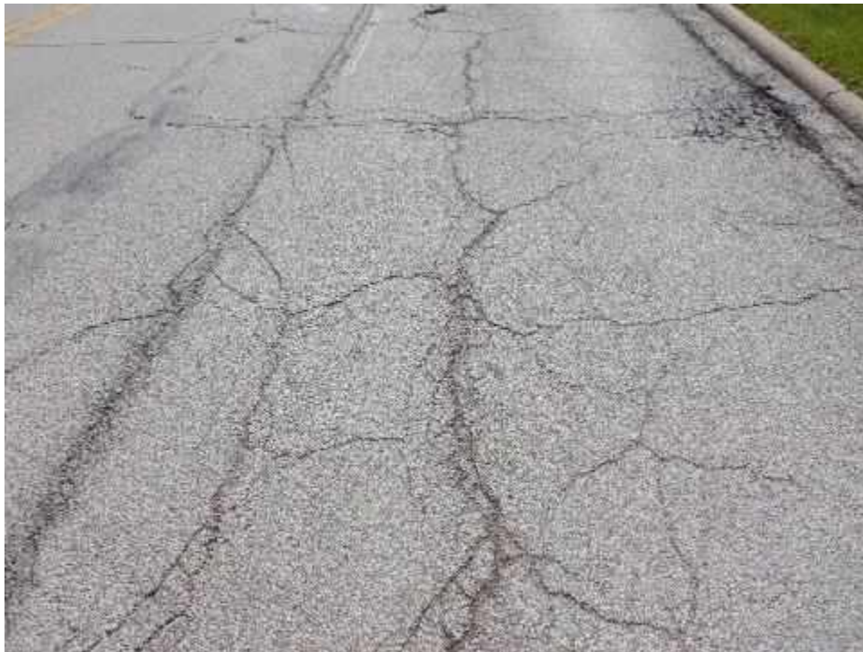
STMARR-E01-Block Cracking-(Sample Unit No. 01)
