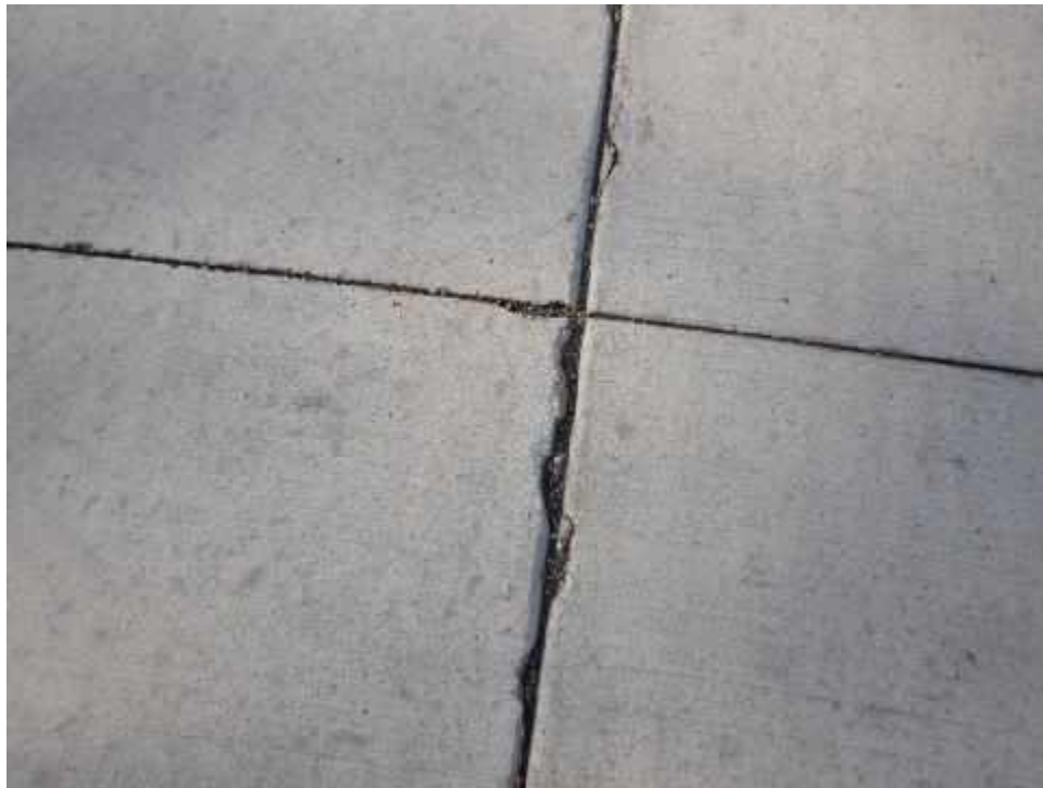
GRIFFITHD-S22A-Joint Seal Damage-(Sample Unit No. 01)
