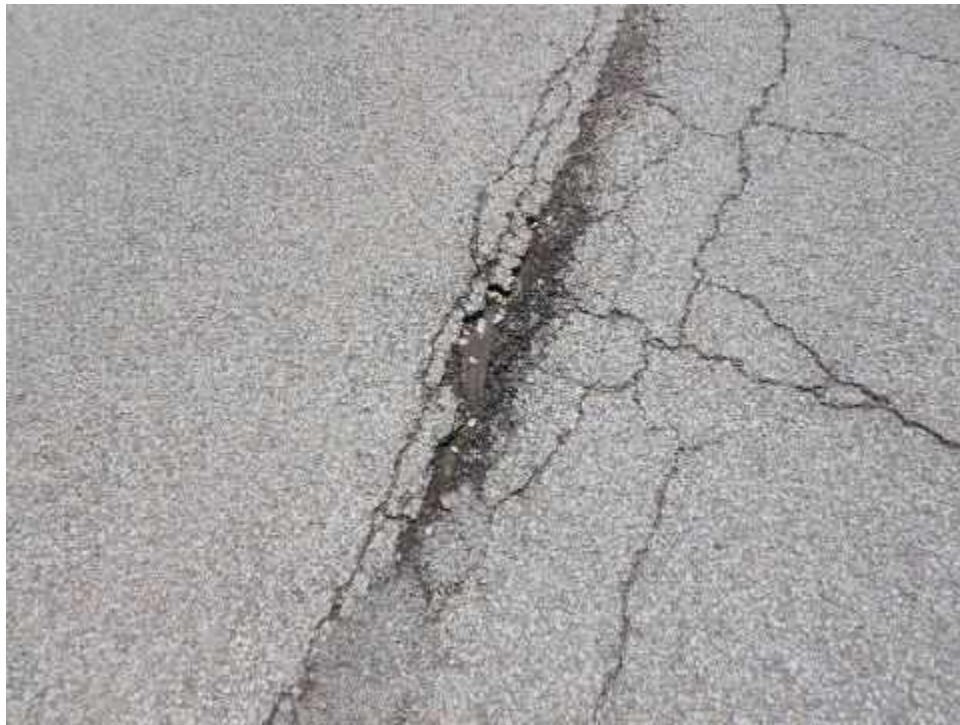
SIXTHS-S11-L&T Cracking-(Sample Unit No. 01)
