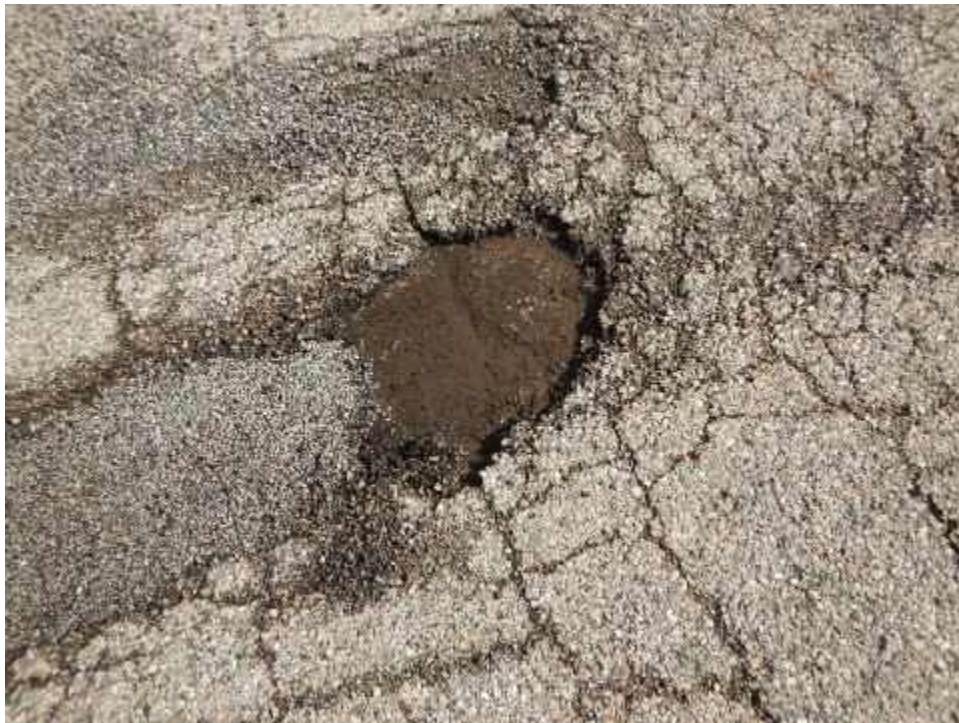
HAZELWDD-E00C-Pothole-(Sample Unit No. 02)
