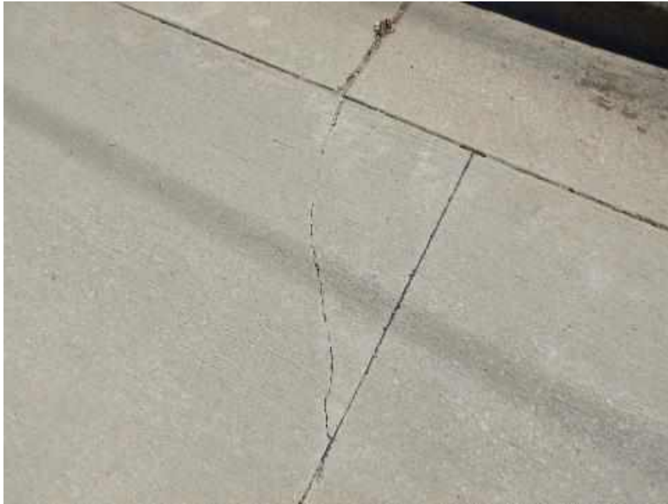
LNCLNAV-US21-Corner Break-(Sample Unit No - 04)
