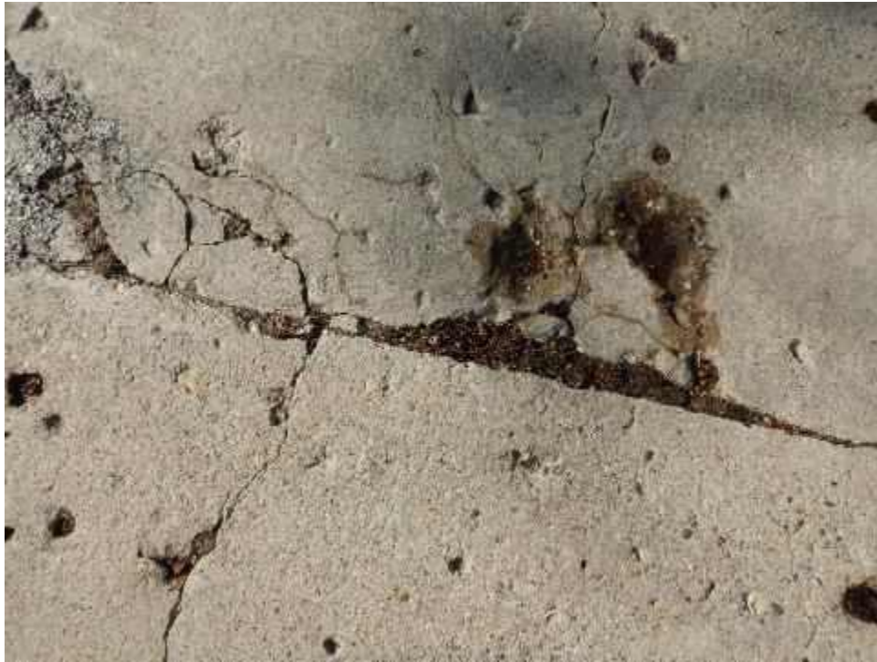
GERTYD-E00B-Joint Spalling-(Sample Unit No. 01)
