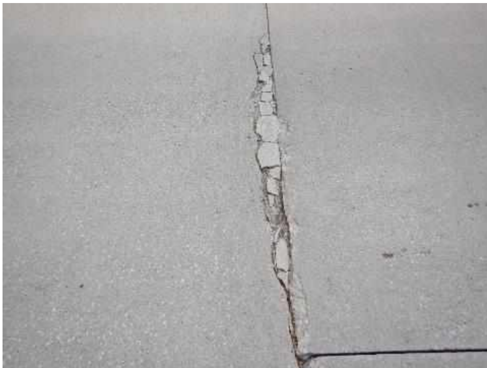
GREGYD-UW12D-Joint Spalling-(Sample Unit No. 01)
