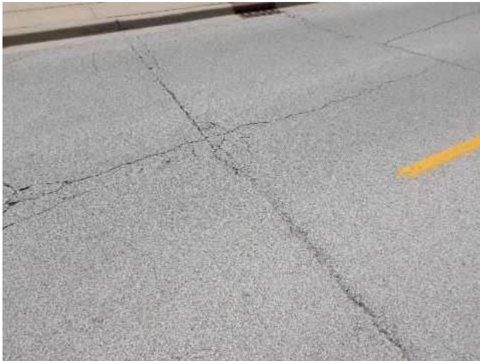
DORNRDR-US11AW-Joint Reflection Cracking-(Sample Unit No. 01)
