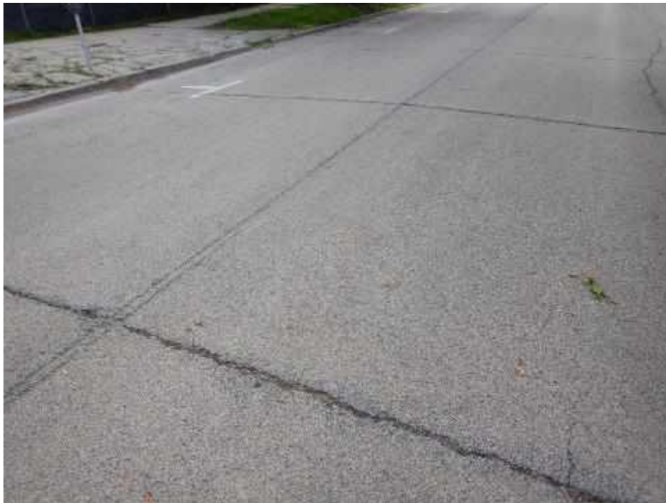
MAINS-UW11B-Joint Reflection Cracking-(Sample Unit No. 01)
