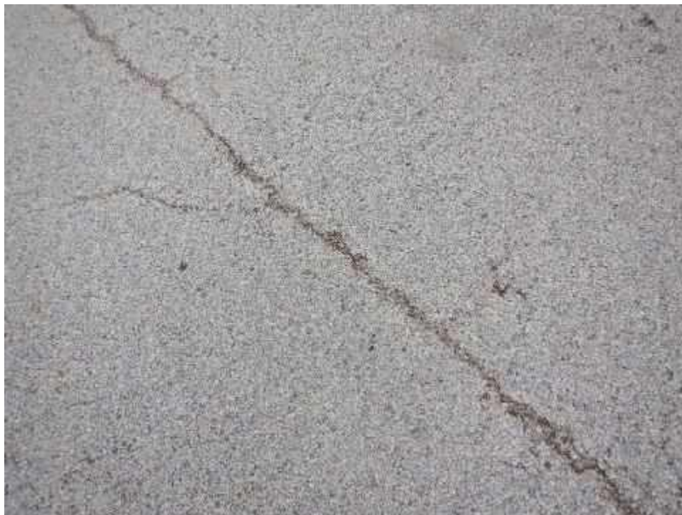
COLAGCT-UW09DN-L&T Cracking-(Sample Unit No. 01)
