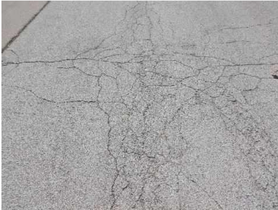
MAINS-UW11AN-Alligator Cracking-(Sample Unit No. 01)
