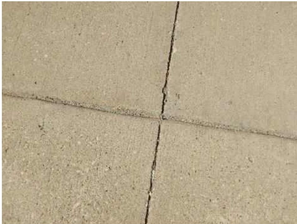
PEABYD-E04B-Joint Seal Damage-(Sample Unit No. 01)
