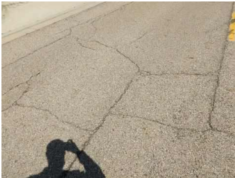
OAKS-S18A-Block Cracking-(Sample Unit No. 01)
