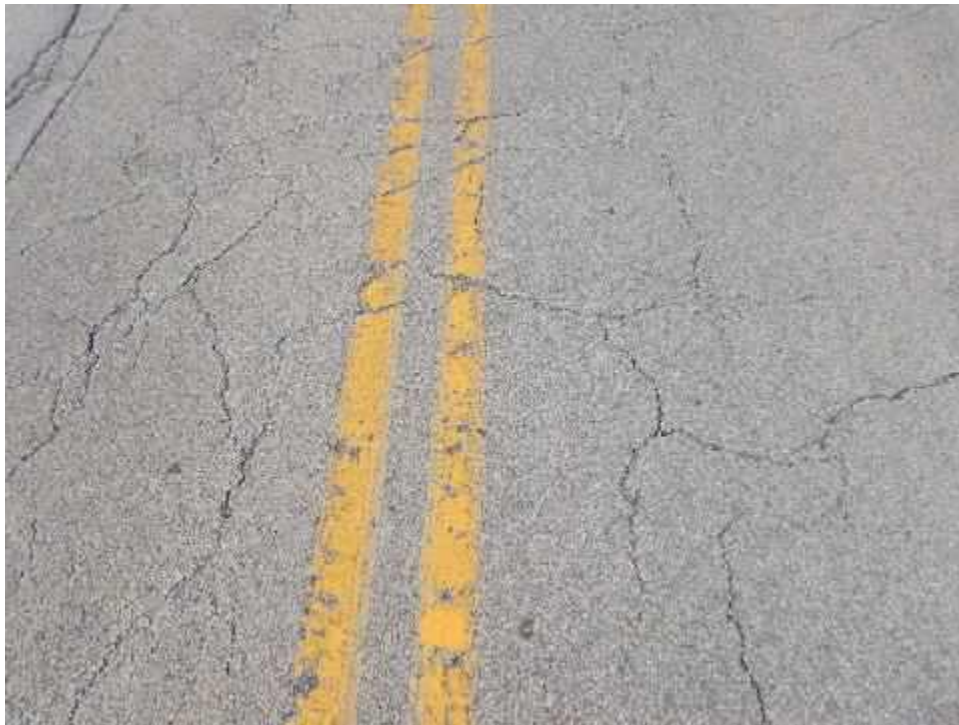
DORNRDR-US13E-Block Cracking-(Sample Unit No. 01)
