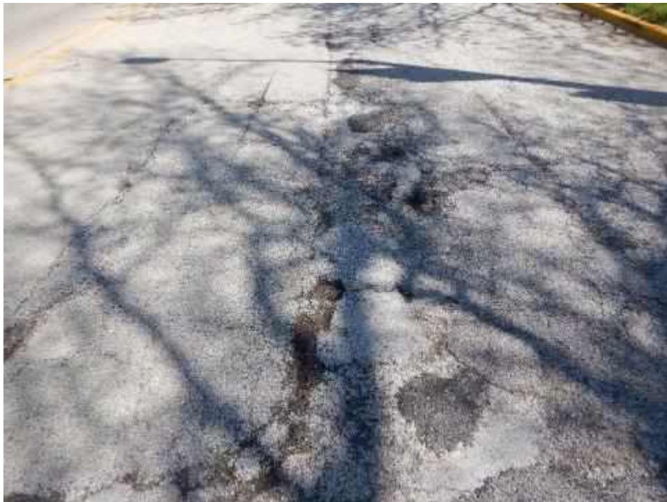
LNCLNAV-US17B-Joint Reflection Cracking-(Sample Unit No. 01)
