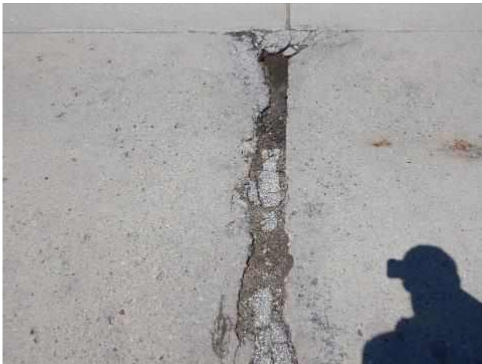
OAKS-S13-Durability Cracking-(Sample Unit No. 02)
