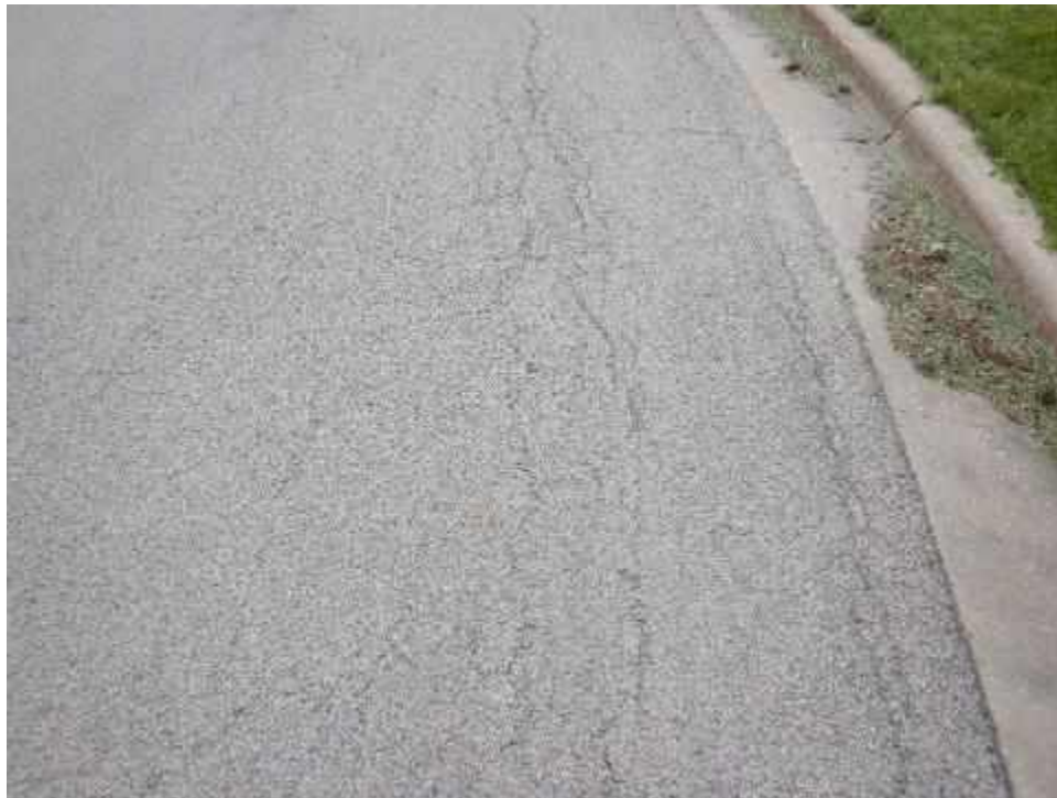
COLAGCT-UW09DN-Alligator Cracking-(Sample Unit No. 01)
