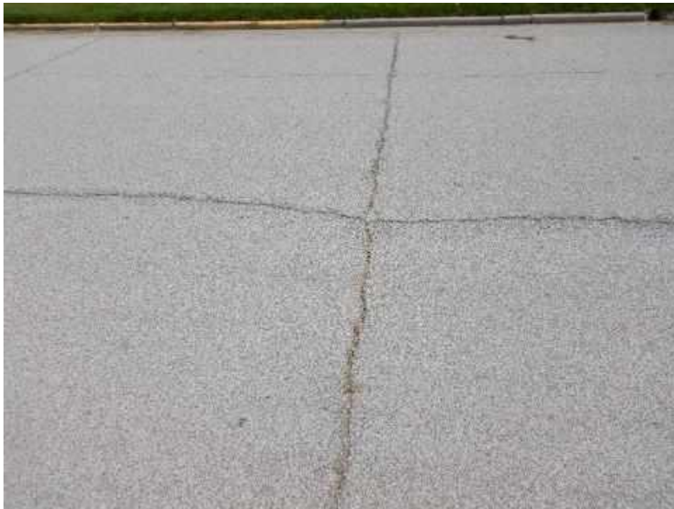
VRGNADR-US14A-Joint Reflection Cracking-(Sample Unit No. 01)
