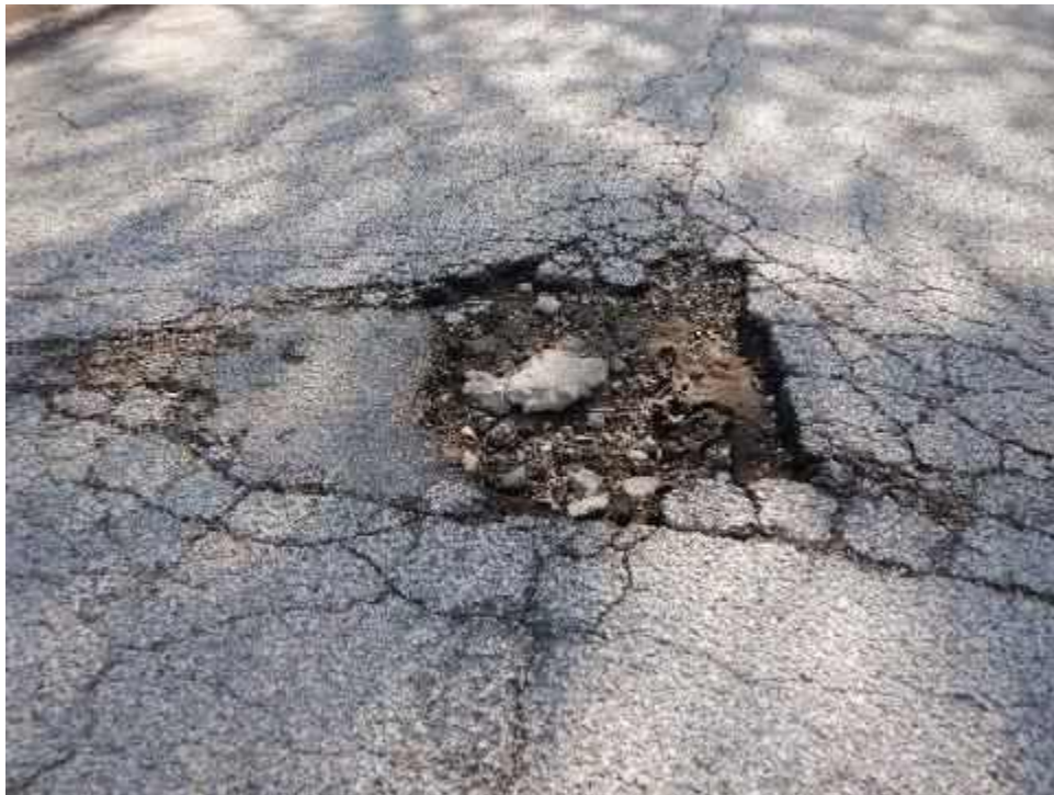
STMARR-E00D-Pothole-(Sample Unit No. 02) (2)
