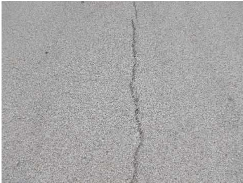
VRGNADR-US14BW-L&T Cracking-(Sample Unit No. 01)
