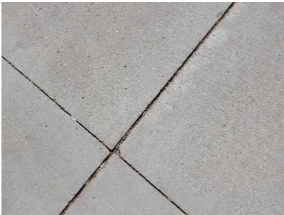
STADMD-E00D-Joint Seal Damage-(Sample Unit No. 02)
