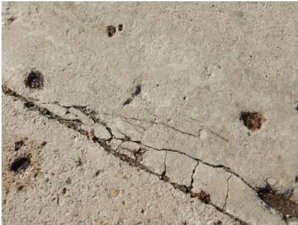
GERTYD-E00B-Durability Cracking-(Sample Unit No. 01)
