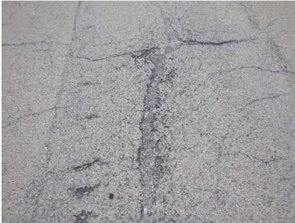
STOUGS-UW13-L&T Cracking-(Sample Unit No. 02)
