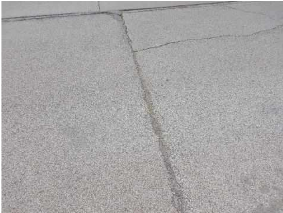
DORNRDR-US11BE-Joint Reflection Cracking-(Sample Unit No. 01)
