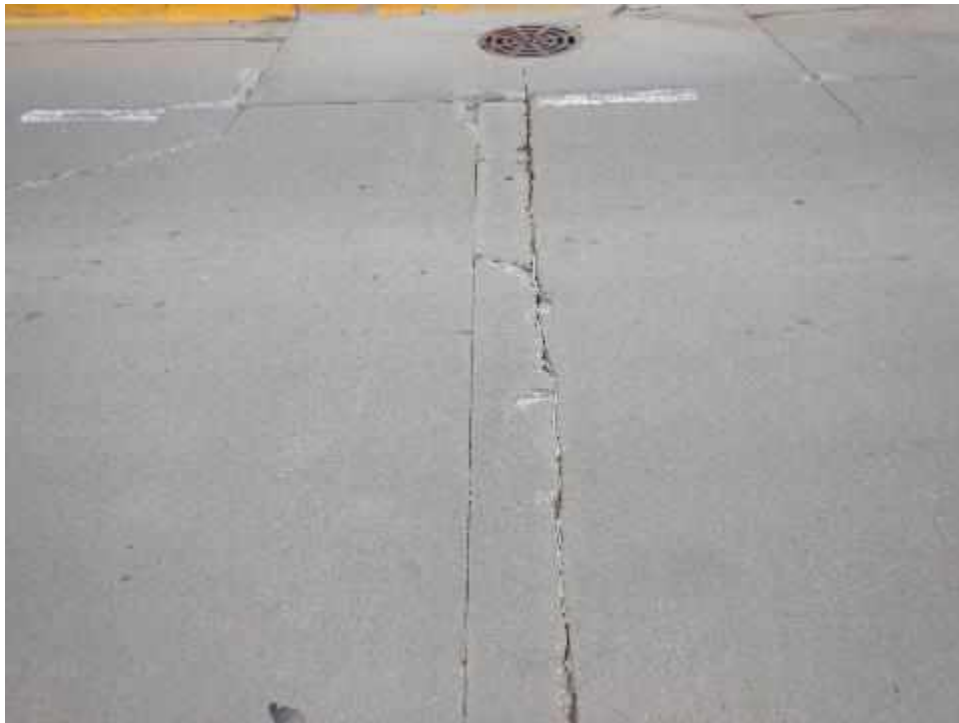
GREGYD-UW12B-Large Patching-(Sample Unit No. 01)
