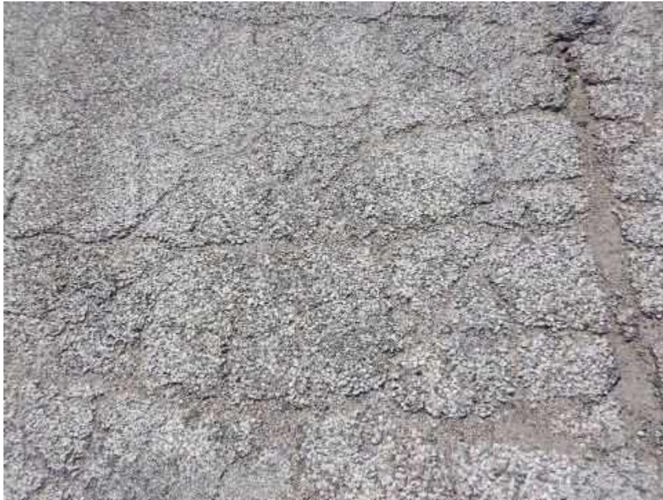
PEABYD-E06A-Alligator Cracking-(Sample Unit No. 01)
