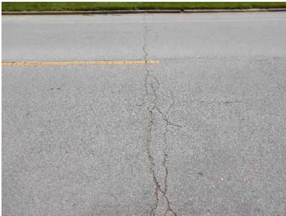
FIRSTS-S15-Joint Reflection Cracking-(Sample Unit No. 01)
