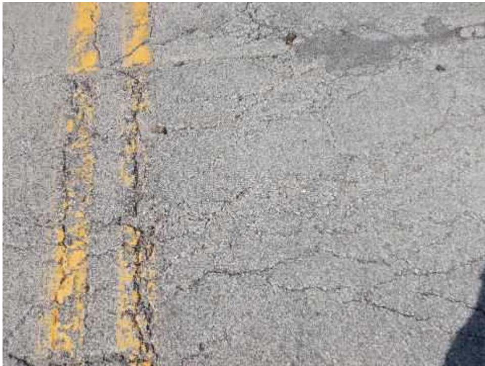
DORNRDR-US13E-Alligator Cracking-(Sample Unit No. 01)
