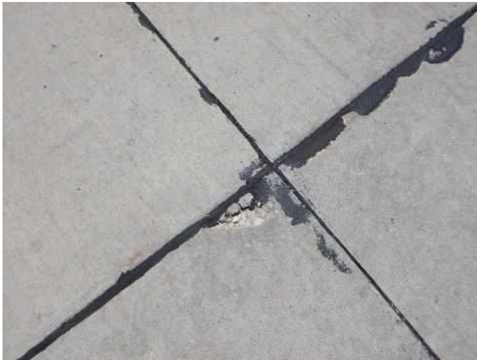
GREGYD-E03B-Corner Spalling-(Sample Unit No. 01)
