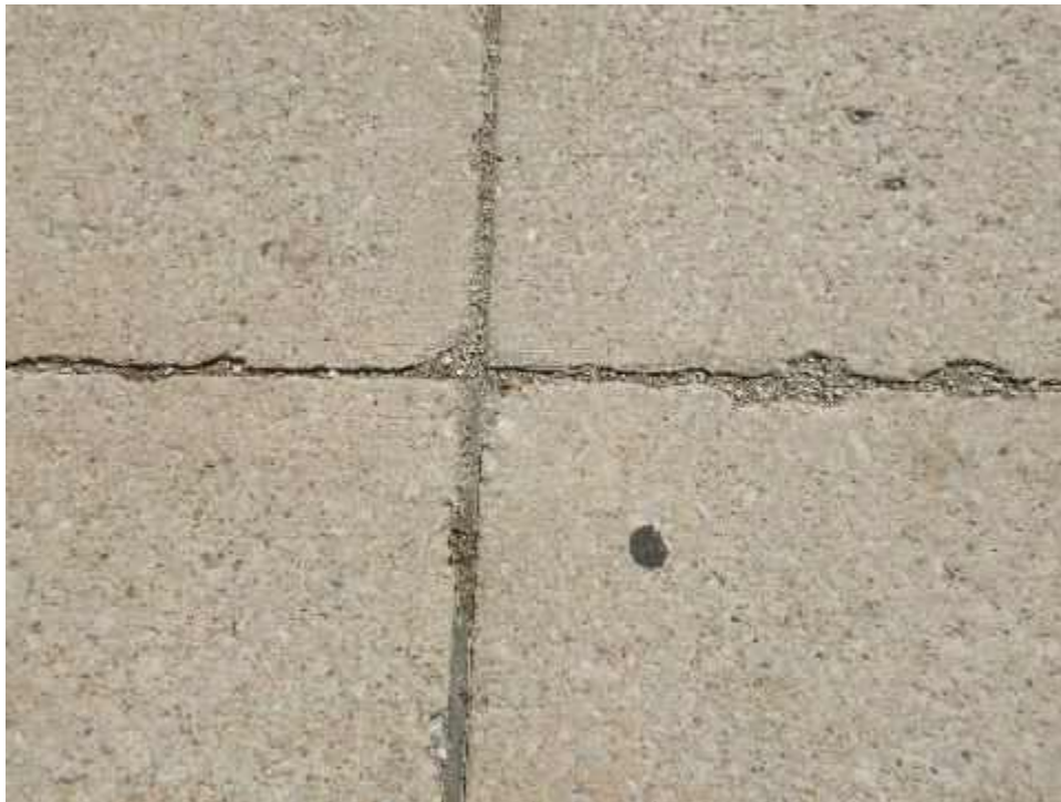
HAZELWDD-UW09-Joint Seal Damage-(Sample Unit No. 01)
