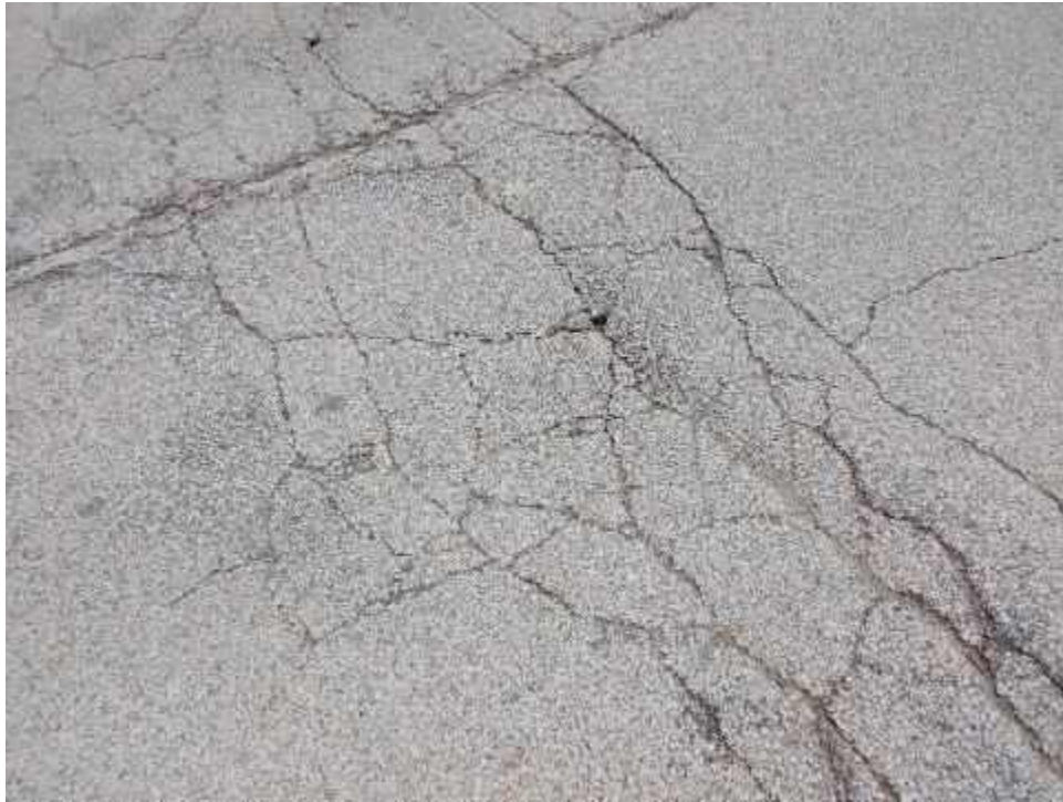
SIXTHS-S13-Alligator Cracking-(Sample Unit No. 01)
