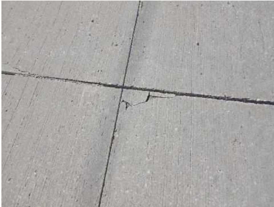
LNCLNAV-US23-Corner Spalling-(Sample Unit No. 01)
