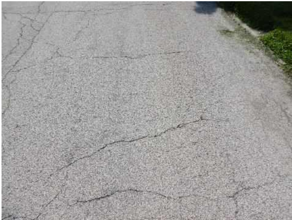
MAINS-UW11AN-Block Cracking-(Sample Unit No. 01)
