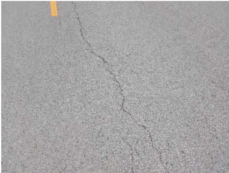
GHUFFDR-UW03-L&T Cracking-(Sample Unit No. 01)
