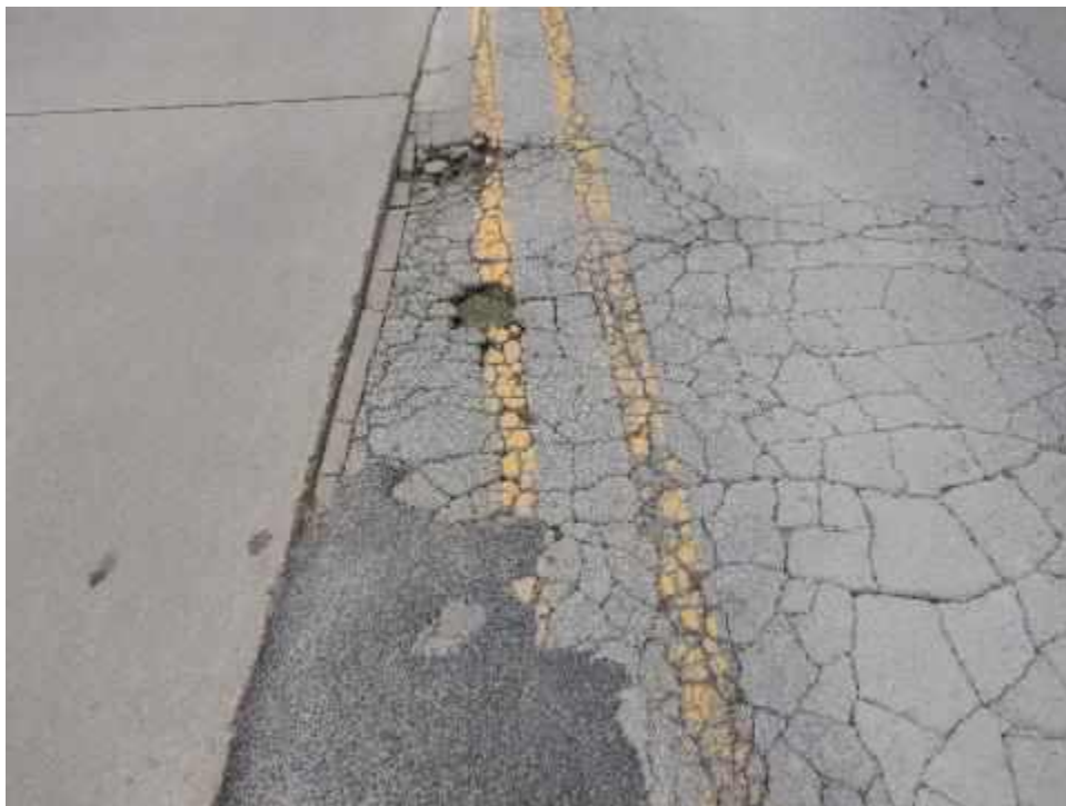
PENSYA-UW11A-Alligator Cracking-(Sample Unit No. 01)
