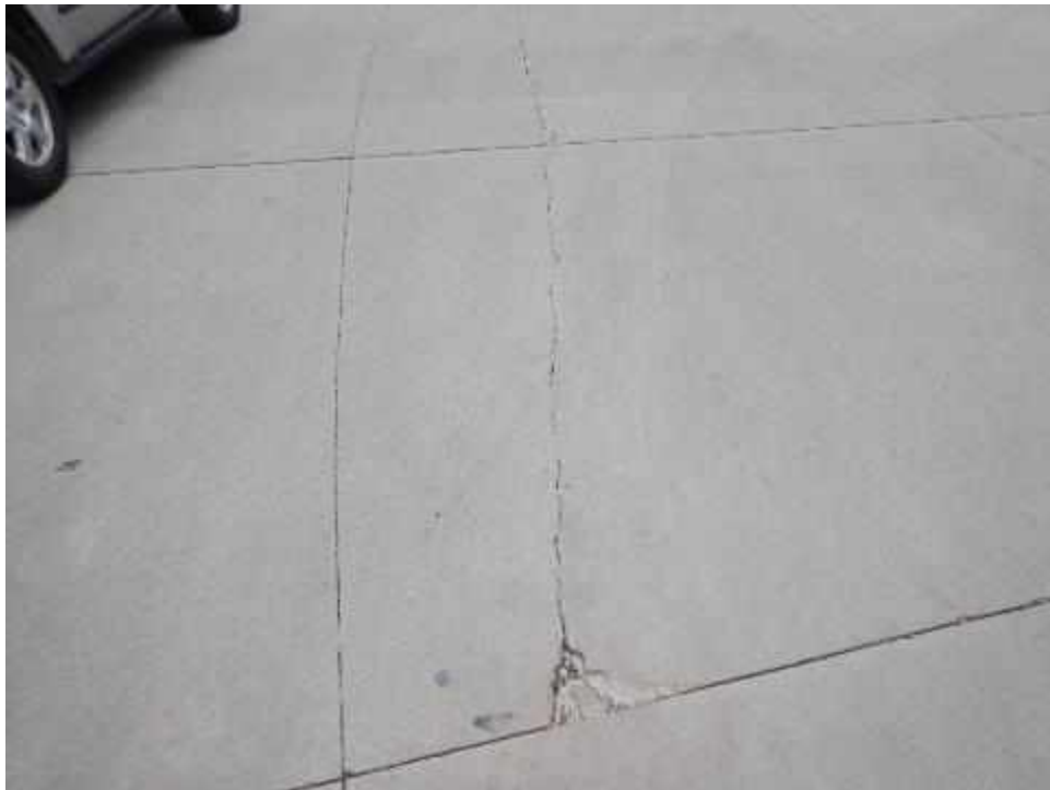
COLAGCT-UW09CN-LTD Cracking-(Sample Unit No. 01)
