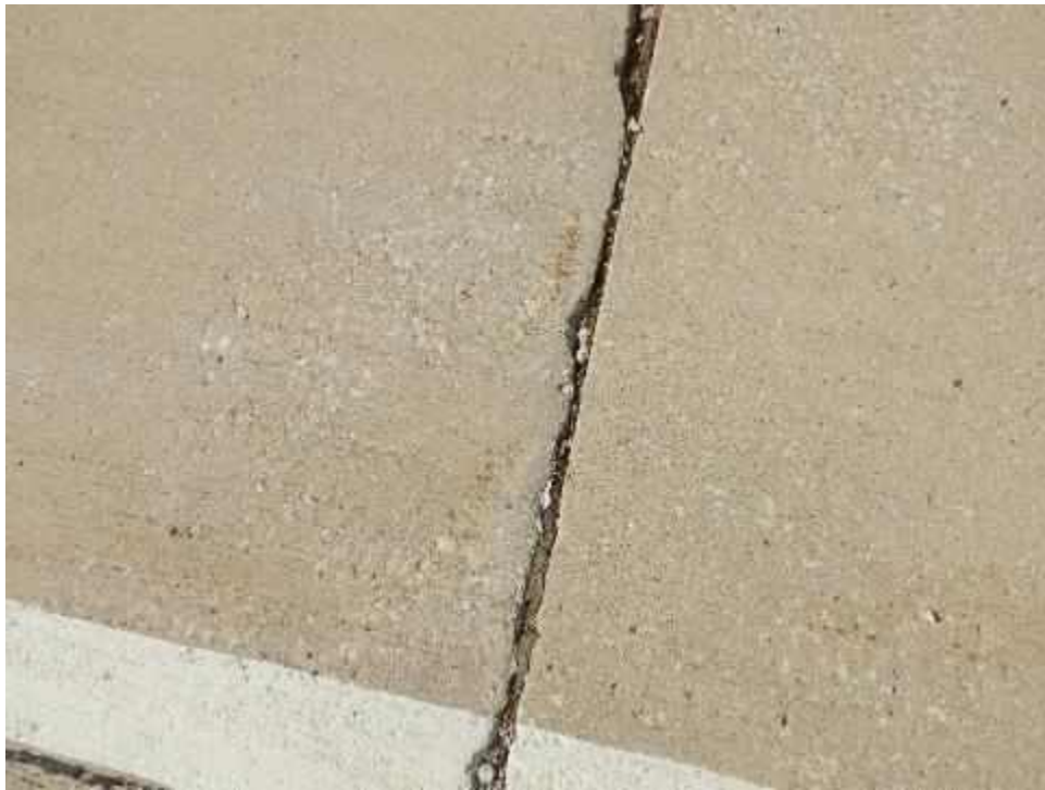
STOUGS-UW12-Joint Seal Damage-(Sample Unit No. 01)
