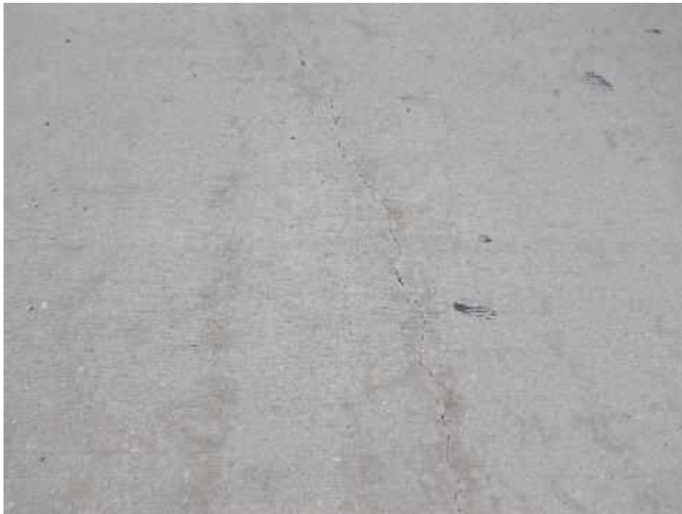
GREGYD-E03B-LTD Cracking-(Sample Unit No. 01)
