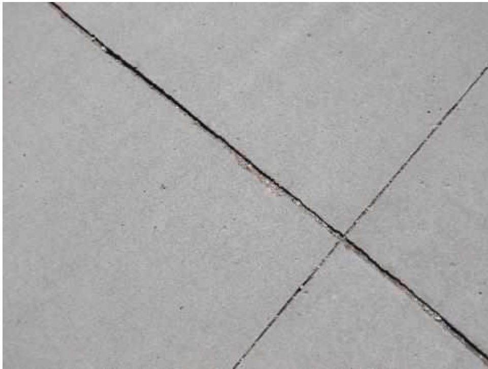
STADMD-E00C-Joint Seal Damage-(Sample Unit No. 01)
