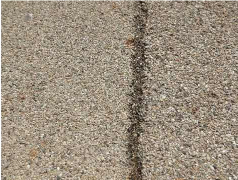
HAZELWDD-E00C-L&T Cracking-(Sample Unit No. 01)
