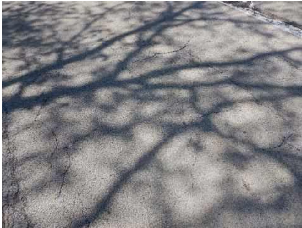
LNCLNAV-US17B-Block Cracking-(Sample Unit No. 02)
