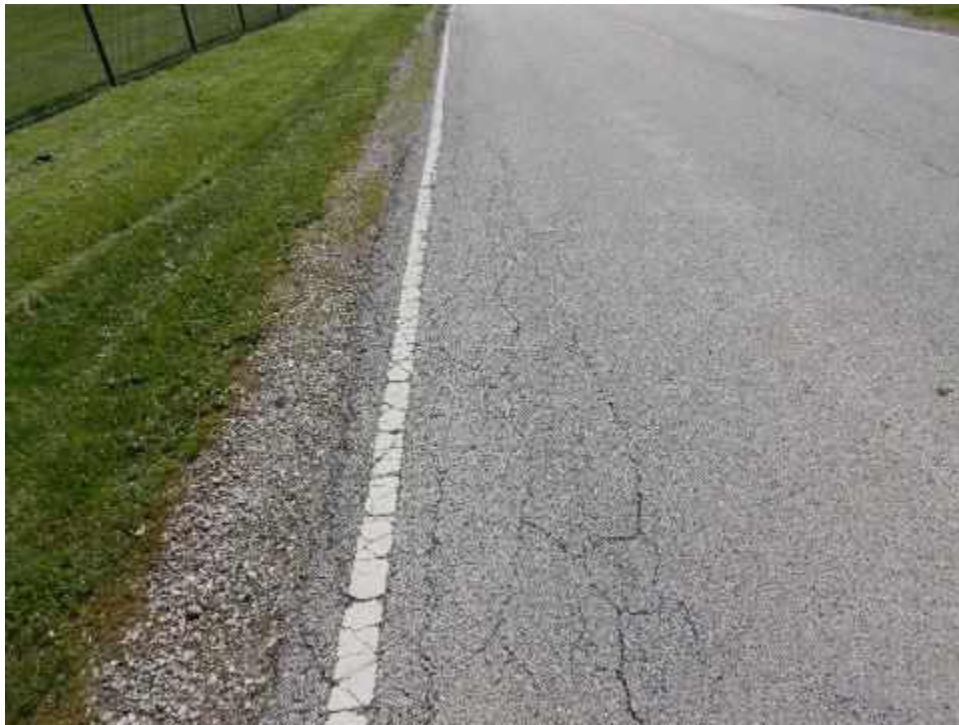
STMARR-UW09C-Alligator Cracking-(Sample Unit No. 01)
