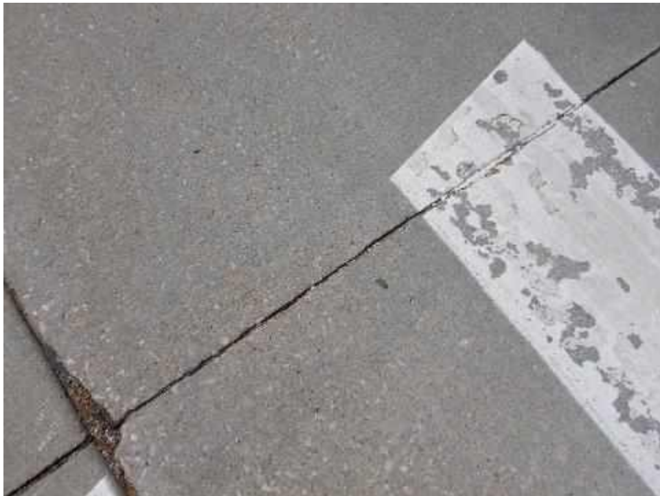
STADMD-E00D-Joint Spalling-(Sample Unit No. 01)
