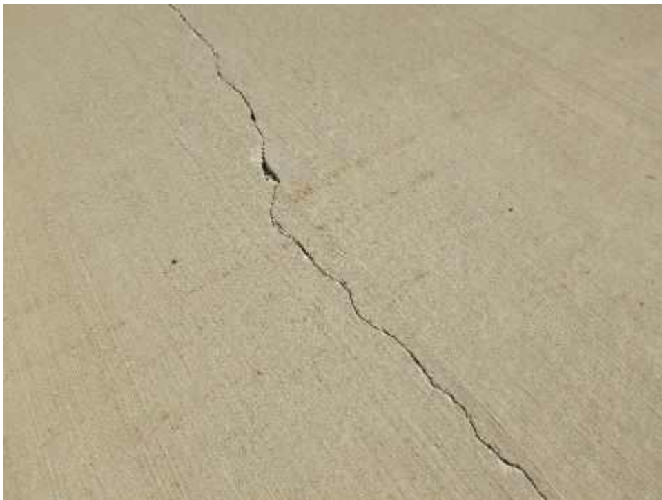
GERTYD-E00D-LTD Cracking-(Sample Unit No. 01)
