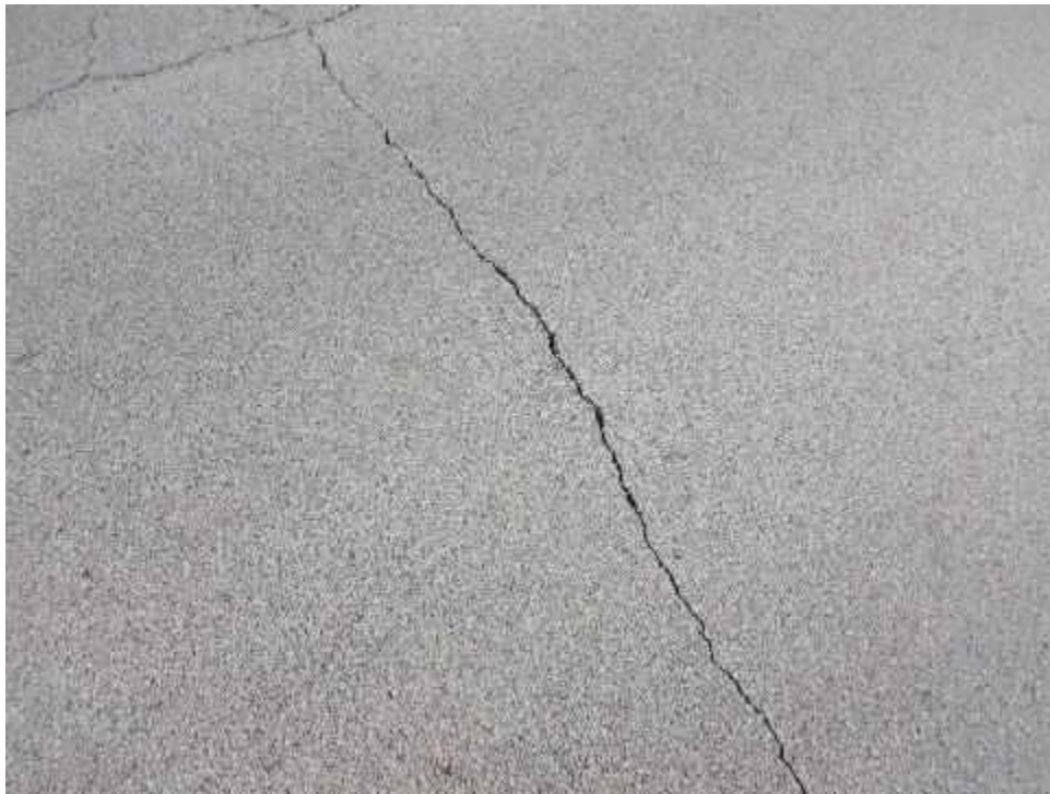
STMARR-UW12-L&T Cracking-(Sample Unit No. 01)
