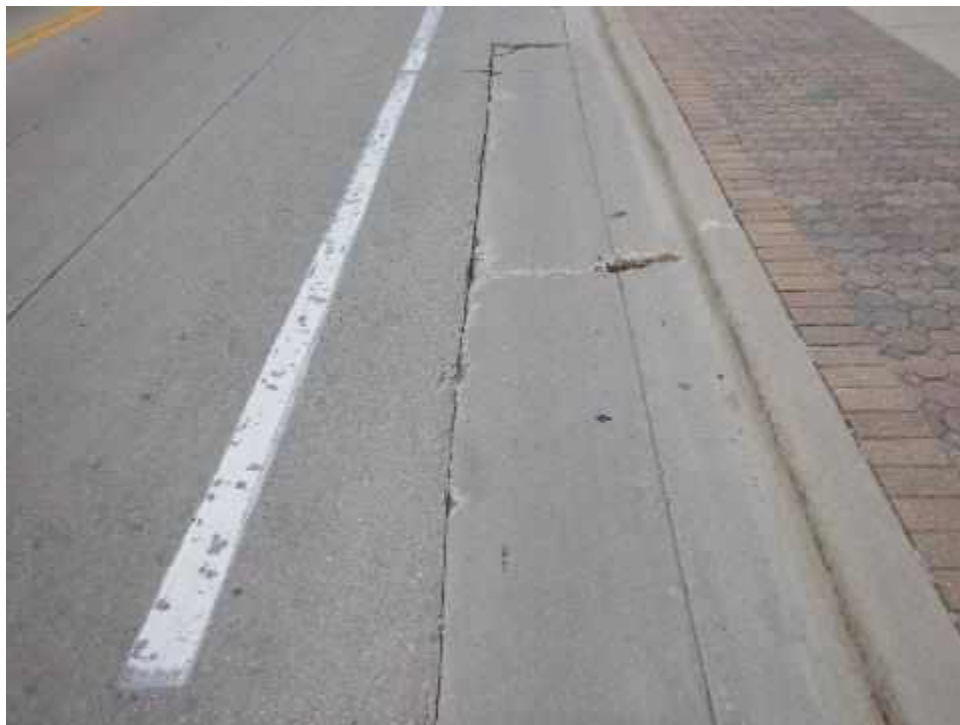
GREGYD-UW12D-Large Patching-(Sample Unit No. 01)
