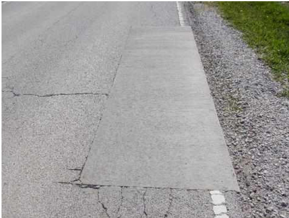
STMARR-UW09C-Patching-(Sample Unit No. 01)
