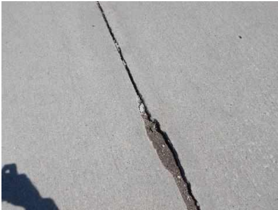
OAKS-S16-Joint Seal Damage-(Sample Unit No. 01)
