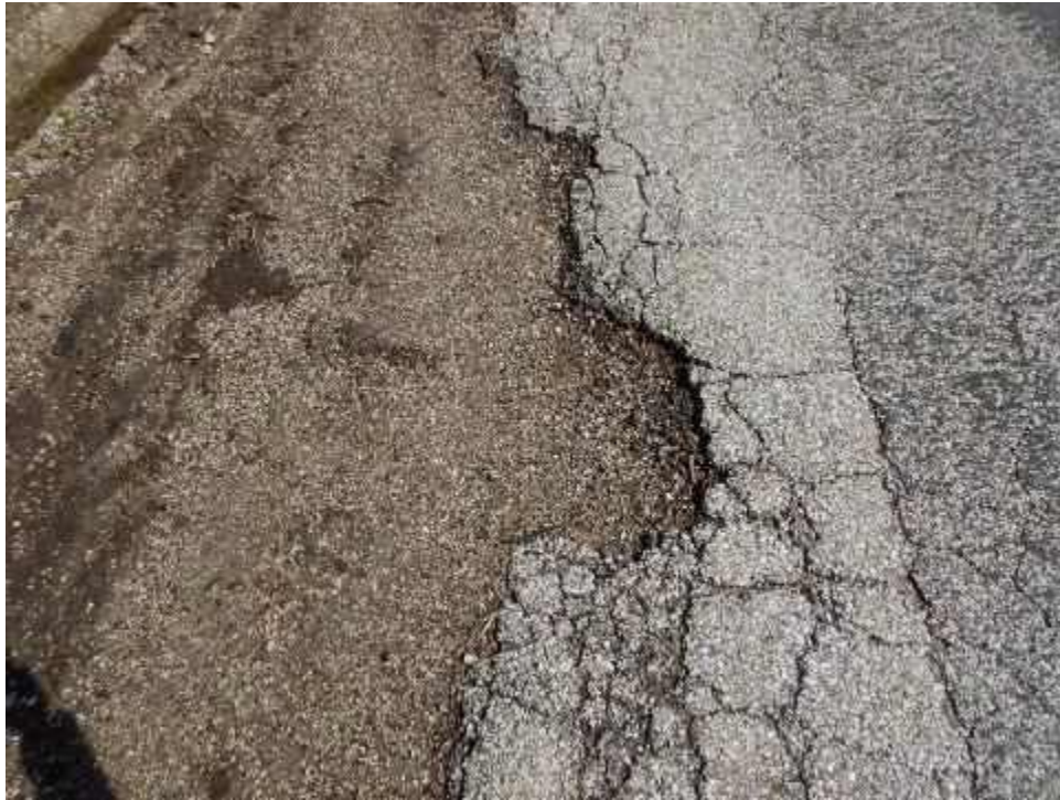
GRIFFITHD-S18-Edge Cracking-(Sample Unit No. 01)
