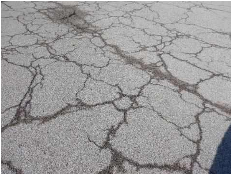
KIRKD-S20B-Block Cracking-(Sample Unit No. 01)
