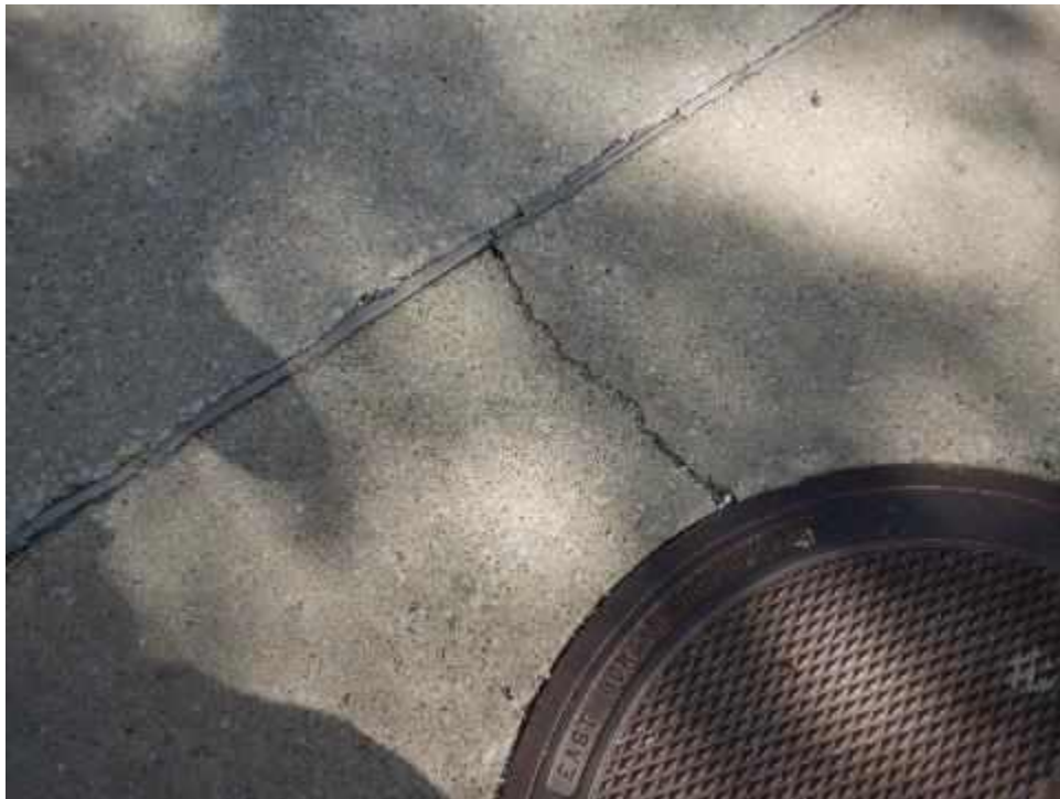
CLARKST-UW12-LTD Cracking-(Sample Unit No. 01)
