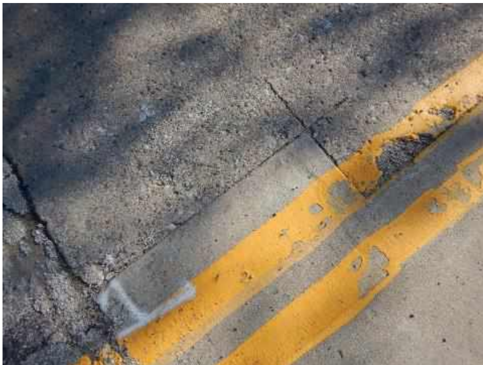
STMARR-E00B-Small Patching-(Sample Unit No. 01)
