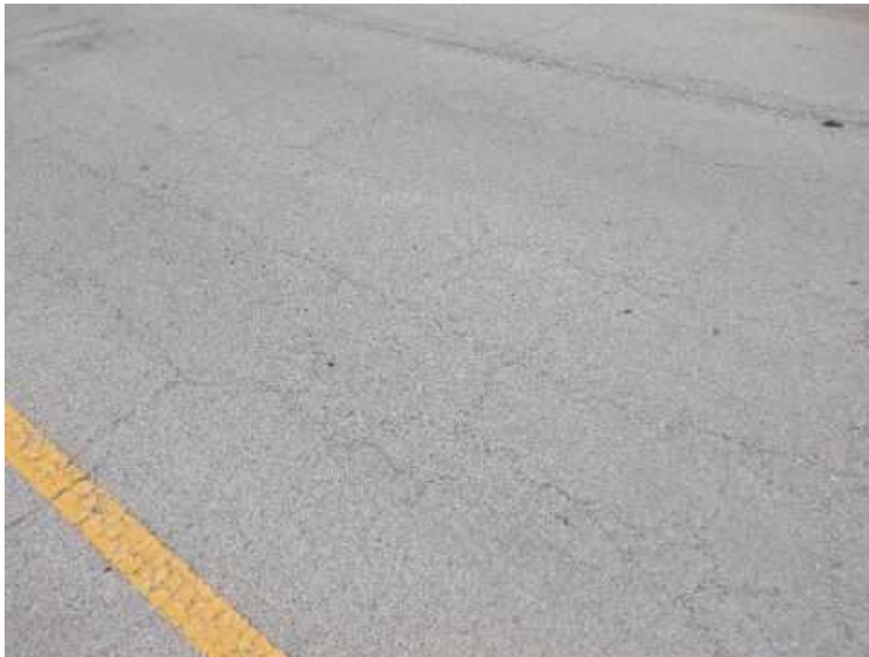
PENSYA-UW09A-Block Cracking-(Sample Unit No. 01)
