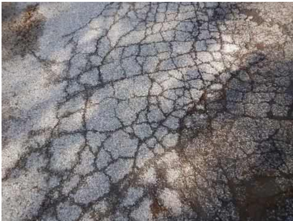
KIRKD-S20B-Alligator Cracking-(Sample Unit No. 01)
