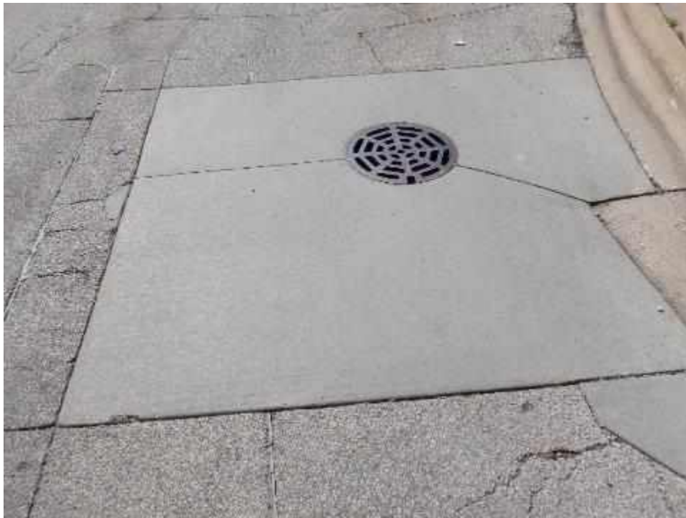
STADMD-E00A-Patching-(Sample Unit No. 01)
