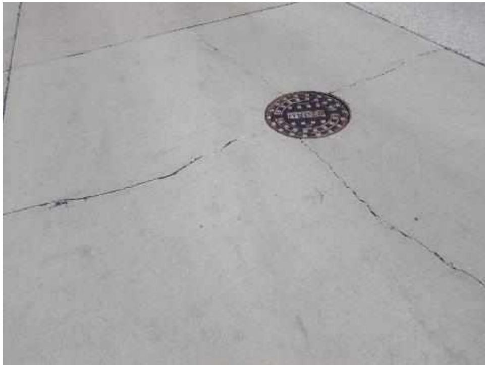
GREGYD-E02A-LTD Cracking-(Sample Unit No. 01) (2)
