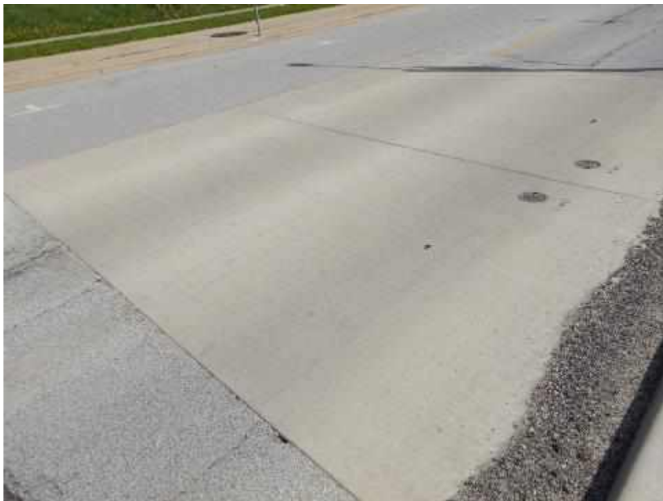
DORNRDR-US11AW-Patching-(Sample Unit No. 01)
