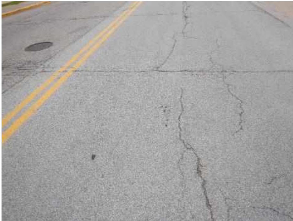
GREGYD-UW12A-Joint Reflection Cracking-(Sample Unit No. 01)
