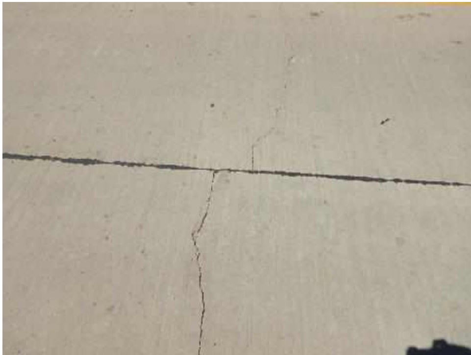
FOURTS-S16-LTD Cracking-(Sample Unit No. 01)
