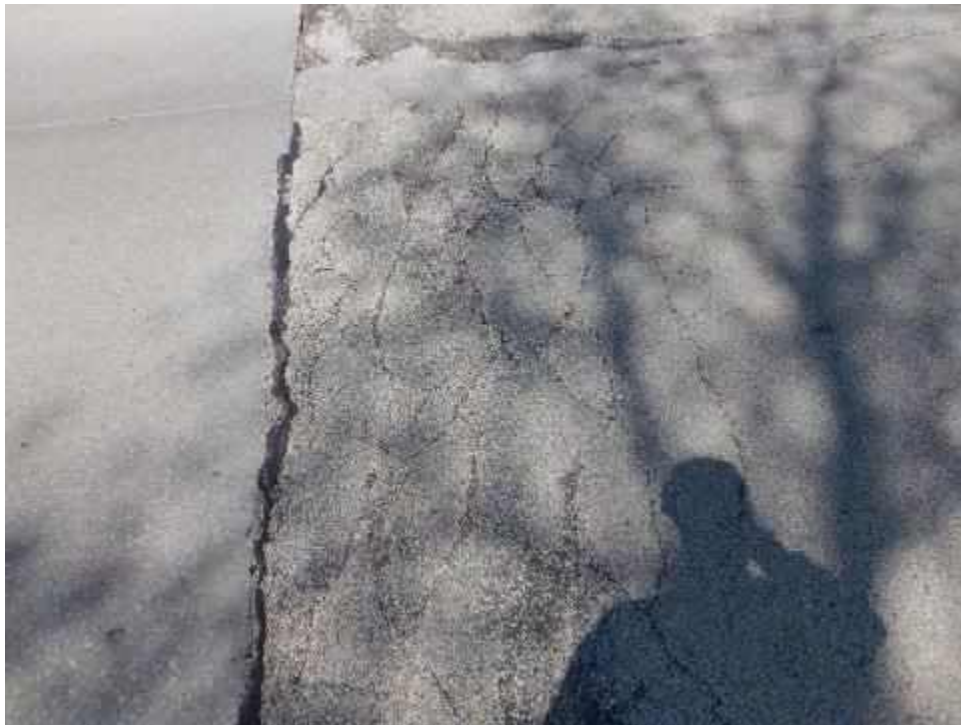
LNCLNAV-US17B-Alligator Cracking-(Sample Unit No. 01)
