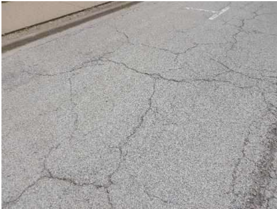
SIXTHS-S14-Block Cracking-(Sample Unit No. 01)
