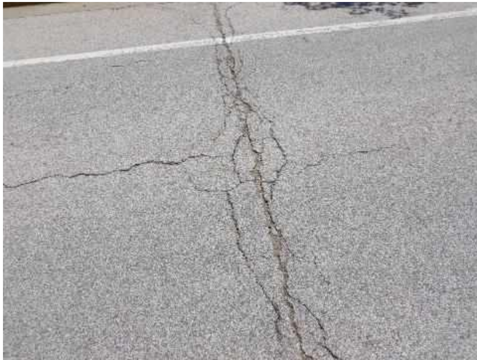
GREGYD-E01AS-Joint Reflection Cracking-(Sample Unit No. 01)
