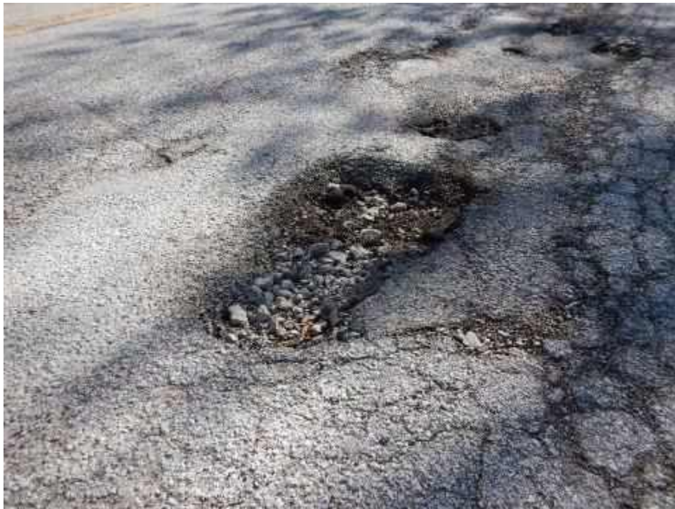
STMARR-E00D-Pothole-(Sample Unit No. 02) (1)
