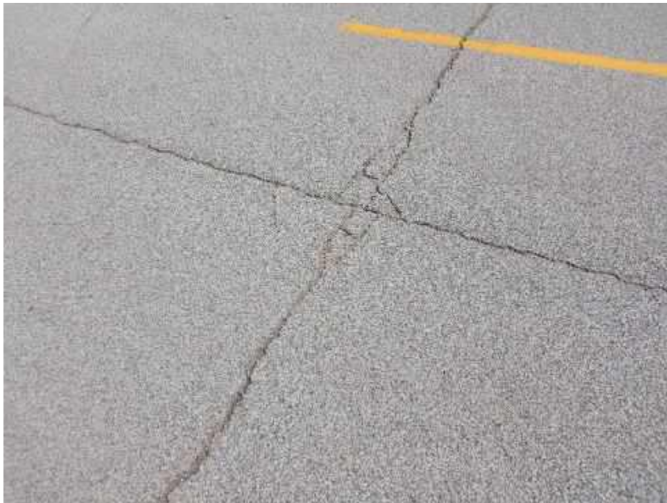
PEABYD-E03-Joint Reflection Cracking-(Sample Unit No. 01)
