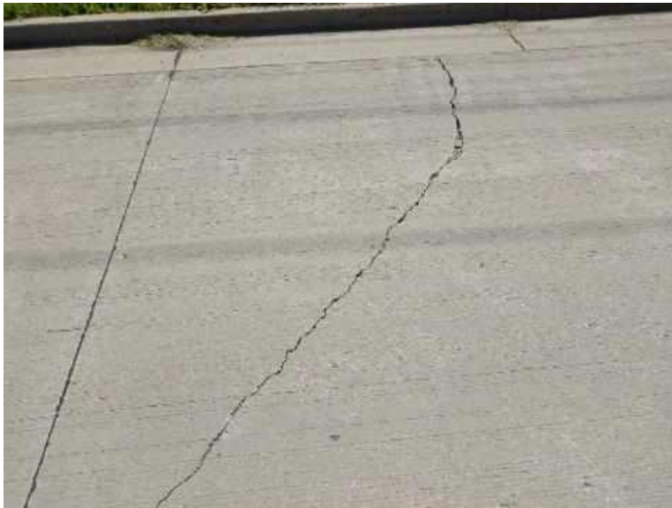
LNCLNAV-US23-LTD Cracking-(Sample Unit No. 01)
