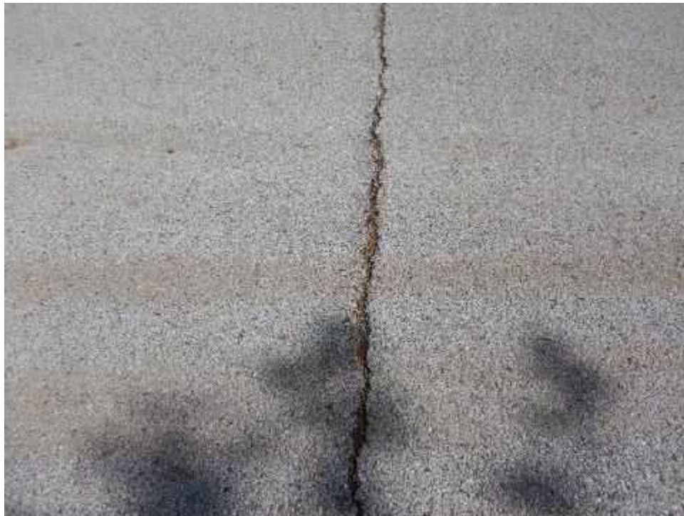
HAZELWDD-E00A-L&T Cracking-(Sample Unit No. 01)
