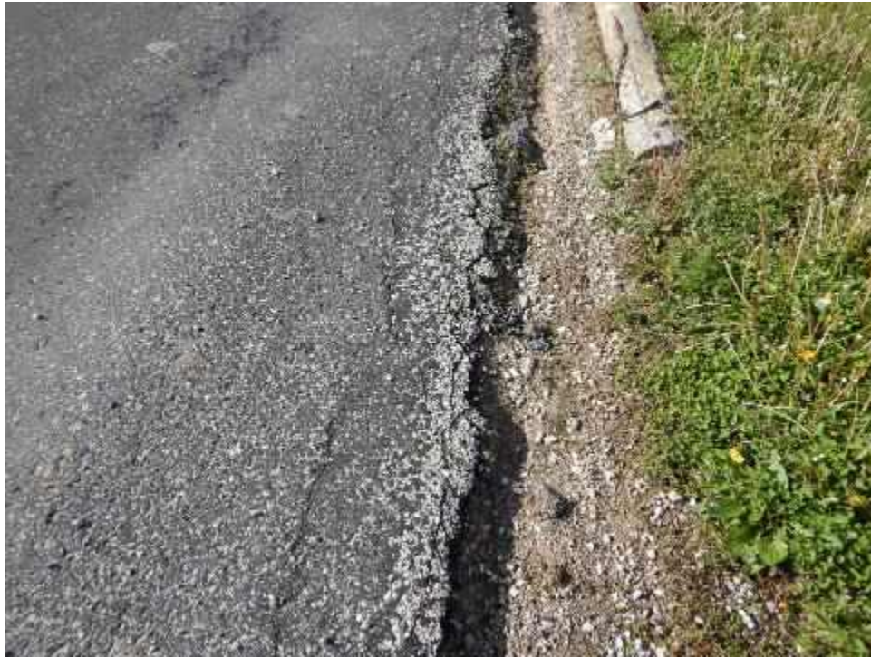
GRIFFITHD-S20-Edge Cracking-(Sample Unit No. 01)
