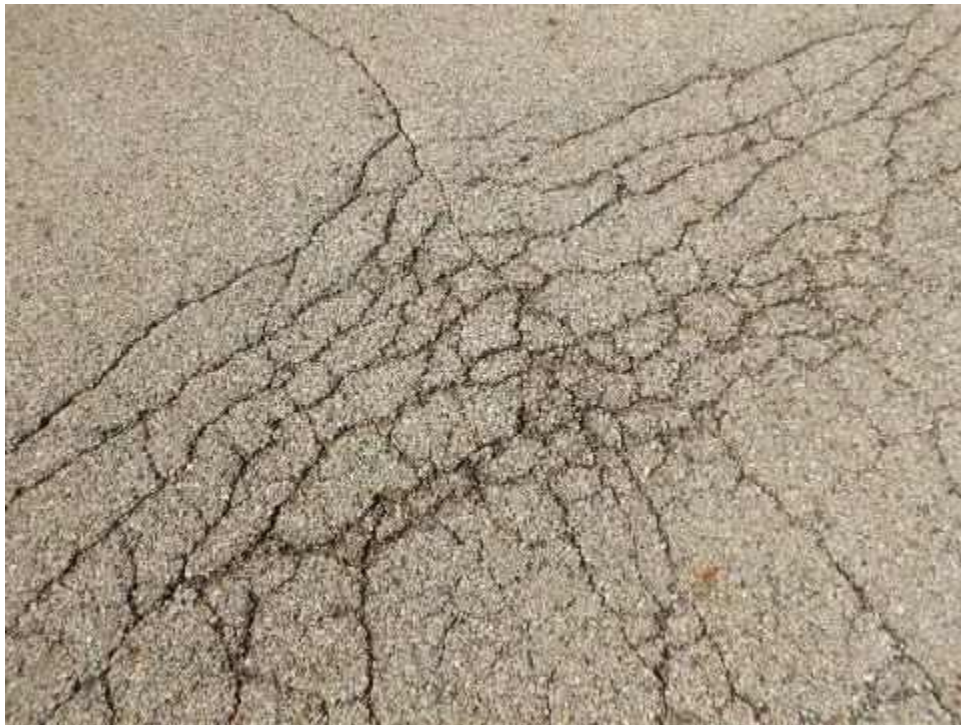
HAZELWDD-E00C-Alligator Cracking-(Sample Unit No. 02)
