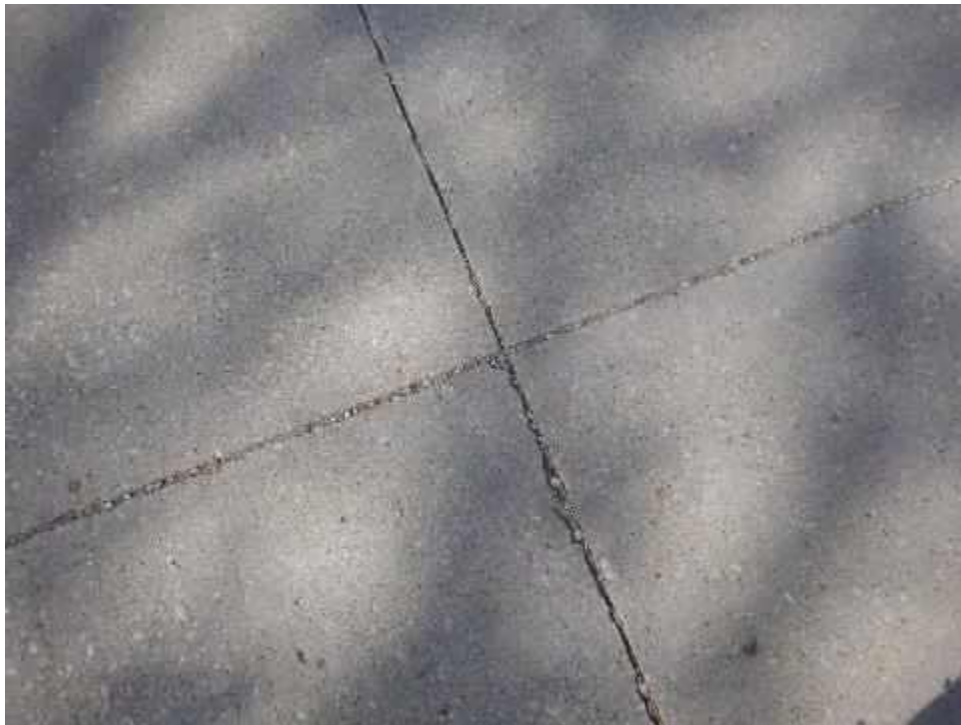
CLARKST-UW12-Joint Seal Damage-(Sample Unit No. 01)
