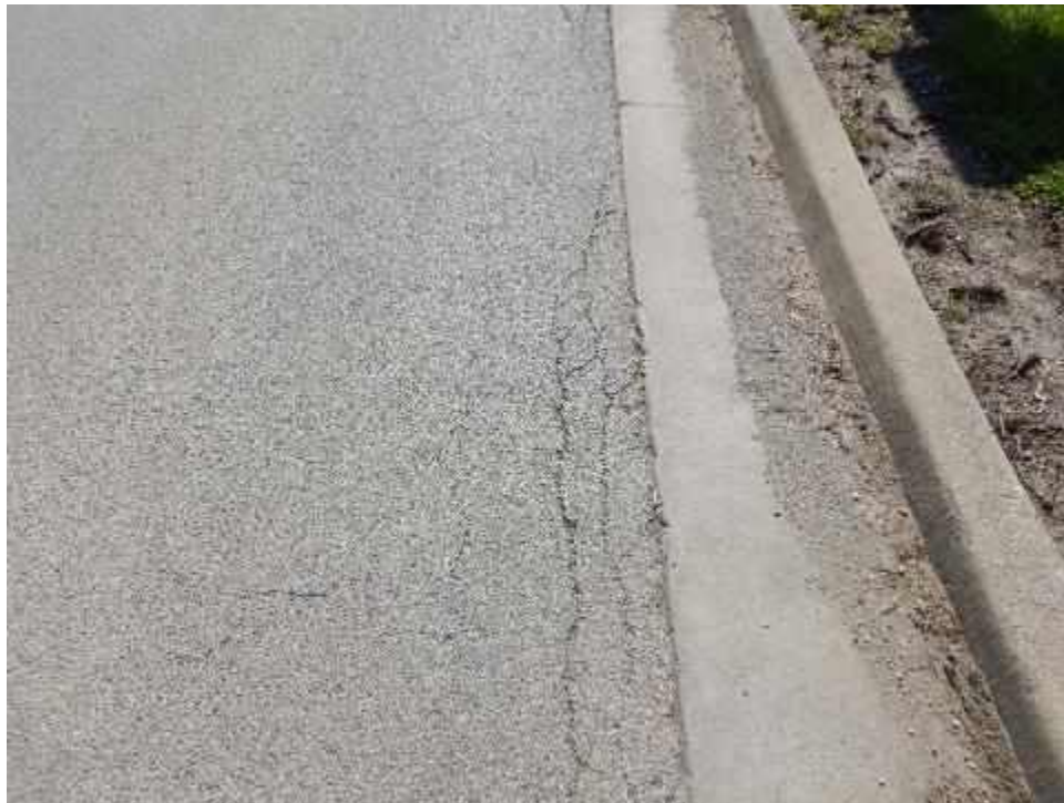
STMARR-E04A-Edge Cracking-(Sample Unit No. 01)
