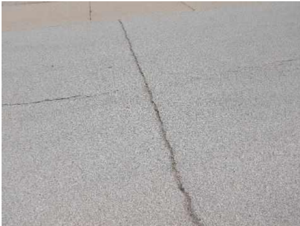
VRGNADR-US14BW-Joint Reflection Cracking-(Sample Unit No. 01)
