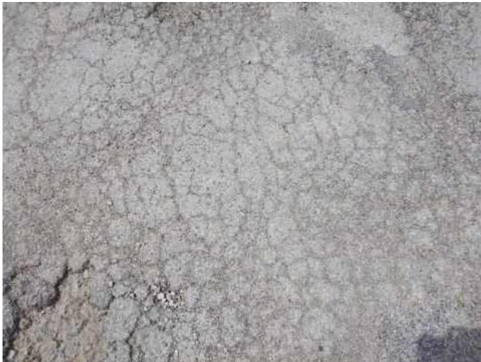
PENSYA-UW09A-Alligator Cracking-(Sample Unit No. 01)
