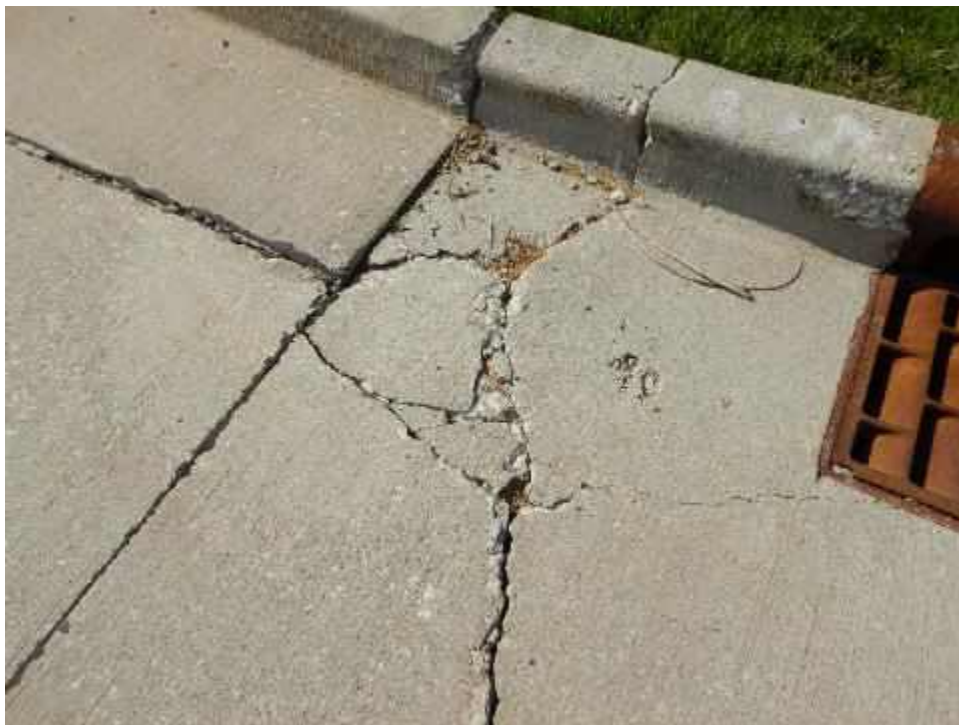
HAZELWDD-E01B-Corner Spalling-(Sample Unit No. 01)
