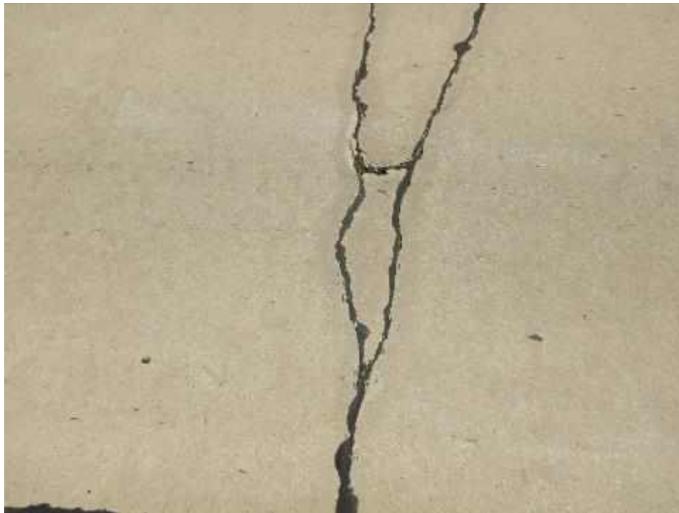
GREGYD-E02A-Shattered Slab-(Sample Unit No. 01)
