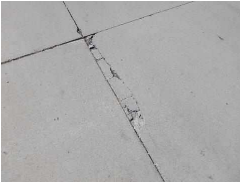
OAKS-S10C-Joint Spalling-(Sample Unit No. 01)
