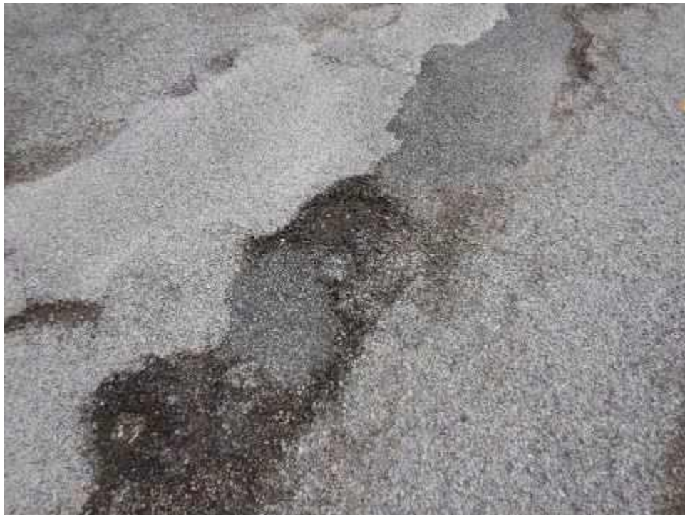
PENSYA-UW11B-Pothole-(Sample Unit No. 02)
