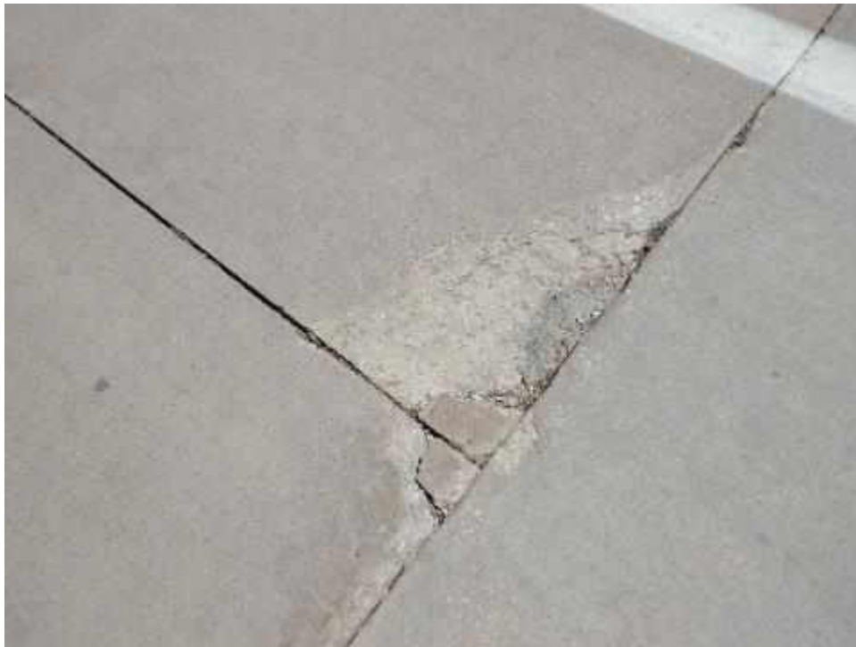
ARMRYA-E04-Corner Spalling-(Sample Unit No. 01)
