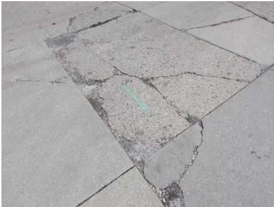
OAKS-S10A-Large Patching-(Sample Unit No. 01)
