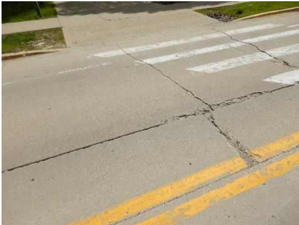
GREGYD-UW12B-Shattered Slab-(Sample Unit No. 01)
