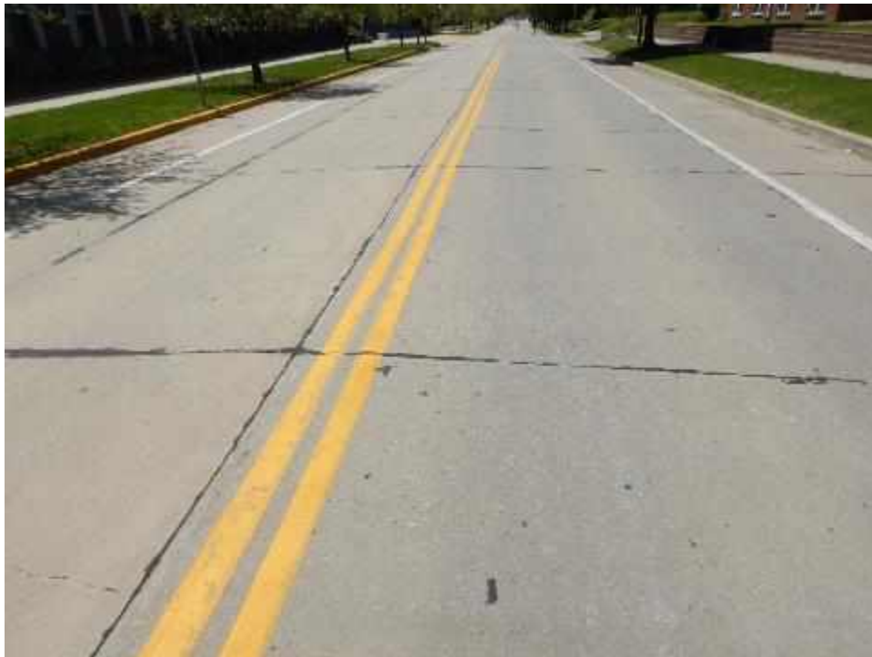
GREGYD-E03A-LTD Cracking-(Sample Unit No. 01)
