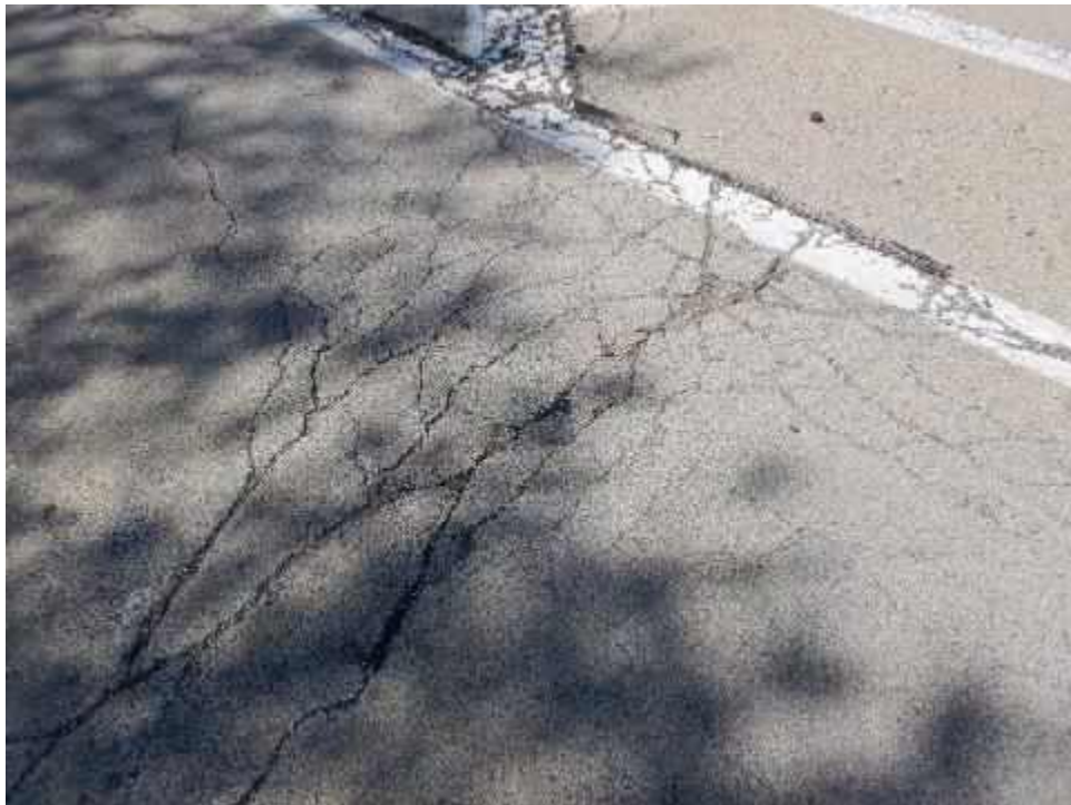
LNCLNAV-US17B-Alligator Cracking-(Sample Unit No. 02)
