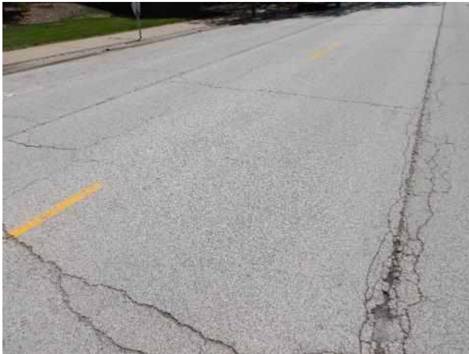
SIXTHS-S13-Joint Reflection Cracking-(Sample Unit No. 01)
