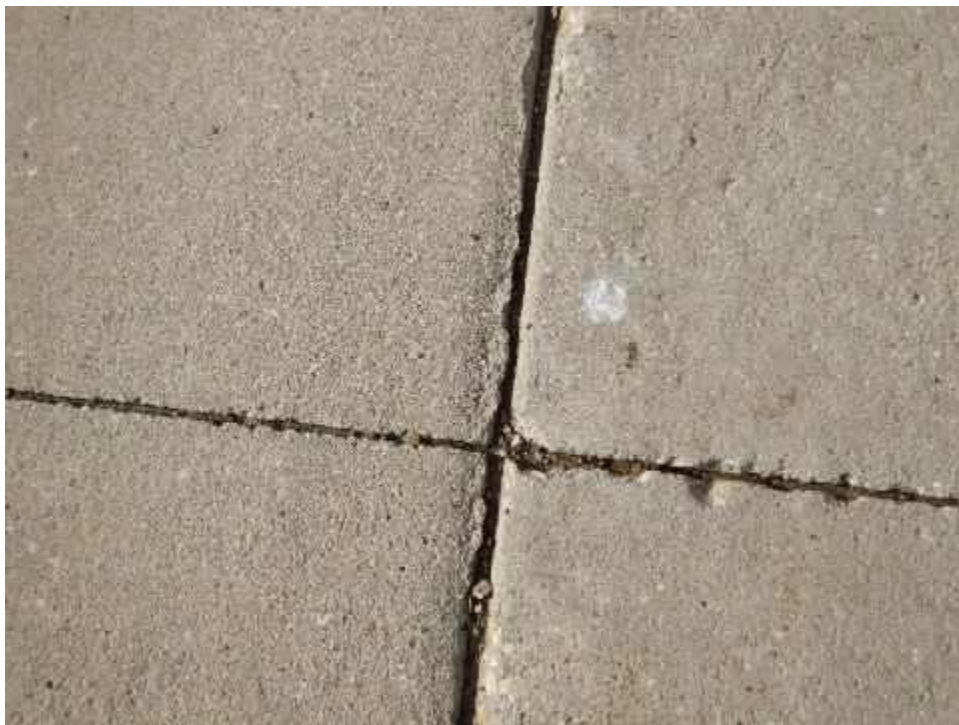
GRIFFITHD-S22C-Joint Seal Damage-(Sample Unit No. 01)
