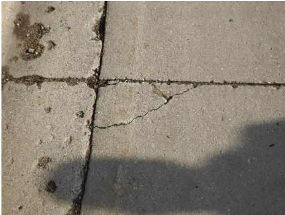
GRIFFITHD-S22B-Corner Spalling-(Sample Unit No. 01)
