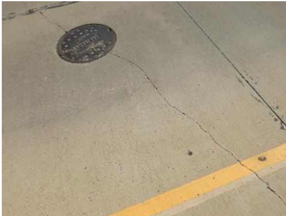
STADMD-E00B-LTD Cracking-(Sample Unit No. 01)
