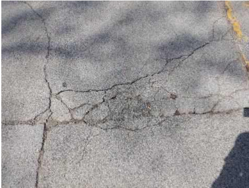
DORNRDR-US13W-Alligator Cracking-(Sample Unit No. 01)
