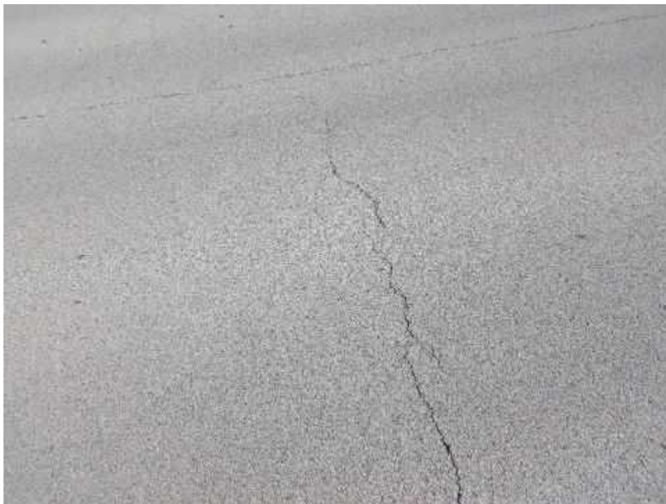
STMARR-UW09B-L&T Cracking-(Sample Unit No. 01)
