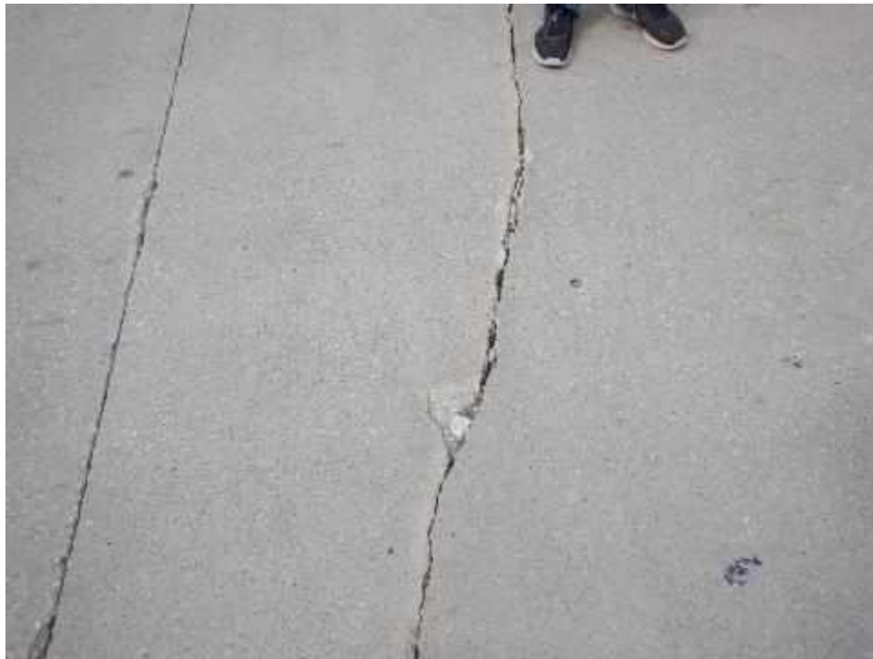
GREGYD-UW12D-LTD Cracking-(Sample Unit No. 01)
