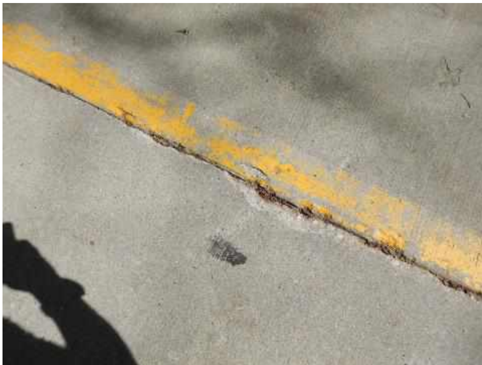
PEABYD-E04A-Joint Seal Damage-(Sample Unit No. 01)
