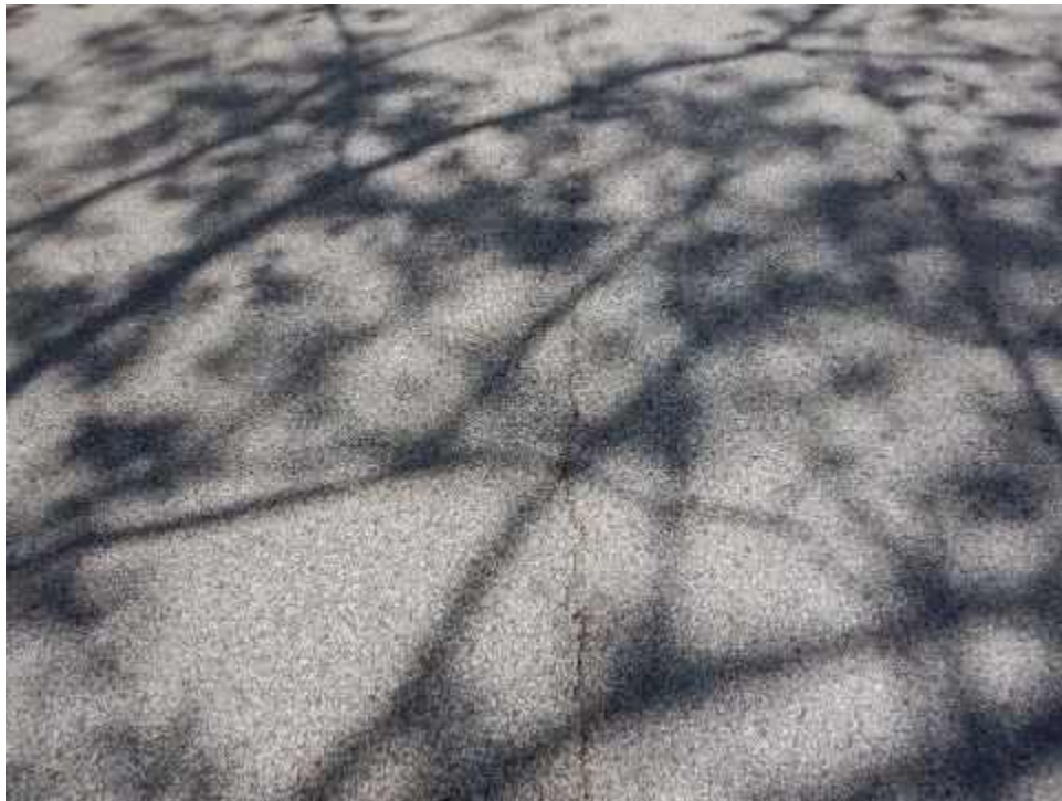
GHUFFDR-UW04S-L&T Cracking-(Sample Unit No. 01)
