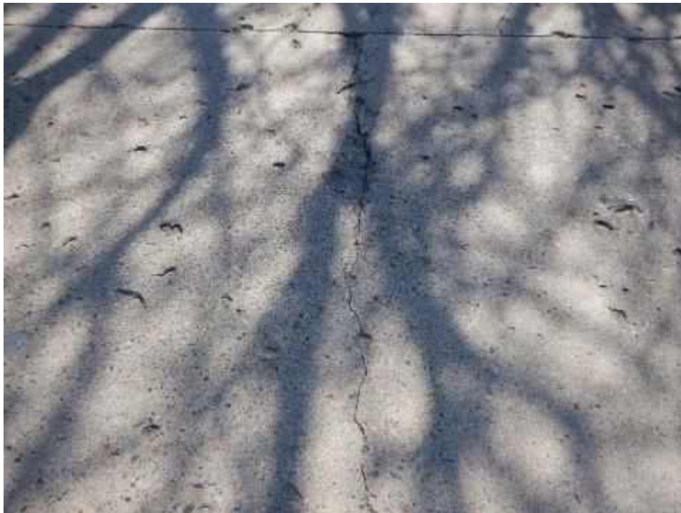
LNCLNAV-US19-LTD Cracking-(Sample Unit No. 01)
