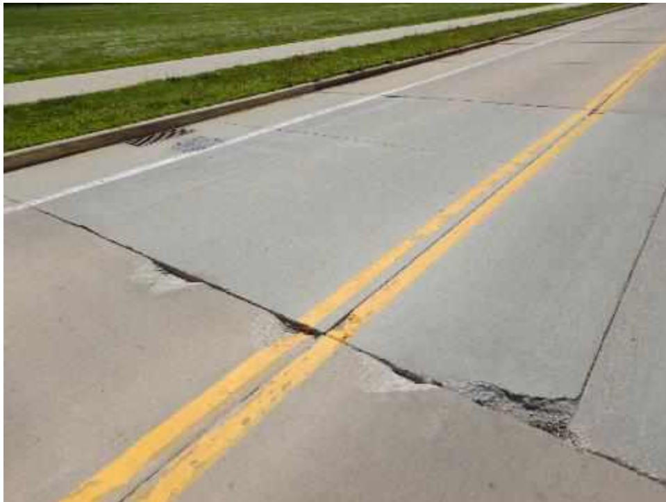
GREGYD-UW12C-Large Patching-(Sample Unit No. 01)
