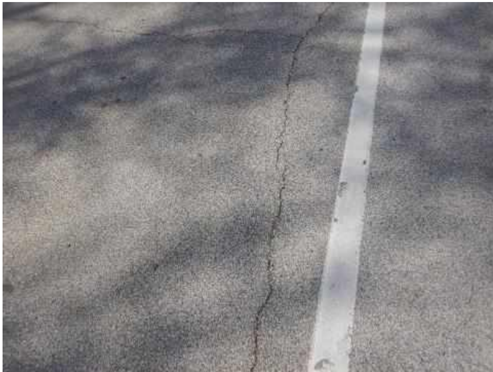
DORNRDR-US13W-L&T Cracking-(Sample Unit No. 01)
