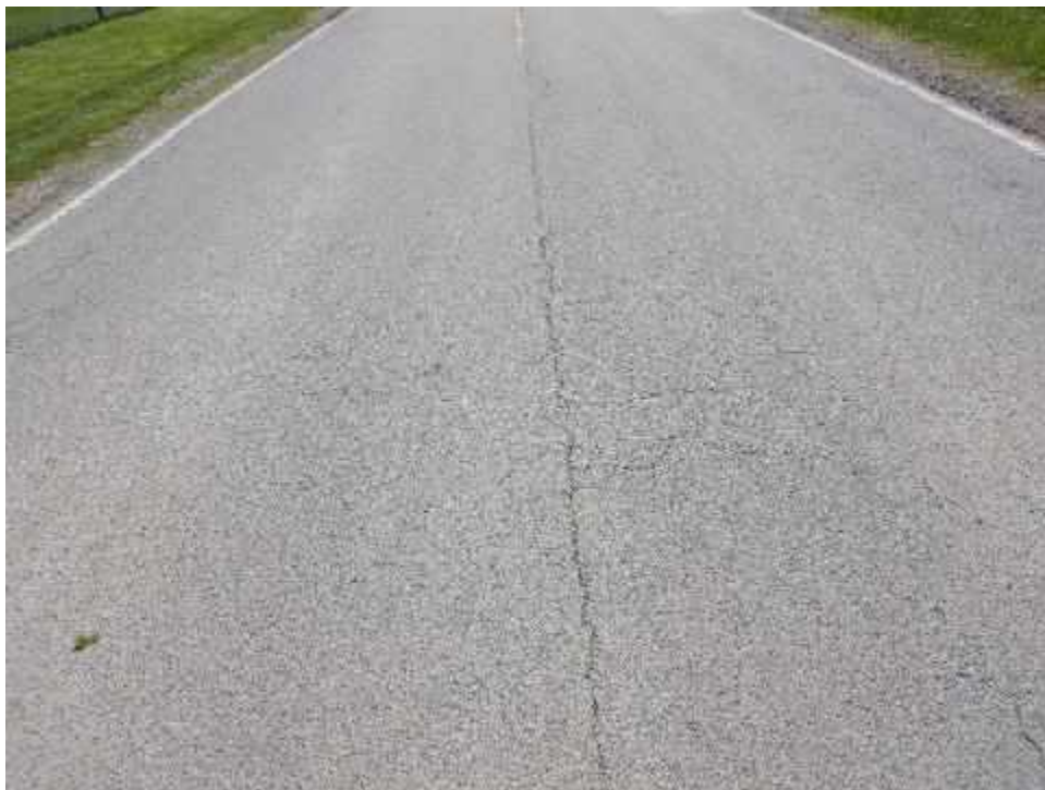
STMARR-UW09C-L&T Cracking-(Sample Unit No. 01)
