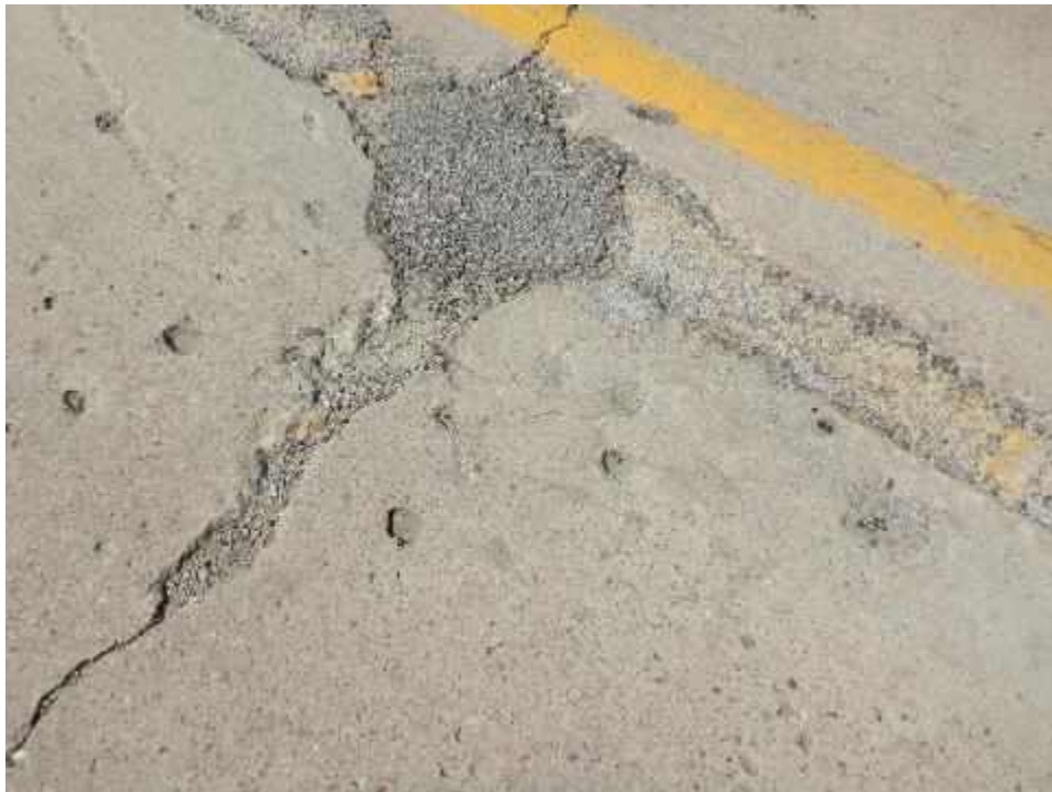
LNCLNAV-US17A-Durability Cracking-(Sample Unit No. 01)
