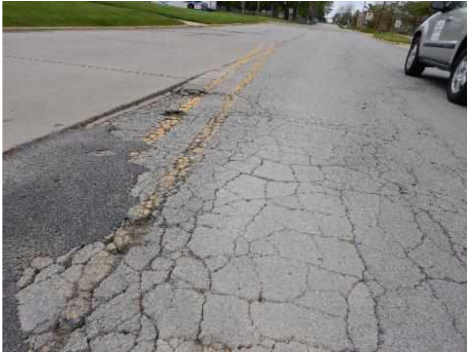
PENSYA-UW11A-Rutting-(Sample Unit No. 01)
