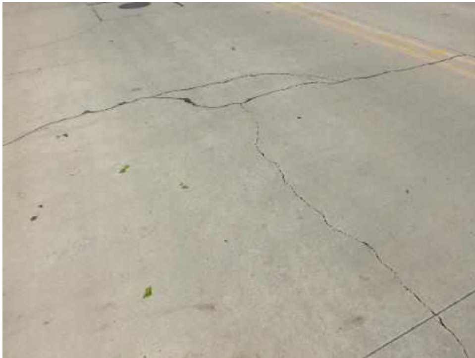
GREGYD-E00-Shattered Slab-(Sample Unit No. 01)
