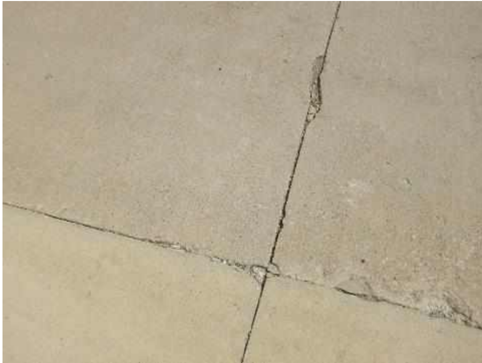
PEABYD-UW11-Joint Seal Damage-(Sample Unit No. 01)
