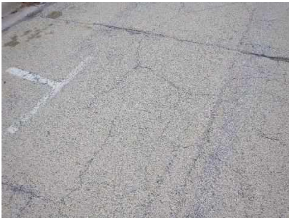
STOUGS-UW13-Block Cracking-(Sample Unit No. 02)
