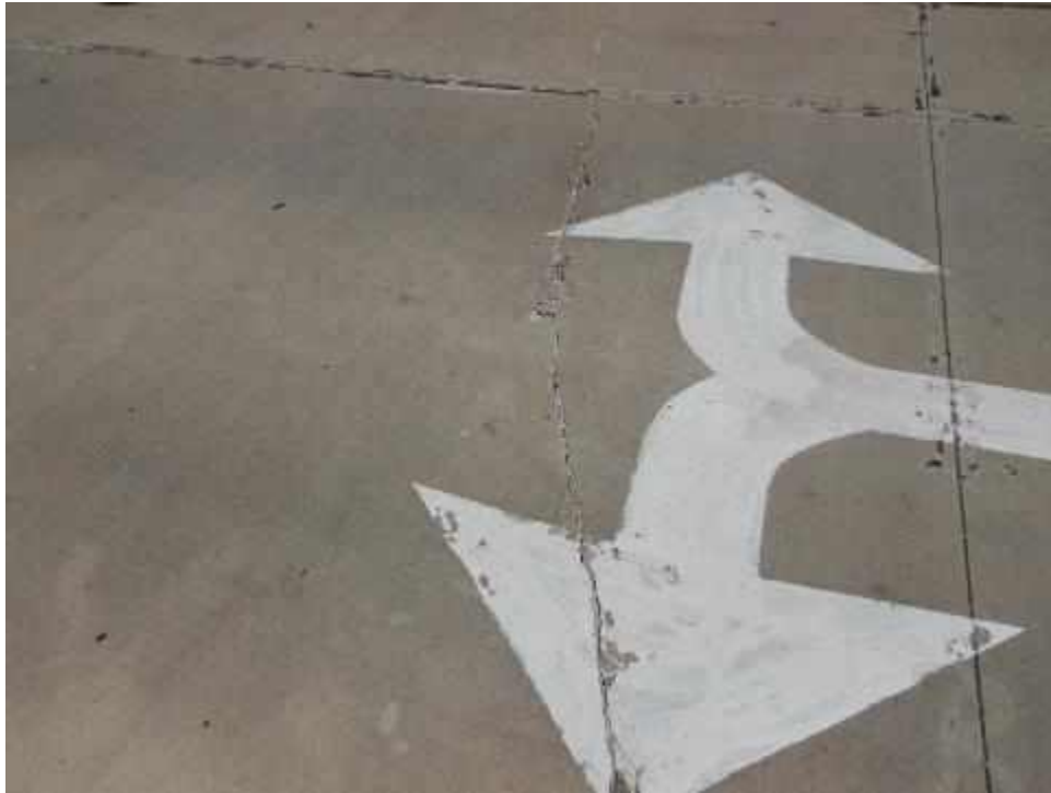
SIXTHS-S10-LTD Cracking-(Sample Unit No. 01)
