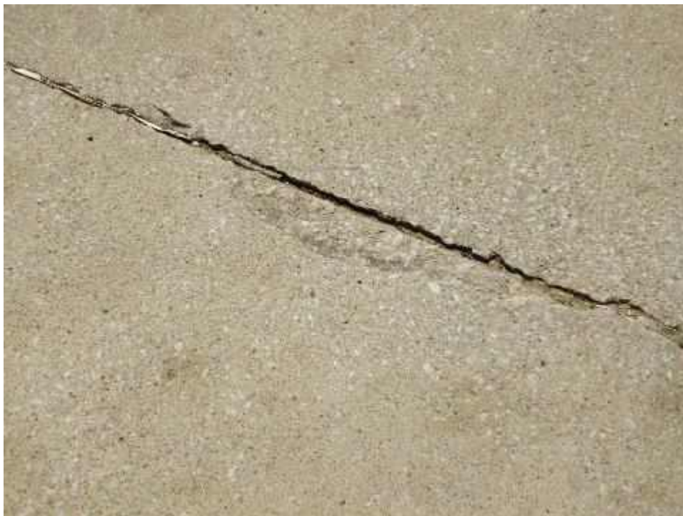
STADMD-E00E-Joint Spalling-(Sample Unit No. 01)
