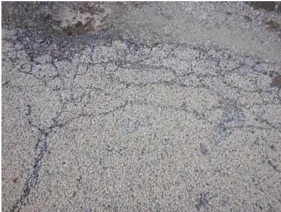
STOUGS-UW13-Alligator Cracking-(Sample Unit No. 02)
