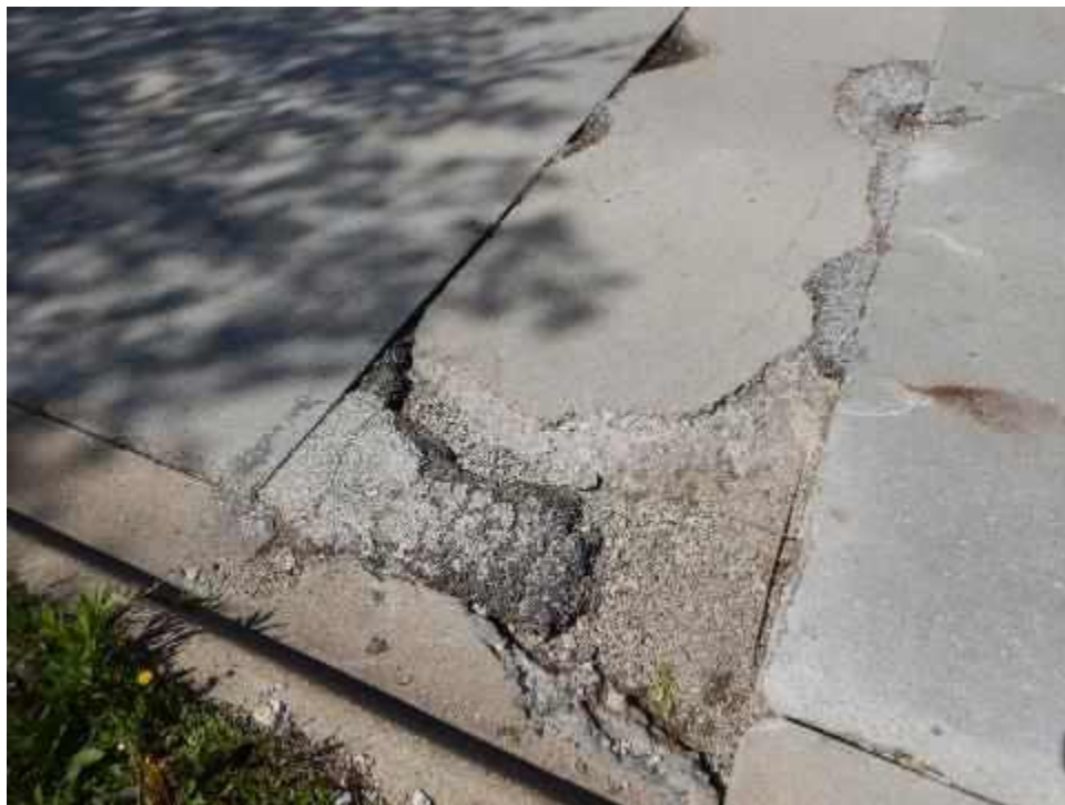
OAKS-S16-Large Patching-(Sample Unit No. 004)
