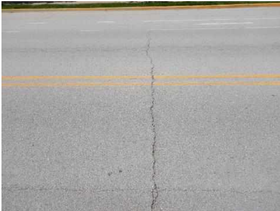
FOURTS-S12-Joint Reflection Cracking-(Sample Unit No. 01)
