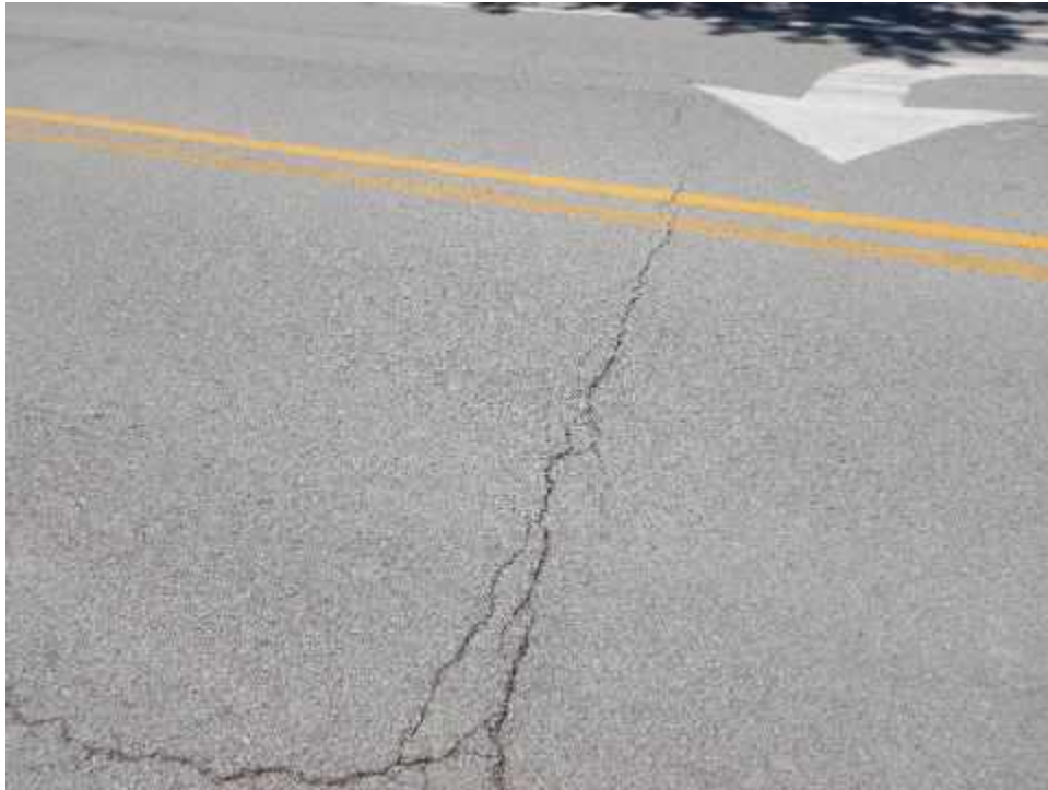
FOURTS-S11-Joint Reflection Cracking-(Sample Unit No. 01)
