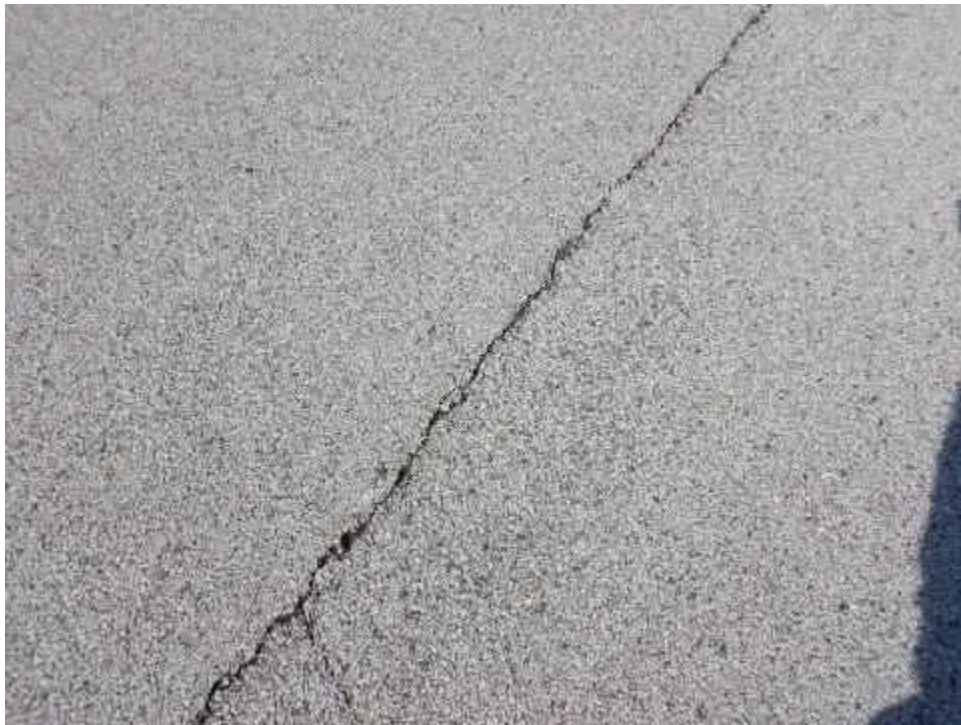
HAZELWDD-E00B-L&T Cracking-(Sample Unit No. 01)
