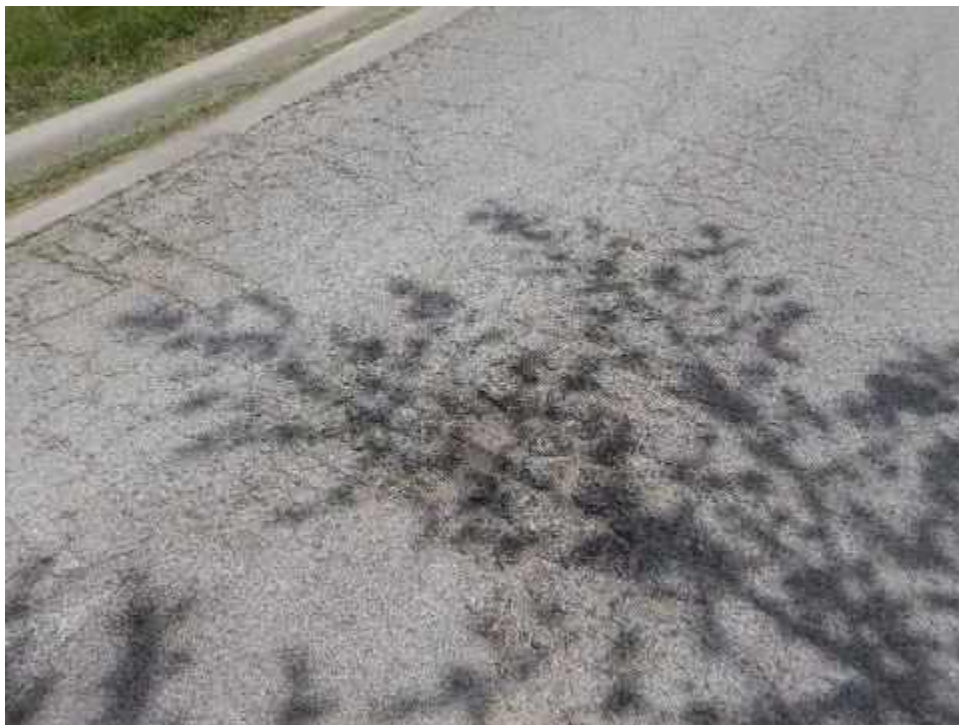
COLAGCT-UW09CS-Alligator Cracking-(Sample Unit No. 01)
