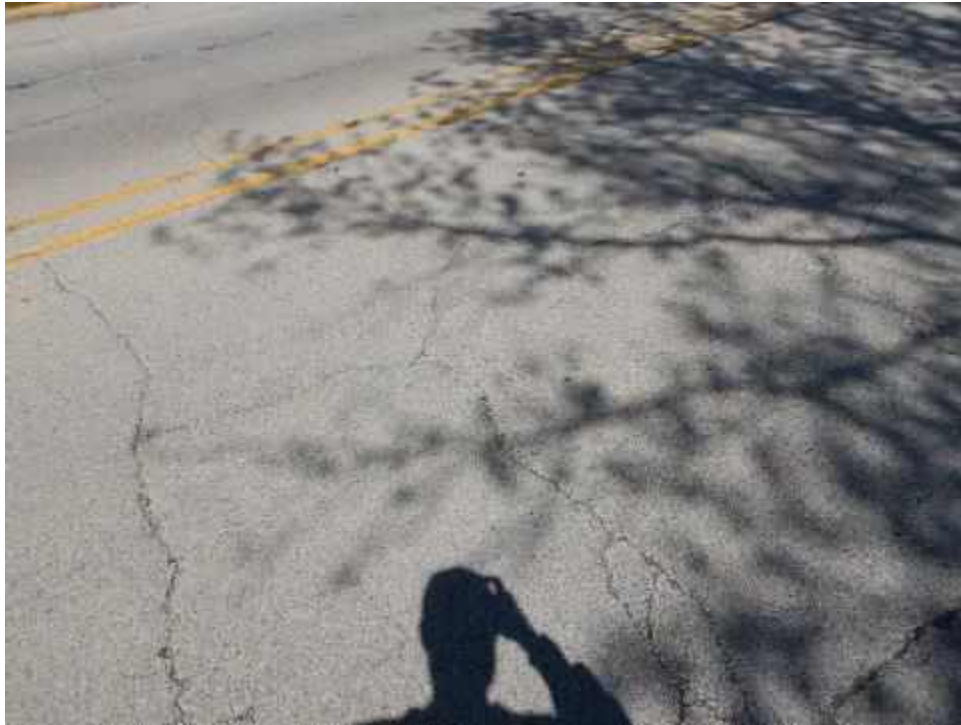
LNCLNAV-US17B-Block Cracking-(Sample Unit No. 01)
