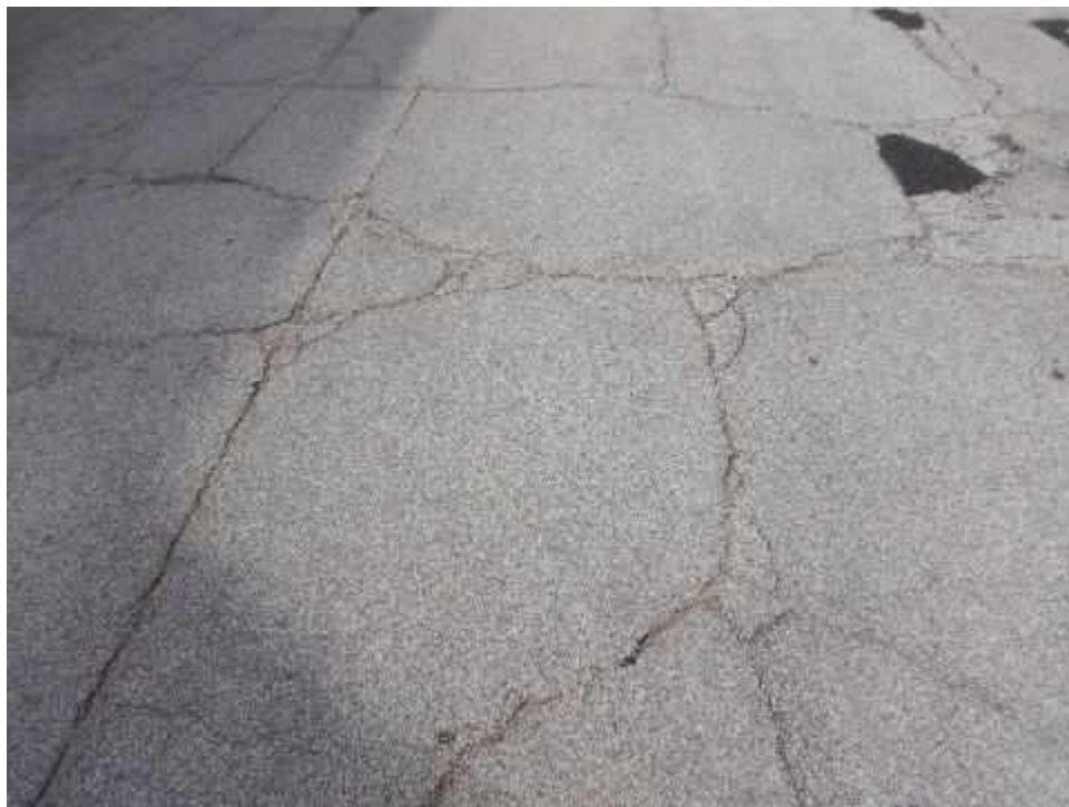
GRGRYST-US05-Block Cracking-(Sample Unit No. 01)
