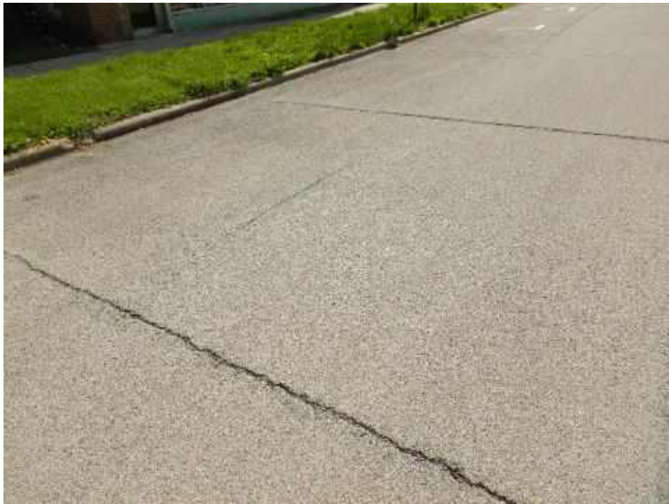
MAINS-UW11AS-Joint Reflection Cracking-(Sample Unit No. 01)
