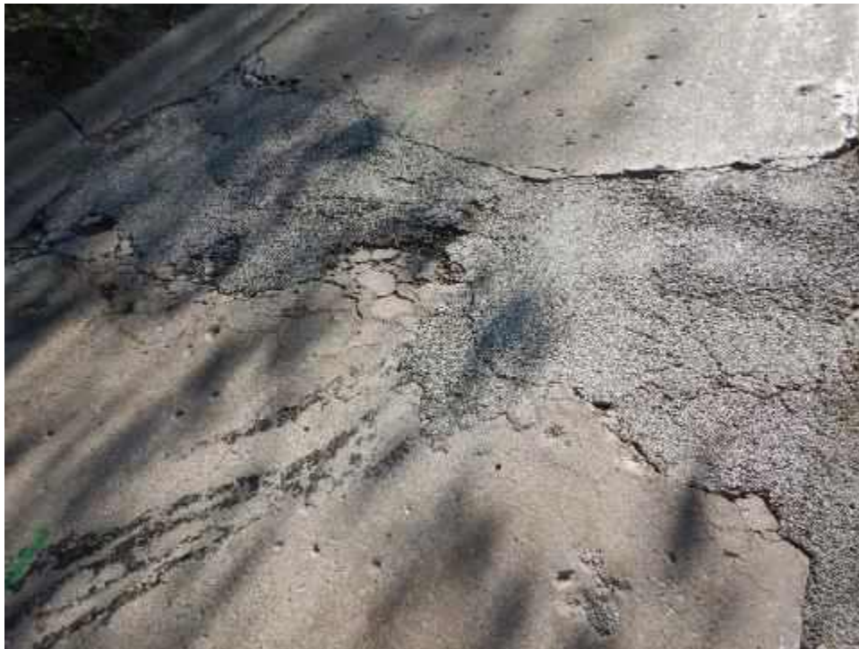
STMARR-E00B-Durability Cracking-(Sample Unit No. 01)
