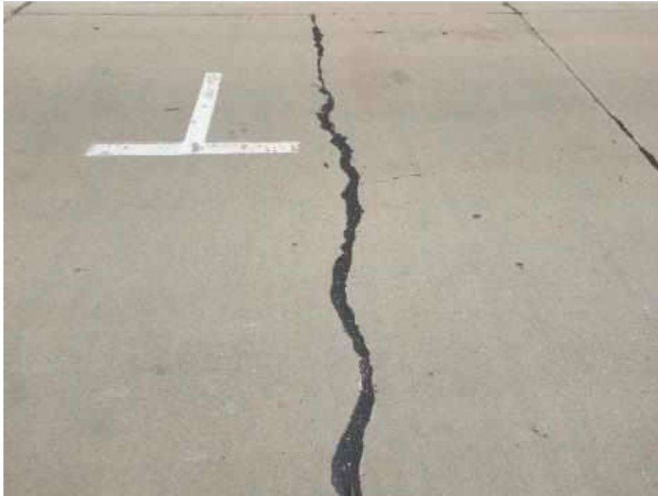
MRYLNDDR-US14-LTD Cracking-(Sample Unit No. 01)
