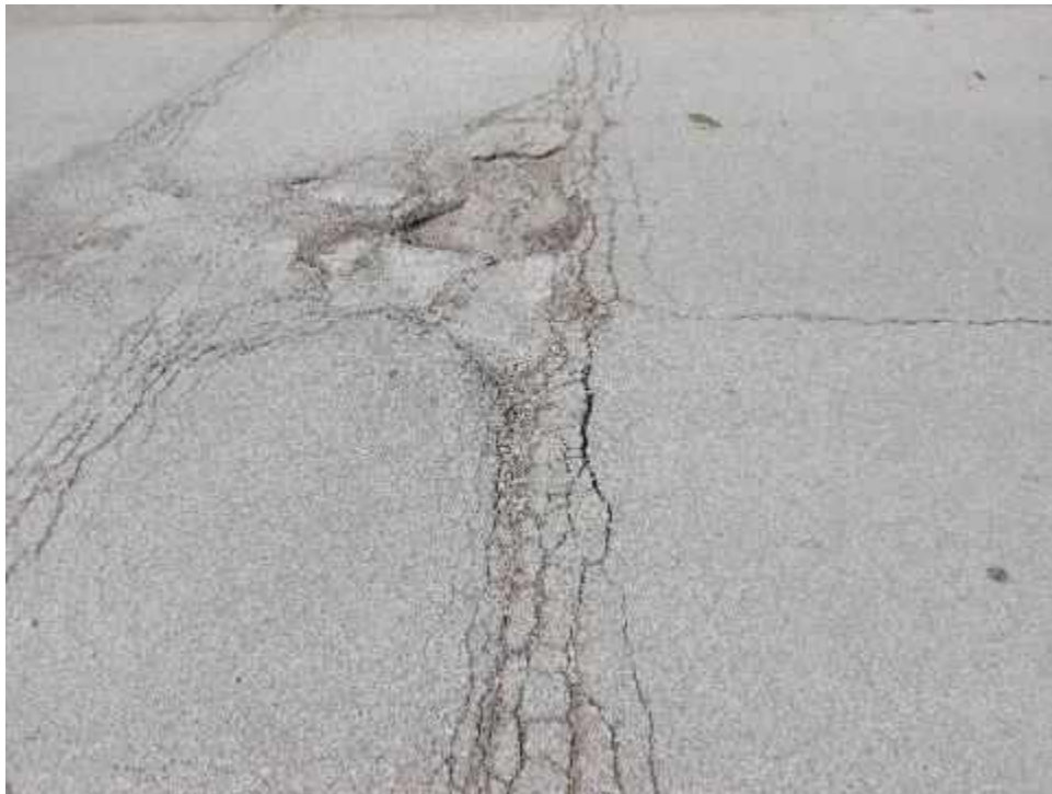
PEABYD-E01A-Joint Reflection Cracking-(Sample Unit No. 01)
