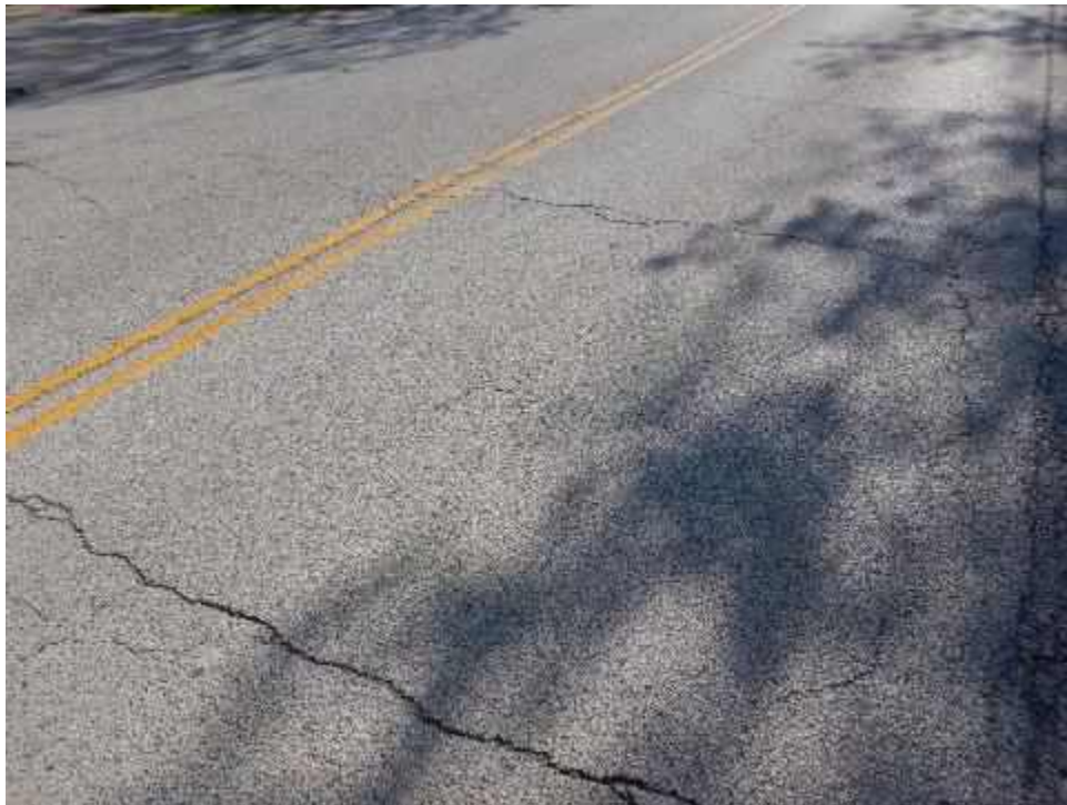
STMARR-E00C-Joint Reflection Cracking-(Sample Unit No. 01)
