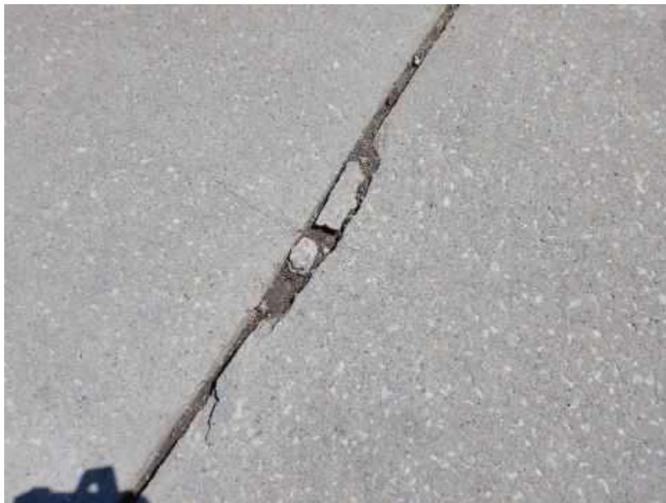
OAKS-S12-Joint Spalling-(Sample Unit No. 01)
