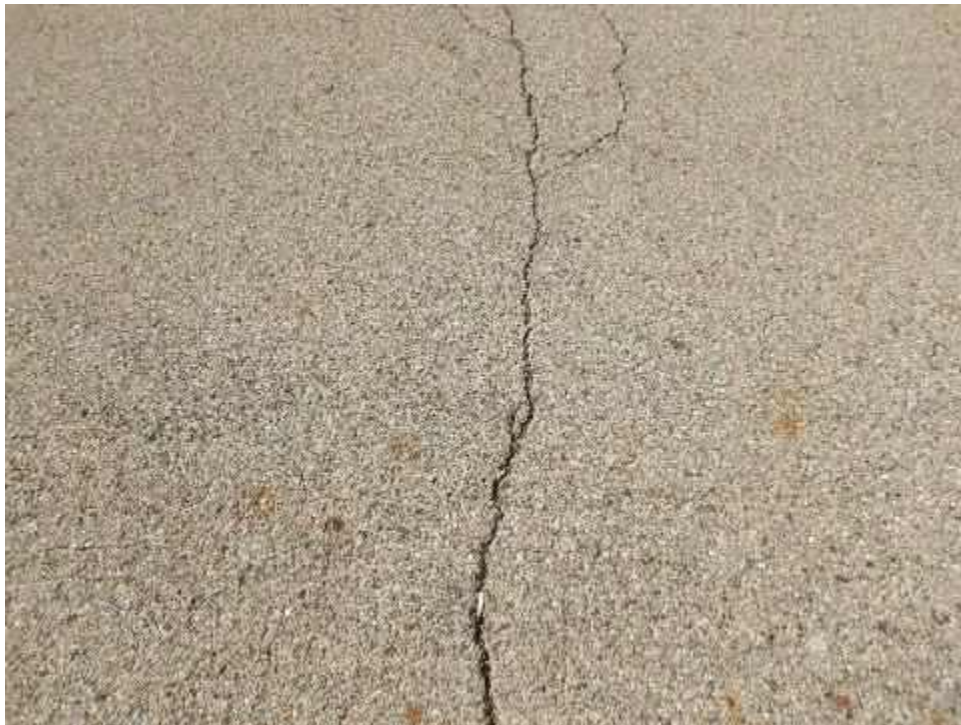
HAZELWDD-E00C-L&T Cracking-(Sample Unit No. 02)
