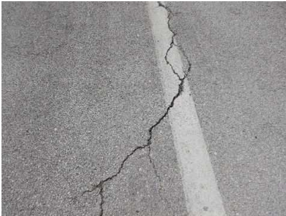
FIRSTS-S15-L&T Cracking-(Sample Unit No. 01)
