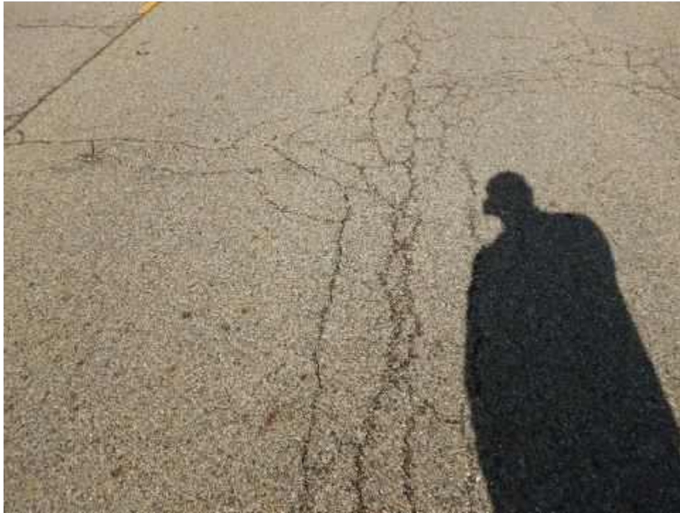
HAZELWDD-E00C-Alligator Cracking-(Sample Unit No. 01)
