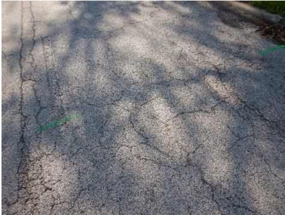
STMARR-E00C-Block Cracking-(Sample Unit No. 01)
