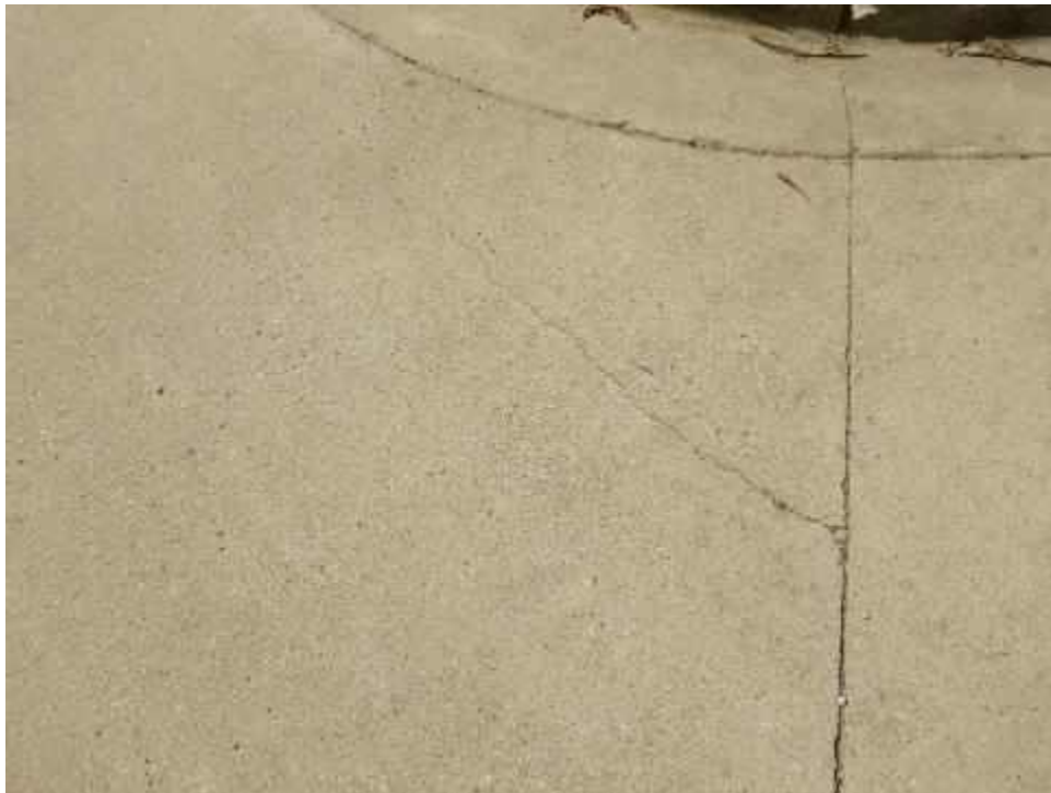
CLARKST-UW12-Shrinkage Cracking-(Sample Unit No. 01)
