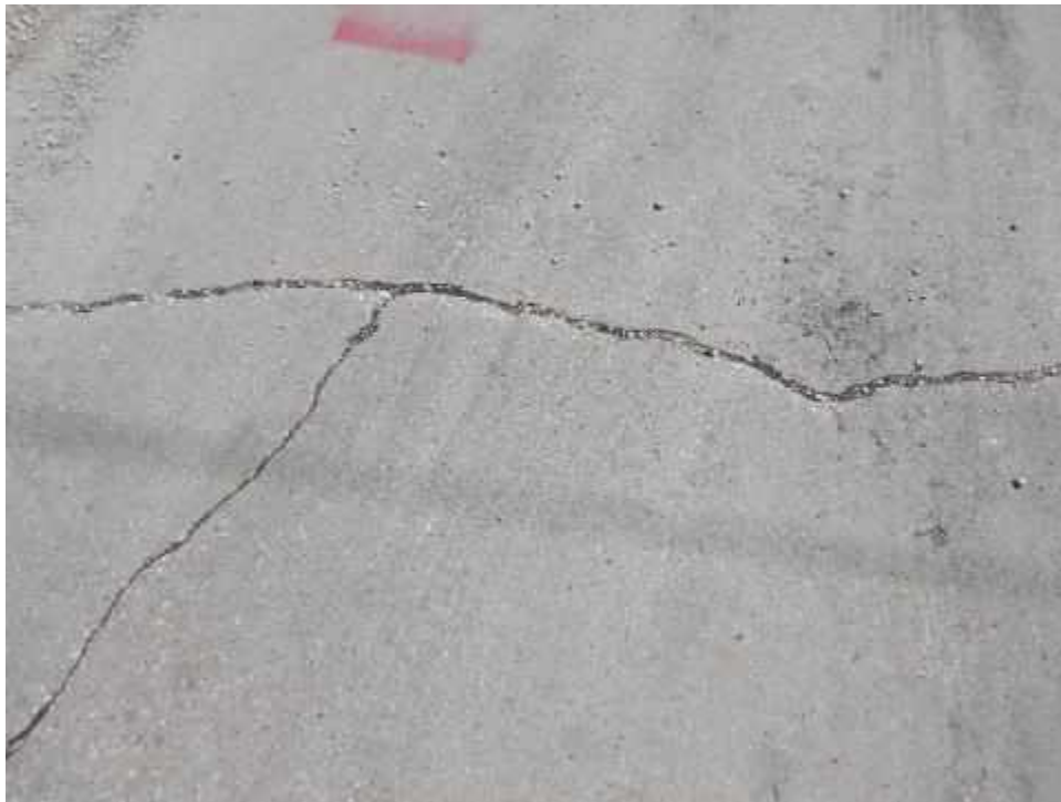
ARMRYA-E00-LTD Cracking-(Sample Unit No. 01)
