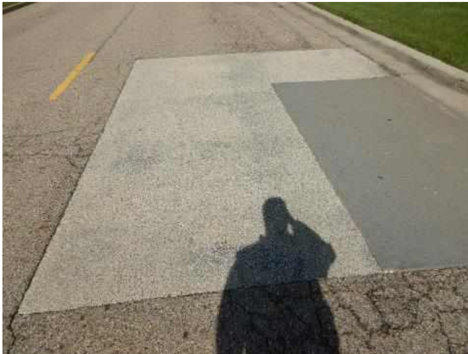
HAZELWDD-E00C-Patching-(Sample Unit No. 02)
