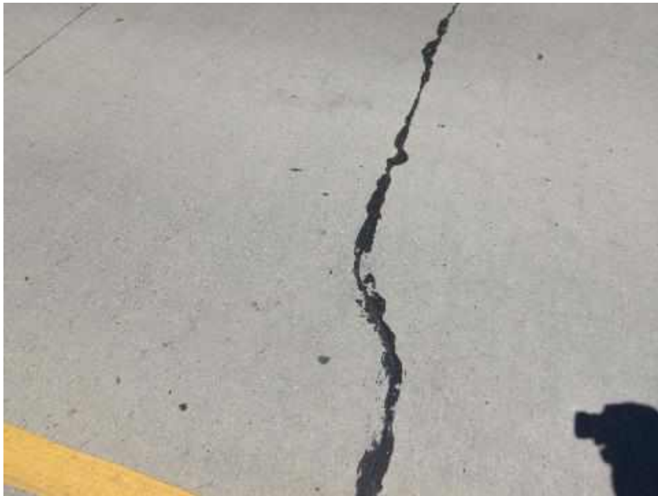
GREGYD-E02A-LTD Cracking-(Sample Unit No. 01)
