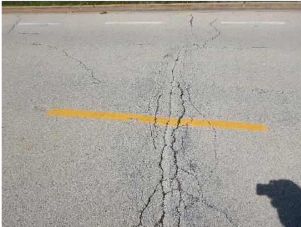
OAKS-S20B-L&T Cracking-(Sample Unit No. 01)
