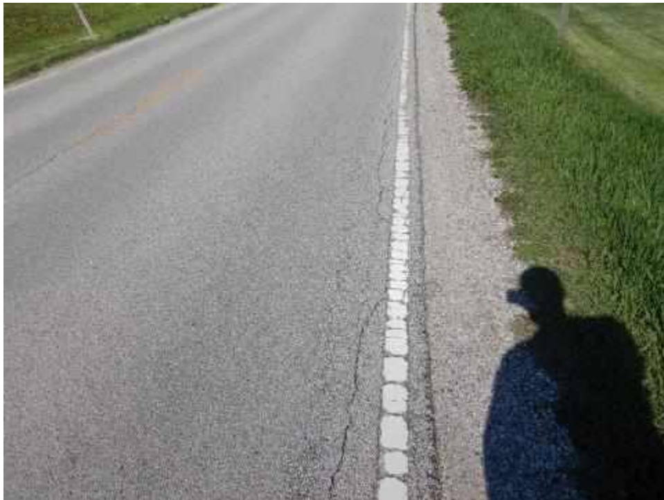
STMARR-UW12-Edge Cracking-(Sample Unit No. 01)
