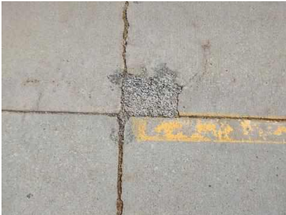
STADMD-E00D-Small Patching-(Sample Unit No. 02)
