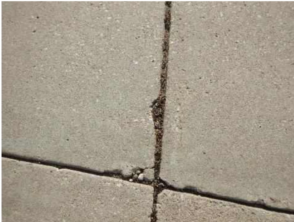
GRIFFITHD-S22B-Joint Seal Damage-(Sample Unit No. 01)
