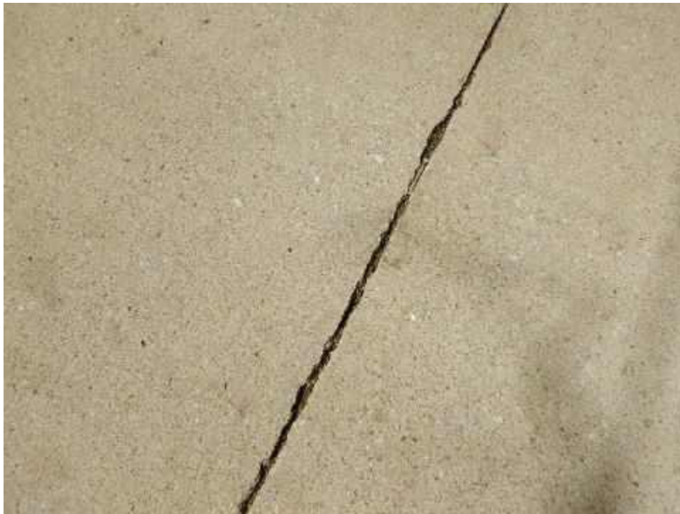
STADMD-E00E-Joint Seal Damage-(Sample Unit No. 01)
