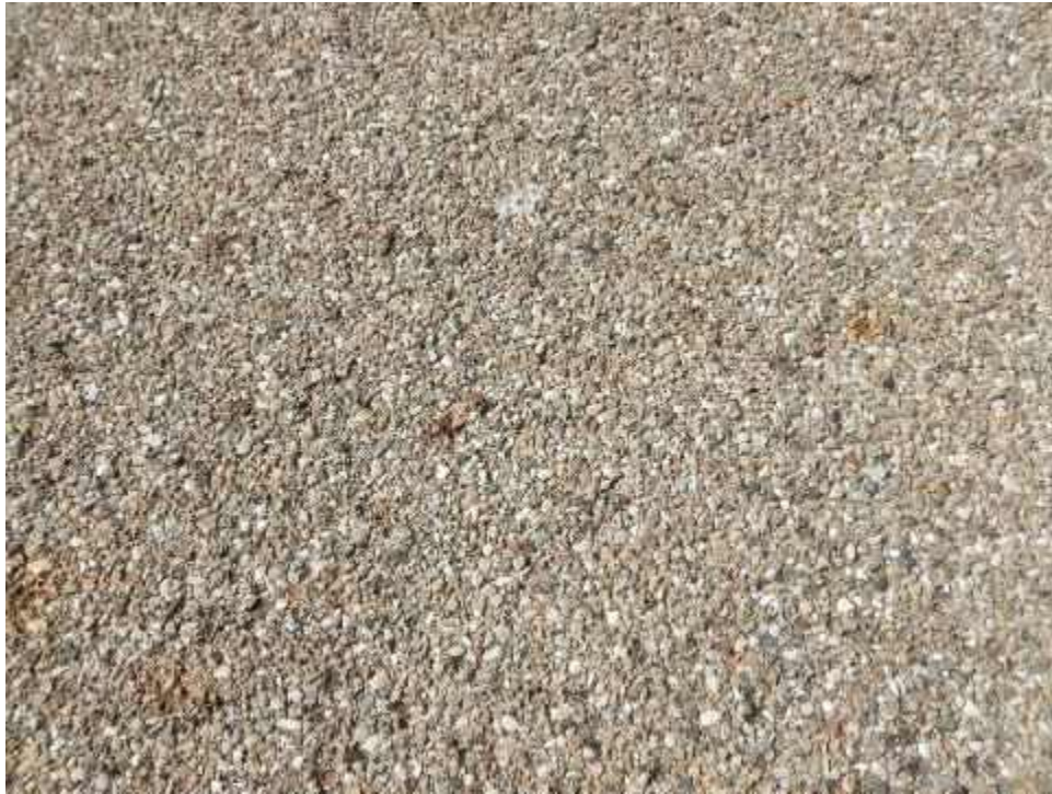
HAZELWDD-E00C-Weathering-(Sample Unit No. 01)
