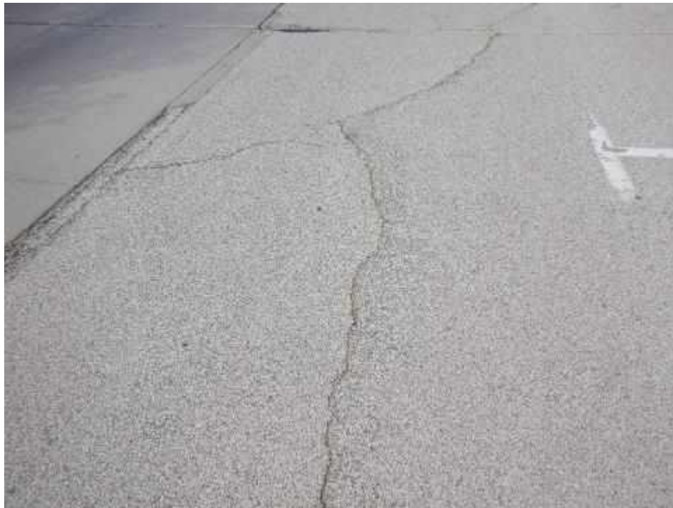
DORNRDR-US11BE-L&T Cracking-(Sample Unit No. 01)
