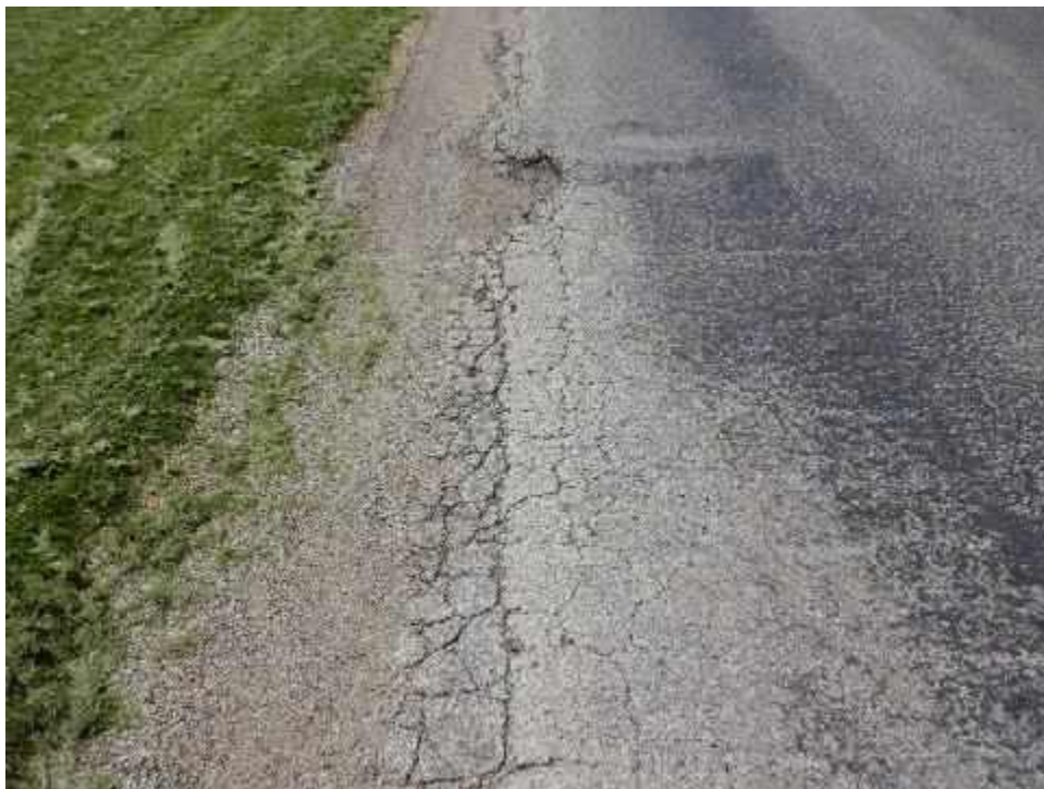
GOODWINA-US17-Edge Cracking-(Sample Unit No. 01)
