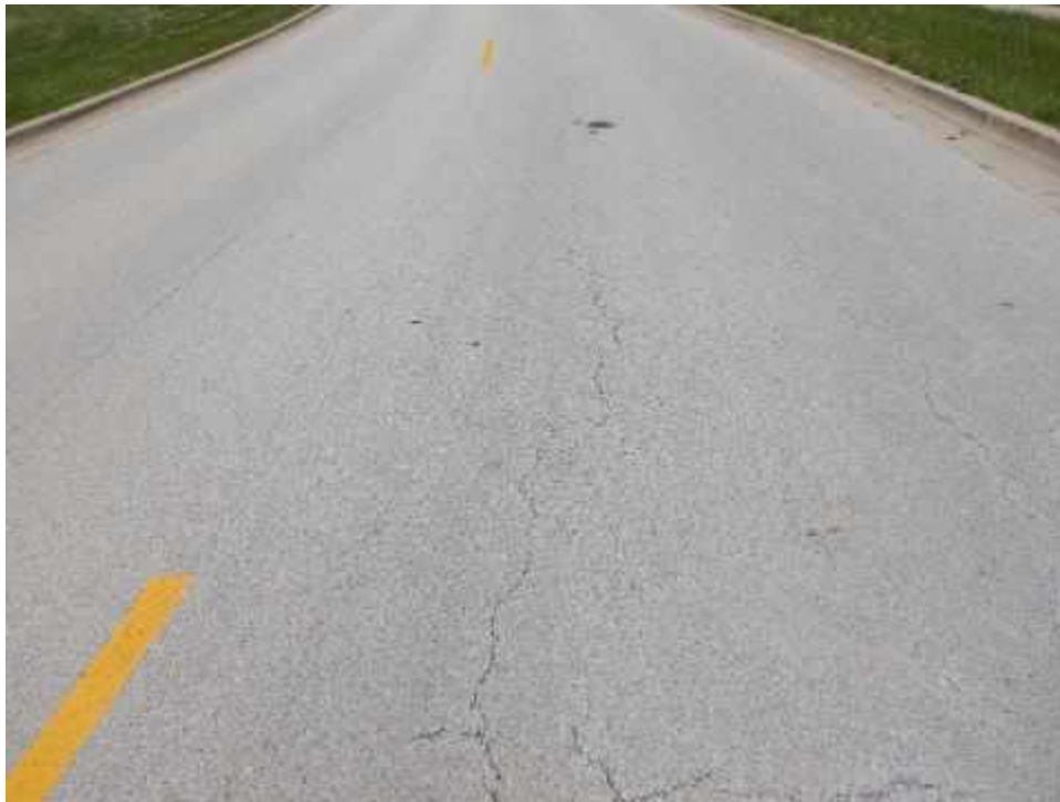
HAZELWDD-UW05-Alligator Cracking-(Sample Unit No. 01)
