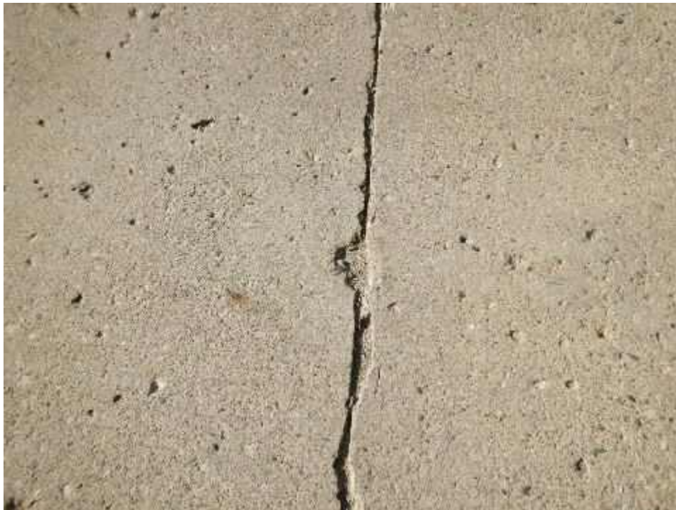
STMARR-E00B-Joint Seal Damage-(Sample Unit No. 01)
