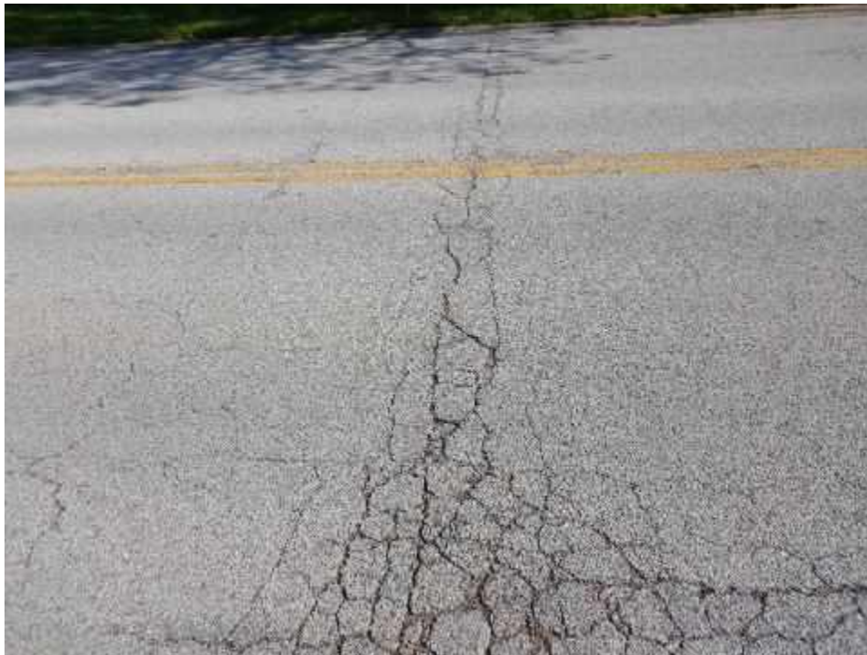
STMARR-E00D-Joint Reflection Cracking-(Sample Unit No. 01)
