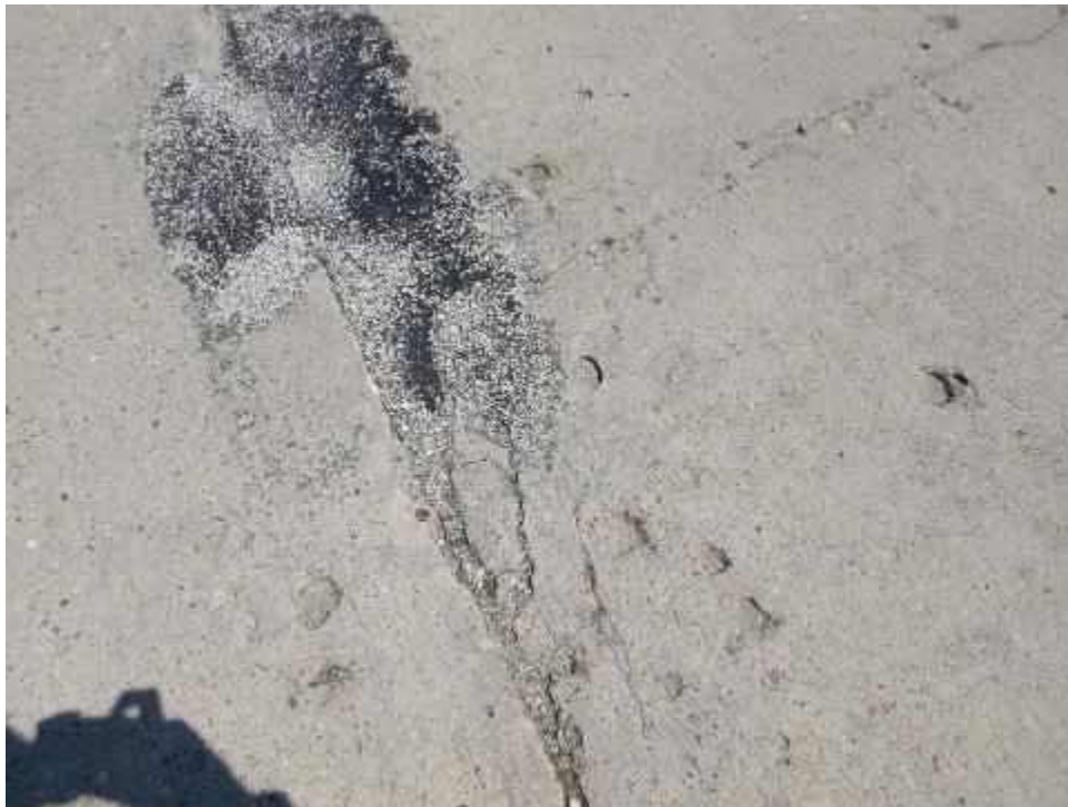
OAKS-S13-Durability Cracking-(Sample Unit No. 01)
