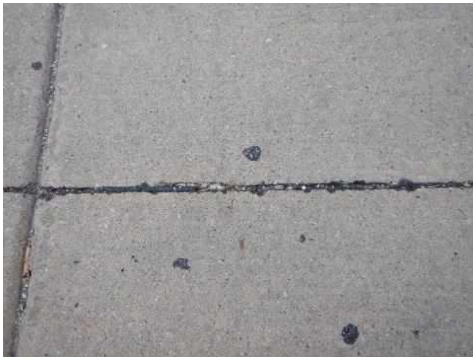
COLAGCT-UW09AN-Joint Seal Damage-(Sample Unit No. 01)
