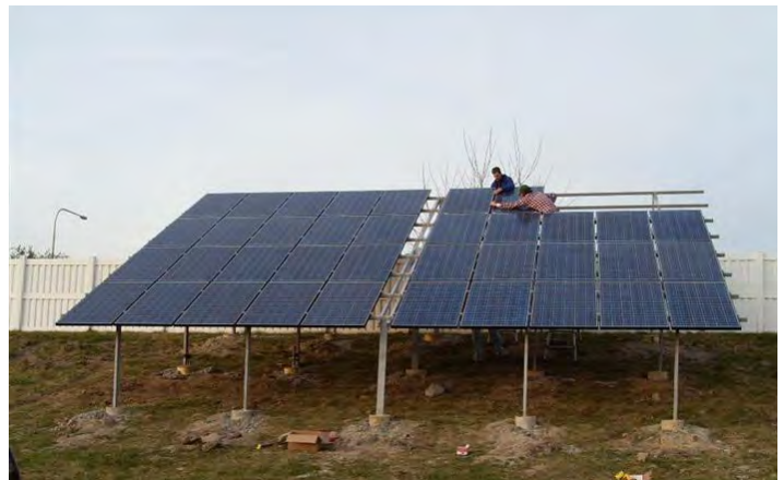
Solar PV panels in back yard.
