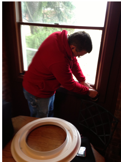
Richard Burton, Allerton Park Facilities Manager, marks leakage points for sealing
