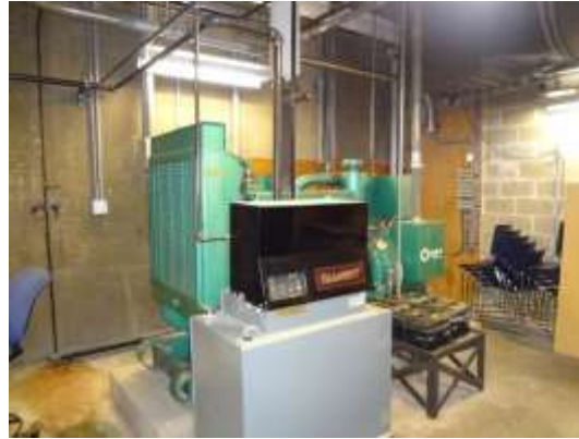
Generator and day Tank
