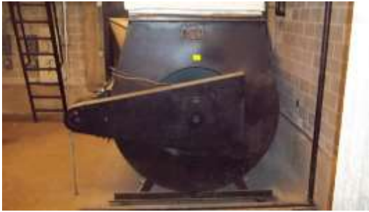
Typical supply fan
