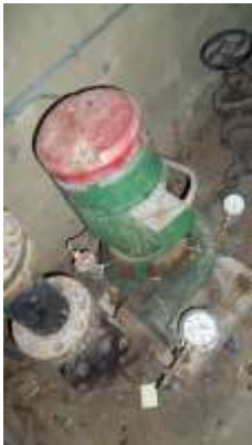
Sump pump Pic #3
