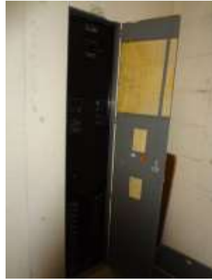
Lighting panelboard with contactor
