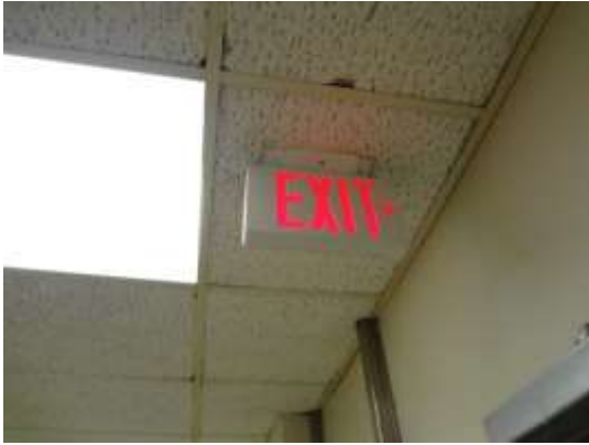
Typical exit sign
