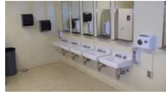
Typical bathroom sinks
