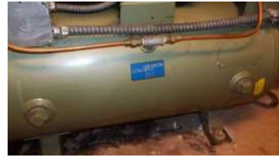
Compressor system angle #2
