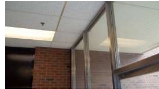
Sprinkler head near café door
