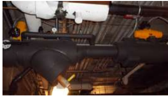
Chilled water piping
