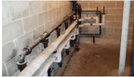
Water piping to water closets
