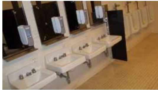
Men's bathroom fixtures
