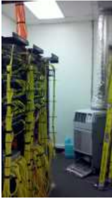
Building 99 Hub Room
