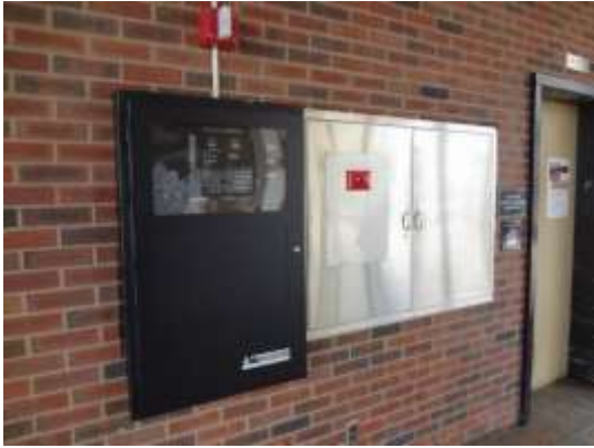
Fire alarm panel
