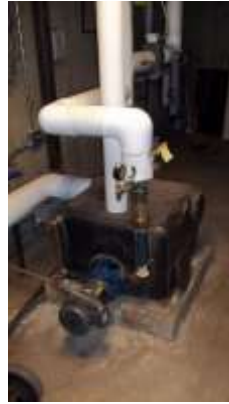
Condensate pump CP-2
