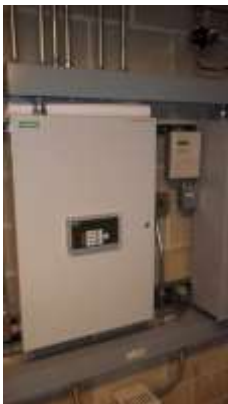
Building automation control panel
