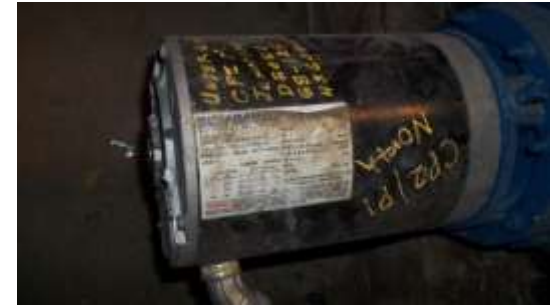
Condensate pump CP-2 motor-3HP
