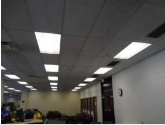
Reading area lighting
