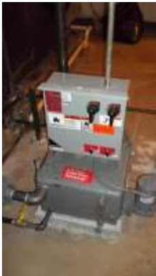
Replaced(new) condensate pump
