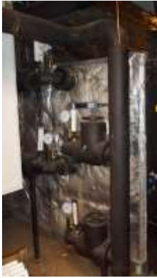
Chilled water connection to AHU unit
