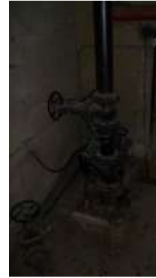
Sump pump Pic #2
