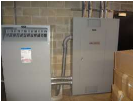
Transformer and distribution panelboard (1989)
