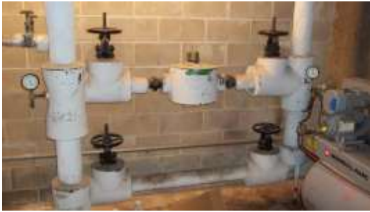
Domestic cold water piping and water meter
