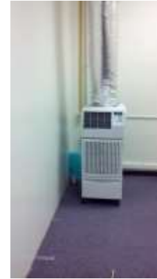
Building 99 Hub Room Cooling System
