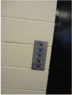
Switches for reading areas and circulation area 81
