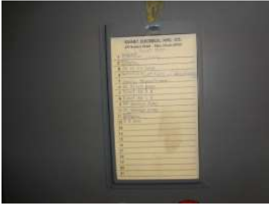
Emergency panelboard directory
