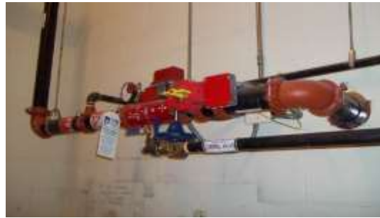
Fire protection zone with piping
