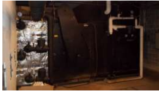
Another typical supply fan
