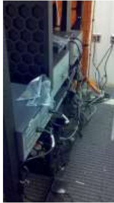
Building 99 Data Rack Receptacles
