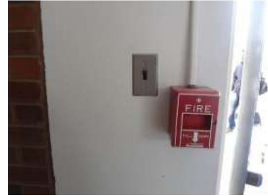
Typical pull station
