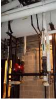
Steam to hot water heat exchanger and hot water circulating pump
