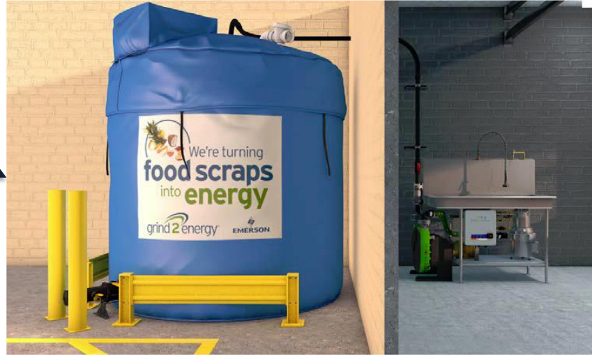
Food waste is ground into a slurry, collected in this tank in the loading dock
