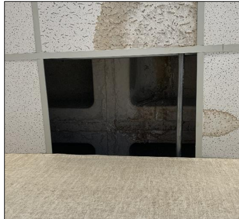
Figure 13 A hole in ceiling
