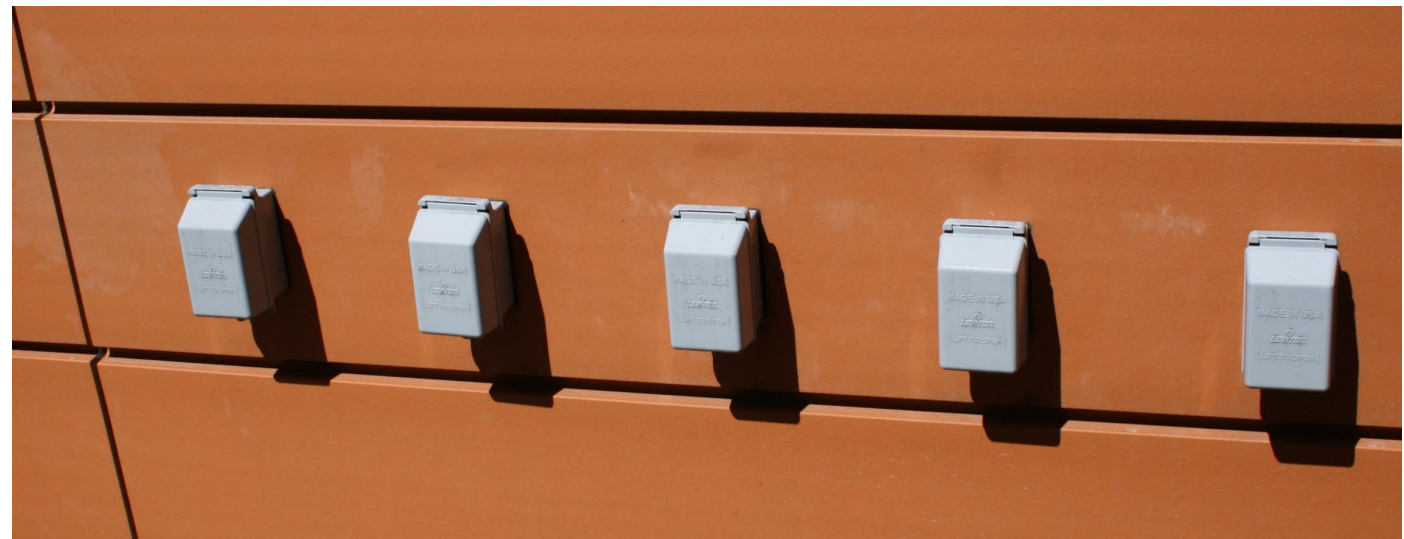
A few outdoor outlets on ECEB.
