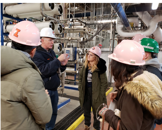
Abbott Power Plant Research and Engagement Support
