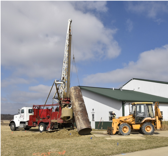
Underground Thermal Battery Test System
