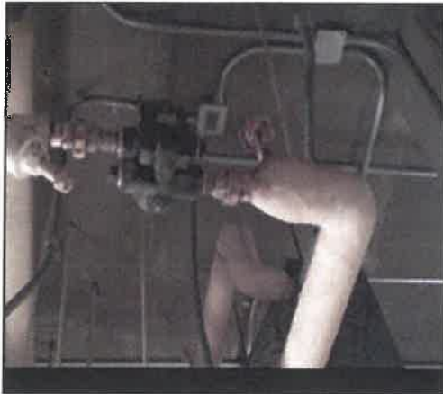
Existing Steam Trap
