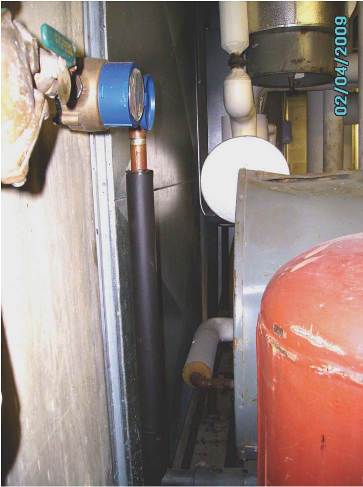
Photo 1: Steam generator close to blanked-off louver. See sketch in Appx. B.
