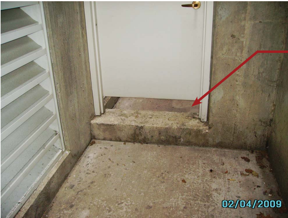
Photo 3: Gap under door to be filled.
