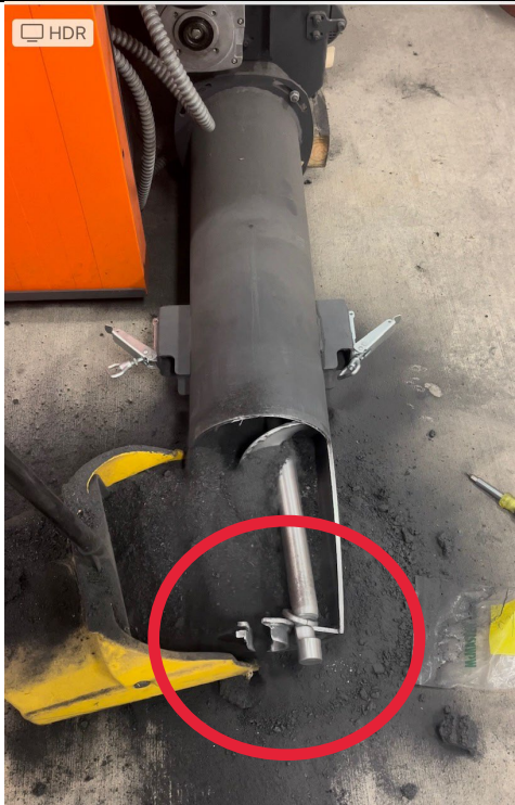
Modified auger design with failed bearings
