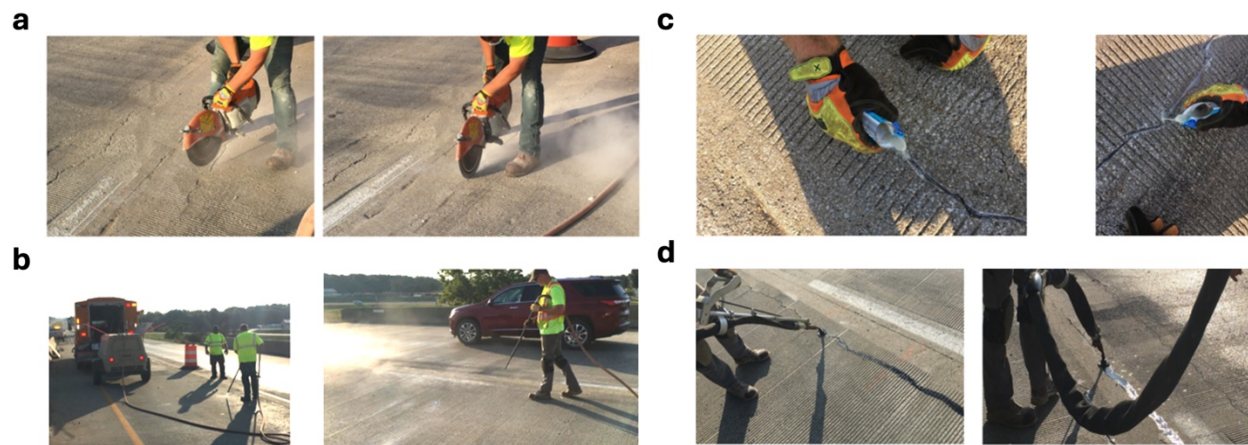
Figure 8: Repair methods for extensive cracking on concrete overlays/pavements. (a) Cracks are widened using saw-cut equipment. (b) Compressed air is used to clean debris from the cracks. (c) Two-part epoxy sealant is manually applied to the cleaned cracks. (d) CRAFCO rubber is melted and applied to the cracks, providing a faster and cheaper solution suitable for wider cracks and colder conditions, although it requires annual reapplication due to its shorter lifespan compared to epoxy.
