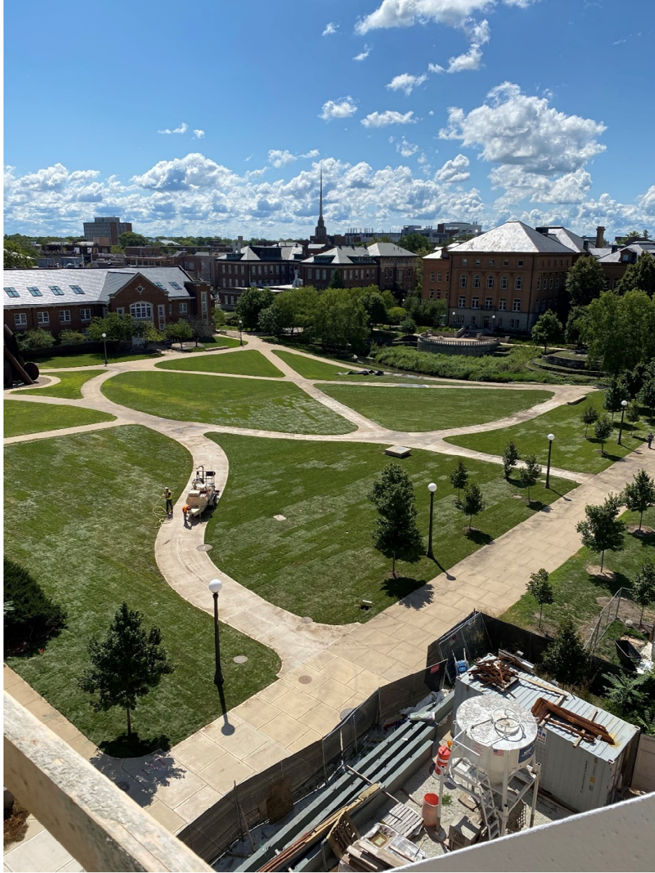
Geothermal well field in late August, 2021
